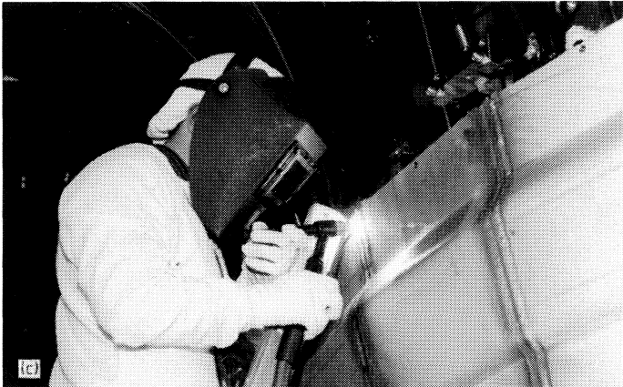
15 Semi-automatic TIG welding: a) Equipment for automatic feeding of the filler wire; b) Vacuum vessel of the Joint European Torus (JET) ; c) Manual TIG welding of the stainless steel inner lining of the toroid vessel (b and c courtesy of the JET Joint Undertaking).
