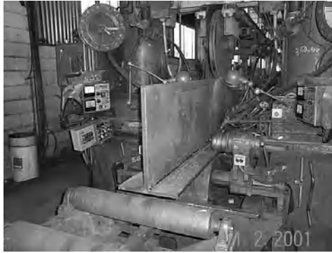
Figure 10.4. Construction of an I section on a vertical bench – photograph from Baudin-Châteauneuf
