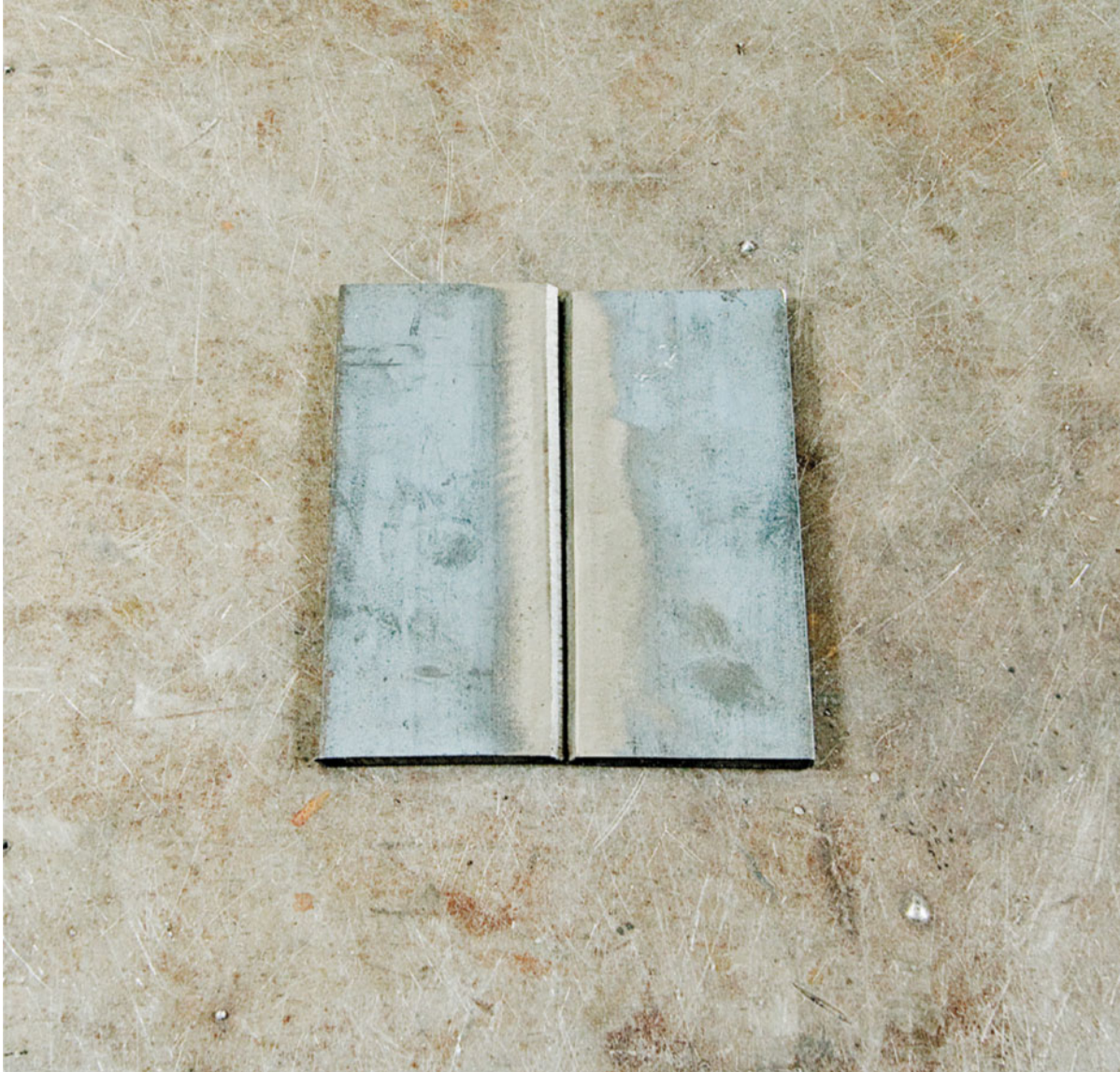
When you are done chamfering, prep the weld zone by grinding and cleaning the steel close to the weld.
