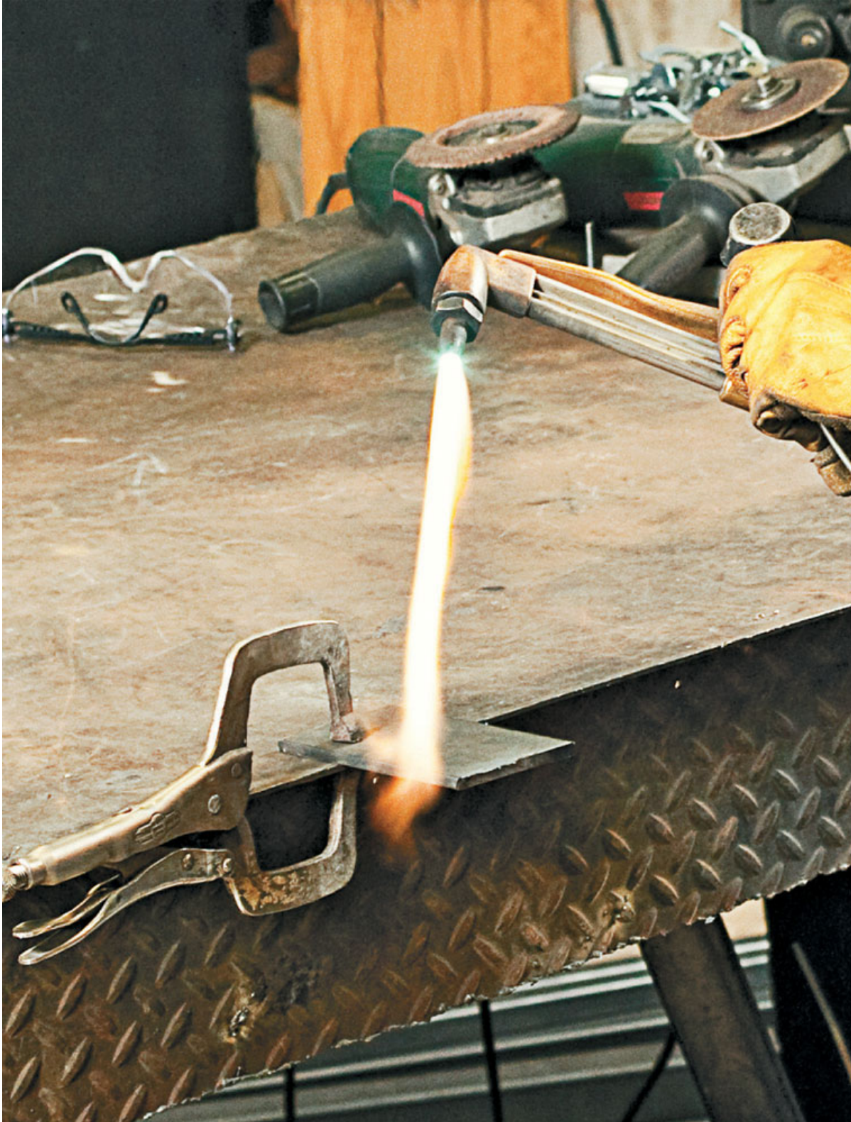
Ignite the acetylene gas first by opening the valve a little and using the striker. Once ignited, slowly add oxygen until you have the proper flame for cutting.
