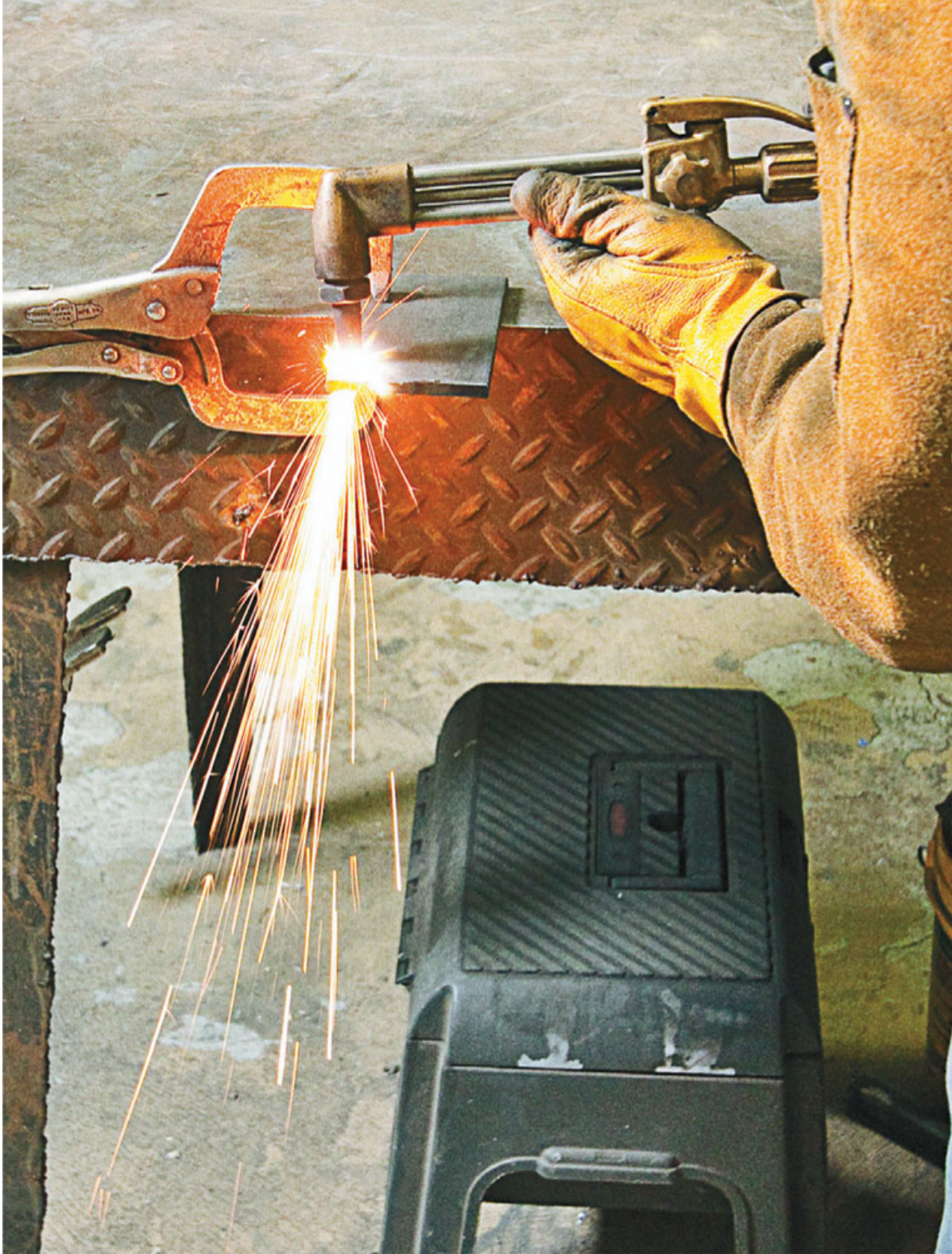
Wait for the steel to become a cherry color before starting the cut.
