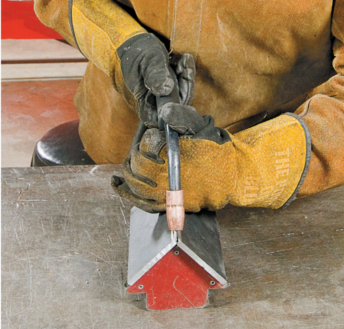
Start tacking by putting the wire down at the bottom of the joint.
