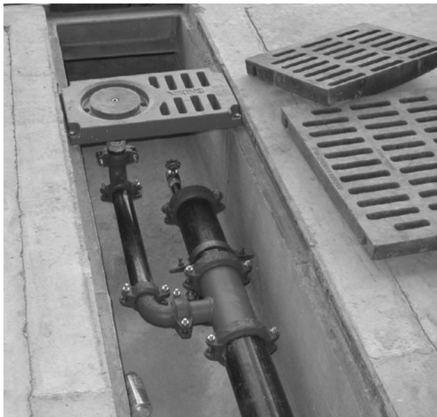
Fig. 4-6 A Viking in-floor sprinkler head and piping under floor grate
