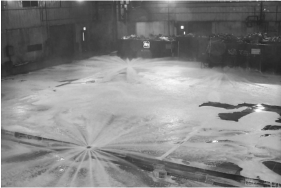
Fig. 4-7 An in-floor sprinkler head in operation
