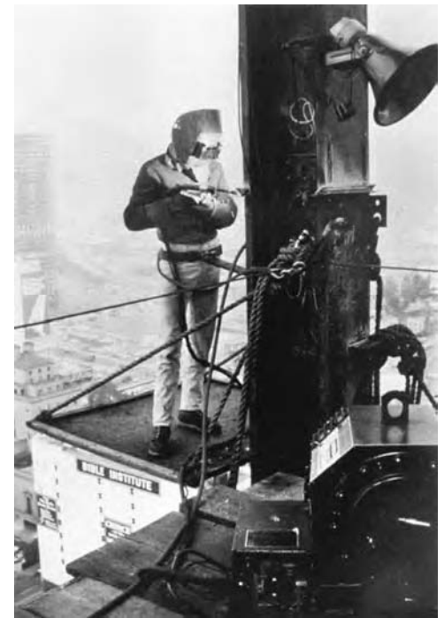
Fig. 13 Splicing a column during the erection of a building in Los Angeles using the semiautomatic self-shielded, flux cored arc welding process
