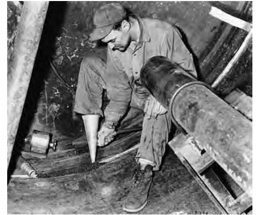
Fig. 12 Four submerged arc passes are made inside the tower of this flame-gouged seam joining the head to the shell. A current of 400 A and a speed of 36 cm/min (14 in./min) were used.
