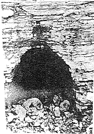
sed drawpoint photographed in the trough after it had been drawn empty. This drawpoint is unreinforced and has had very well. Note the is of wear above the brow.
