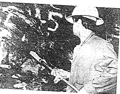
Figure 201 : The instrument, filled with activated epoxy resin, is carried to the end of the hole by means of a special tool fitted with guide wheels to centre the instrument. A mercury switch in the tool gives the orientation of the gauges and a trip wire within the cell indicates that all the cement has been extruded.
