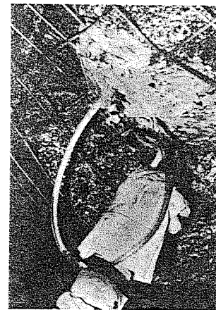
Application of rapid setting plaster to a rockbolt washer assembly to seal it for grouting.
