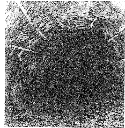
Figure 187 : Results achieved in a hard rock mining tunnel using crude smooth blasting techniques. In spite of the wide spacing of the boreholes (marked with white paint), the results are better than those obtained with normal bulk blasting.
