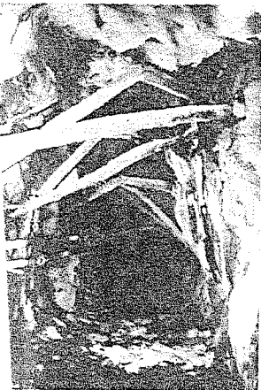
In spite of the severe deformation indicated by the buckled sets, spalling of this mine excavation has been controlled by the application of a thin concrete layer and stability is adequate for temporary access.
