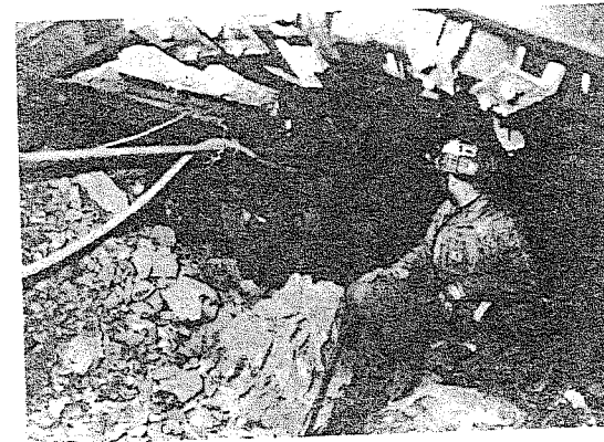
Figure 132 : Use of heavy steel sets in an attempt to control fracturing around a mine tunnel subjected to high stresses. The steel sets are too stiff for this application and cannot accommodate the deformation to which they are subjected.
