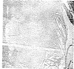
p_2/\sigma_c = 0.3 - severe sidewall spalling.
