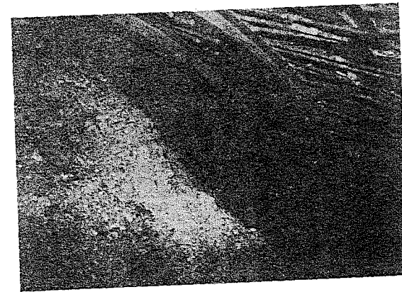
Figure 148 : Detail of figure 147 showing spiles driven between steel sets to provide an umbrella under which excavation of the face and the installation of the next set could be carried out. In this case, the fault material was soft enough for the spiles to be driven in by means of a heavy hand-held hammer.
