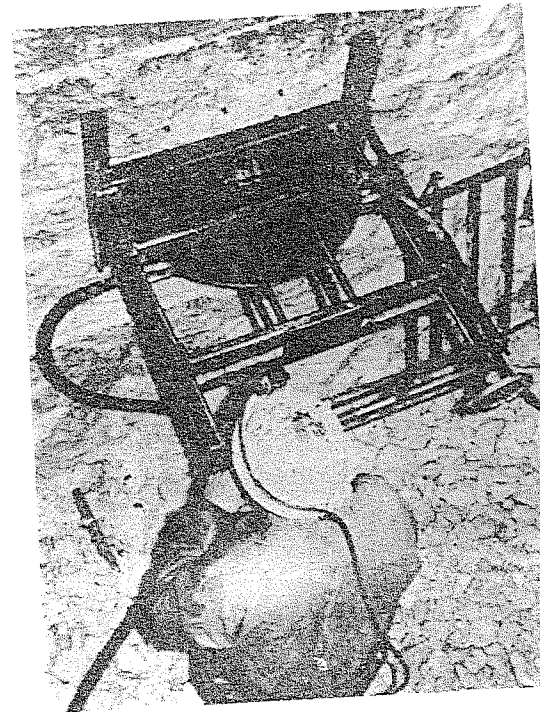
Figure 194 : Cutting a semi-circular slot in a rock face by means of a diamond blade driven by a hydraulic motor. Photograph reproduced with permission of Pierre Londe of Coyne et Bellier, Paris.
