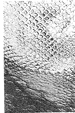
Chainlink mesh is not recommended for the reinforcement of shotcrete.
