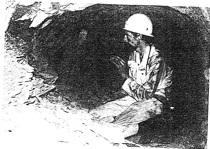
Figure 112 : Sidewall failure in a mine tunnel in very highly stressed rock in a mine in Zambia.
