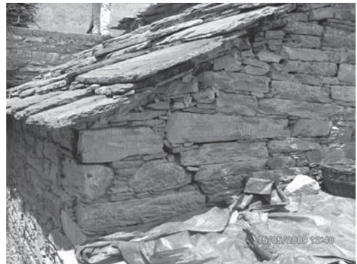
Figure 6. Crack in the stone clay structures due to differential settlement.
