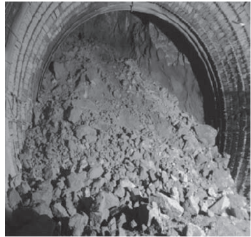
Figure 2. Loose fall from left SPL to crown.
