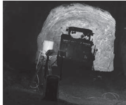
Figure 1. Laser scanning the wall of a tunnel (here the Callidus unit). Lighting is used for photographs and is not needed for acquiring the point cloud data alone.
