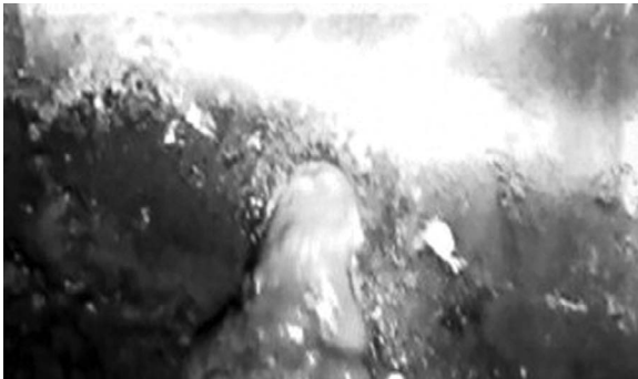
Figure 1.17 Sand and water flowing through an opened grout plug in an old cast iron lining.
