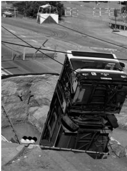
Figure 1.16 Collapse of the Munich Metro ( Construction Today , 1994).
