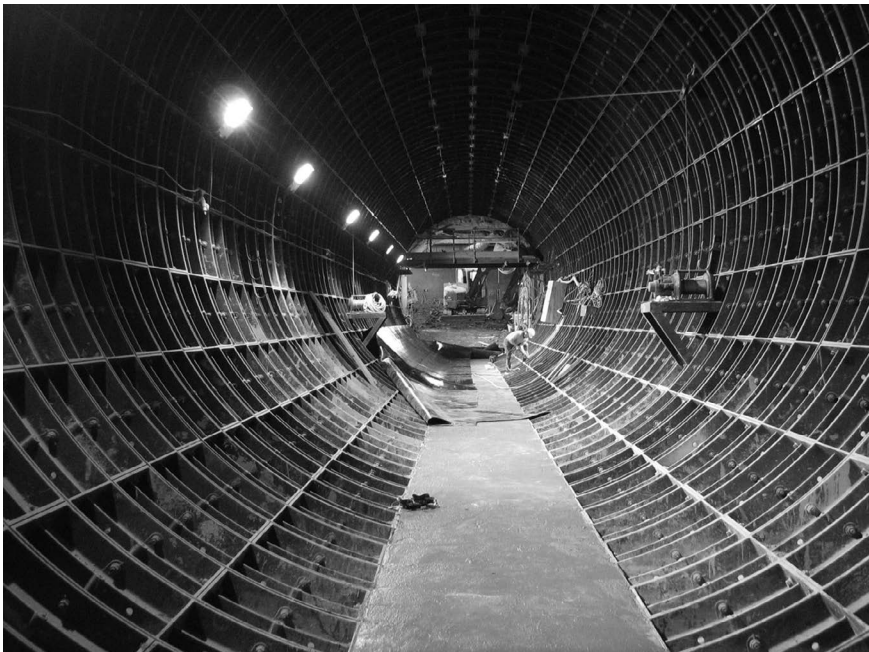
Figure 8.5 Cast iron rings in the Piccadilly Line Access passageway at King's Cross under construction.
