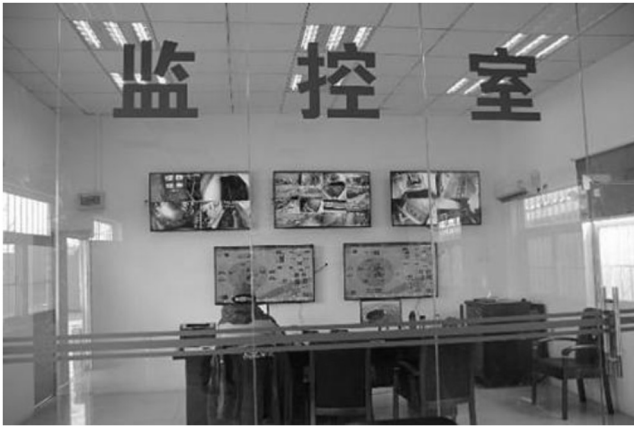
Figure 3.28 Remote monitoring center on the ground surface.
