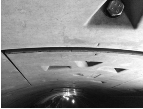
Figure 12.1 Uneven circumferential joint of shield tunnel lining.
