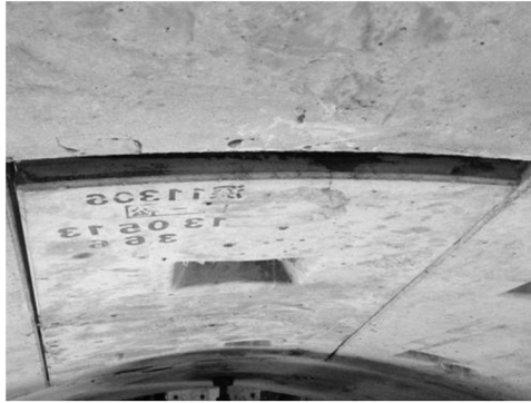
Figure 12.2 Uneven longitudinal joint of segment tunnel lining.
