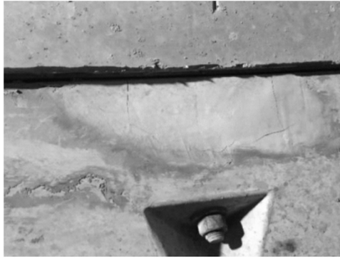
Figure 12.7 Segment dislocation and local cracking of a metro shield tunnel.
