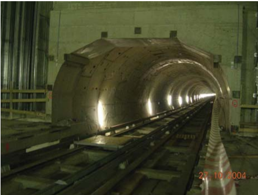
Figure an.4.2 Metro Torino Line I. The connection between a station and the tunnel.
