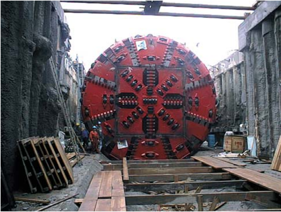
Figure 1.3 One of the Earth Pressure Balance Shields operating in the Porto Metro; the 8.7-m - diameter Herrenknecht TBM.
