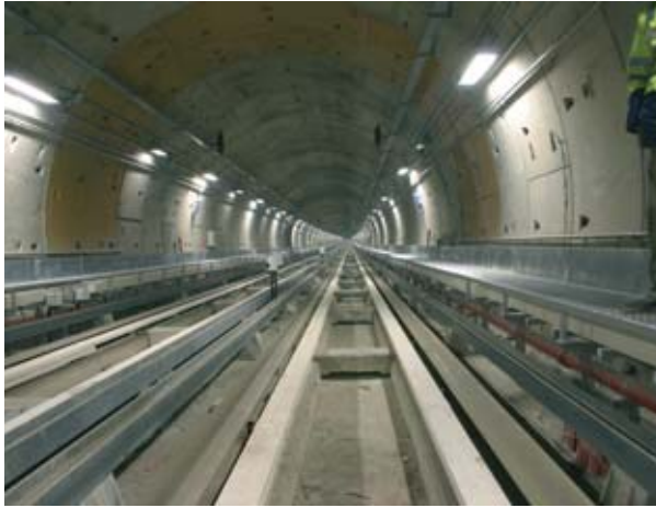
Figure 8.30 TBM-bored tunnels of Turin Metro supported by the segmental lining.
