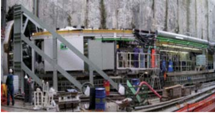
Figure ap.7.11.5 The TBM back-up.
