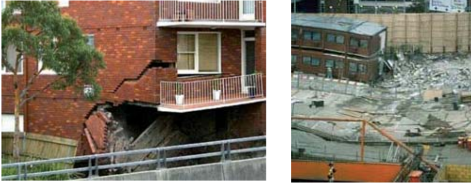
Figure 3.10 Damage to existing structures during tunnel excavation in an urban area (Left: Lane Cove Tunnel, Sydney; Right: Heathrow Express, London).
