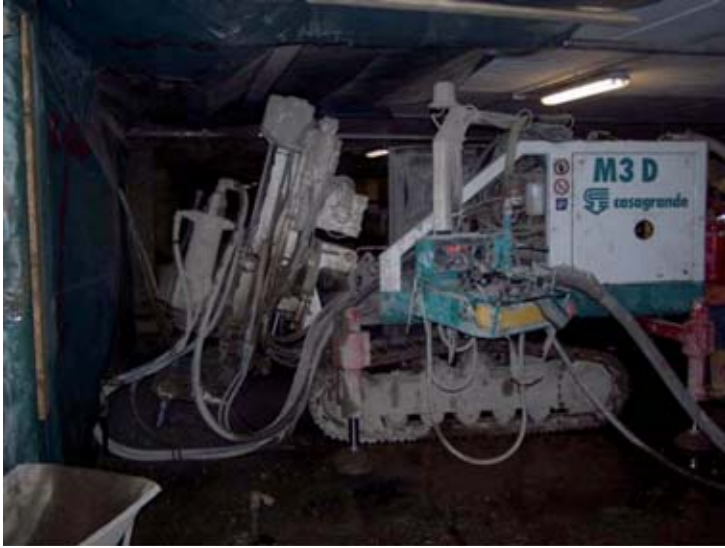
Figure 3.7 Ground treatment through grouting to allow a TBM to pass under an underground car park during the construction of a Metro Line.
