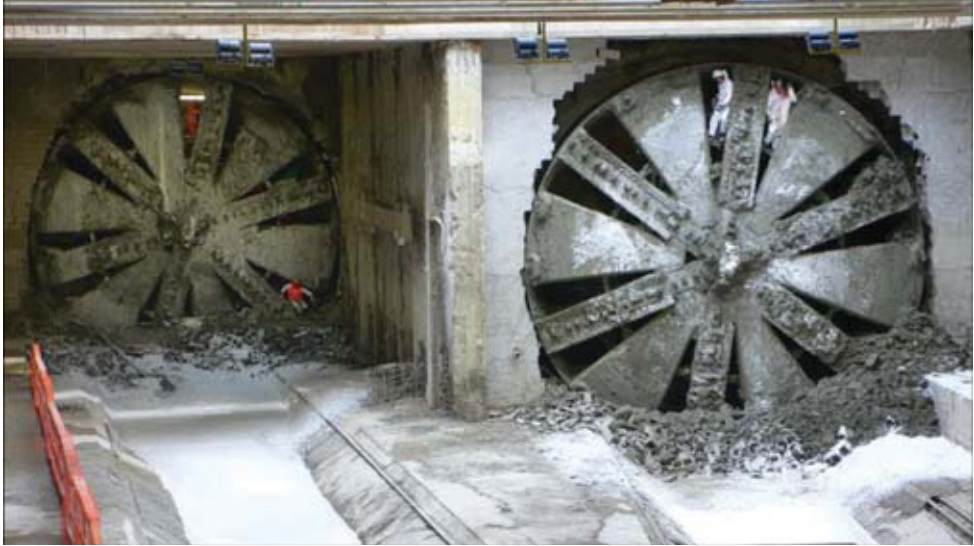
Figure an.3.1 Nodo di Bologna: the final breakthrough of the two TBMs.
