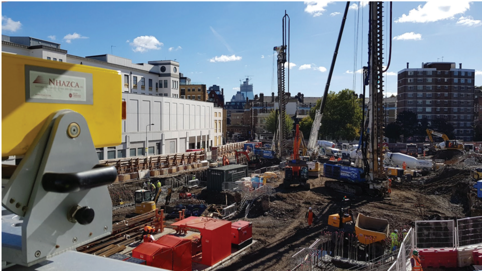
Figure 11.8 Terrestrial interferometer installed (Mazzanti et al., 2020).
