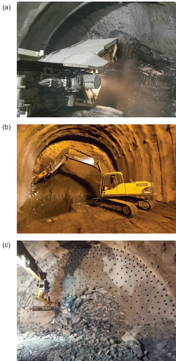
Figure 8.4 Photographs of some conventional excavation methods using machines. (a) Roadheader working in an argilloschist formation; (b) high-energy impact hammer working in a tuff tunnel face; (c) drill and split method in a hard gneiss tunnel face. (Courtesy of Italferr S.p.A. and AK.)
