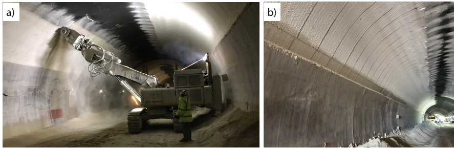
Figure 12.6 Mechanical milling of the internal lining concrete aimed at re-lining the tunnel. (Courtesy of CIPA SpA.)
