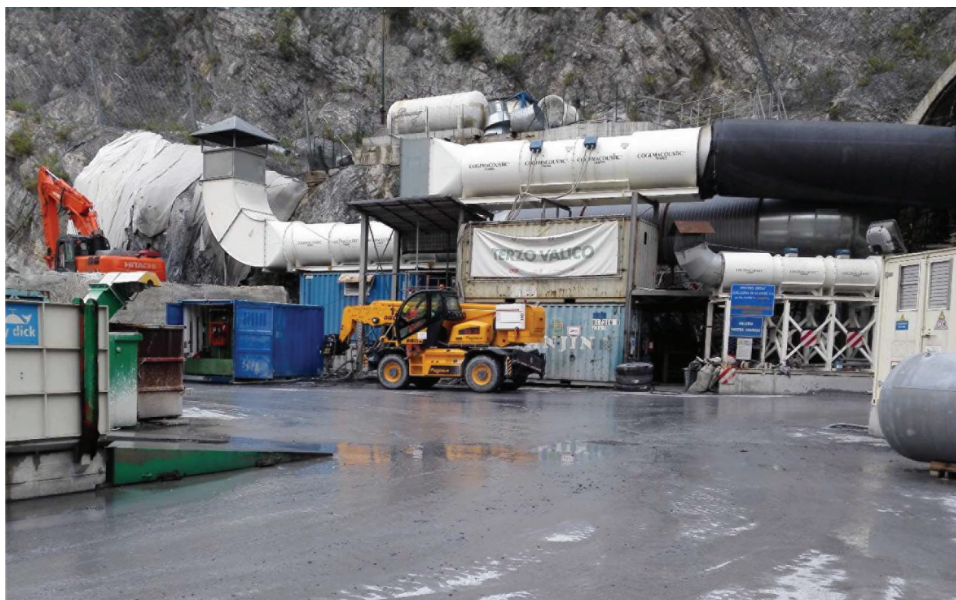
Figure 5.6 Example of fan system and filters in the case of the Cravasco tunnel of the Terzo Valico dei Giovi (Italy). (Courtesy of Italferr.)
