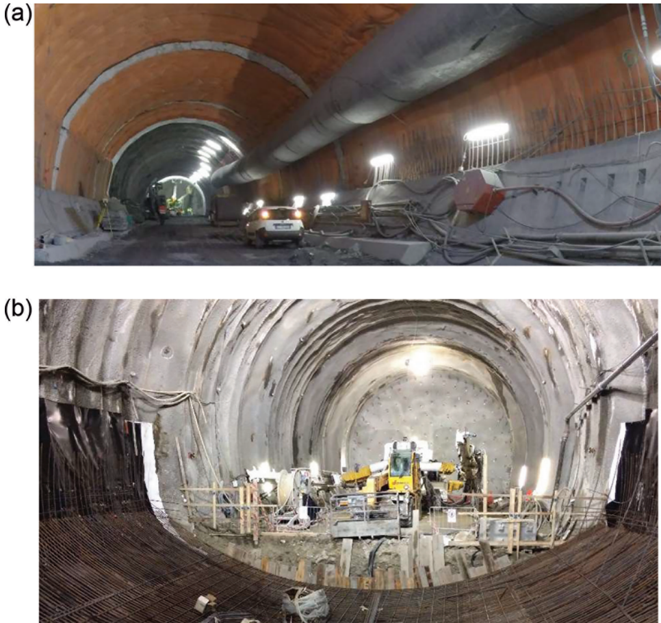
Figure 8.20 Example of a conventional tunnel where there is a large (a) distance between the final lining and the tunnel face (courtesy of Mapei S.p.A.) and (b) where the invert is cast very close to the tunnel face. (Courtesy of Italferr S.p.A.)
