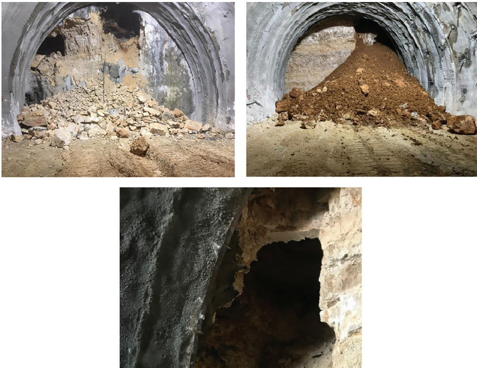
Figure 3.19 Example of karst phenomena intercepted during the excavation. (Courtesy of E.M. Pizzarotti.)
