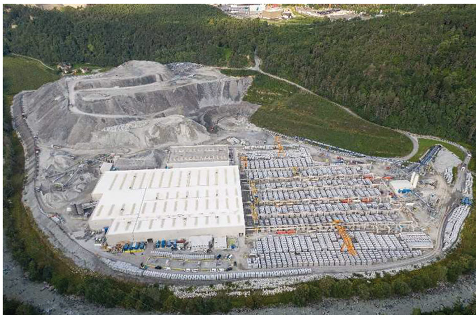
Figure 5.3 Hinterrigger site plan view; area for the spoil management of Brenner Base Tunnel, Italian side. Part of the excavated is used in the concrete for the production of the segment lining. (Courtesy of BBT.)
