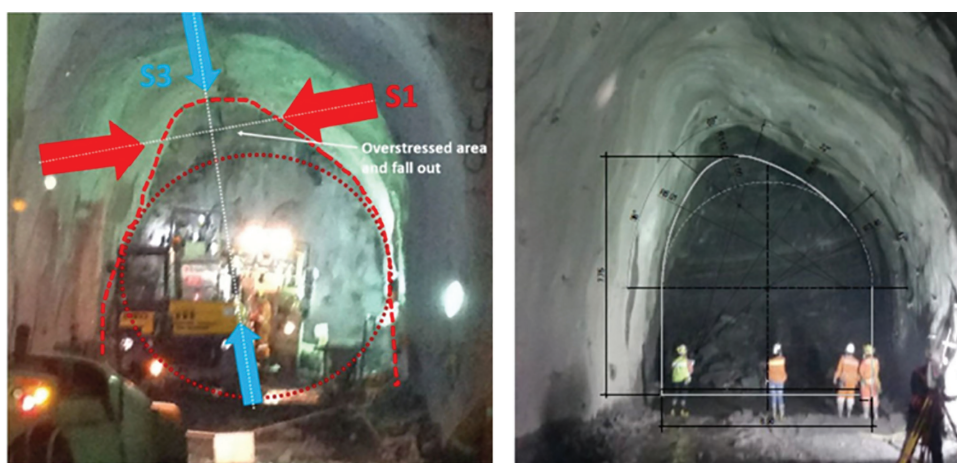
Figure 7.6 Example of large overbreak resulting from overstressed zone in the crown of an adit tunnel for hydroelectric plant in Andean region (Russo, 2019).
