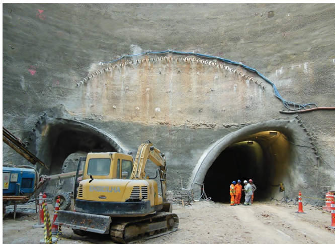
Figure 8.7 Example of Chakara Klabin Station in Sao Paulo (over 350 m 2 ) constructed with partial excavation with side drifts and systematic pre-support in a poor rock mass and soil, below water table at low overburden. (Courtesy of Geodata S.p.A.)
