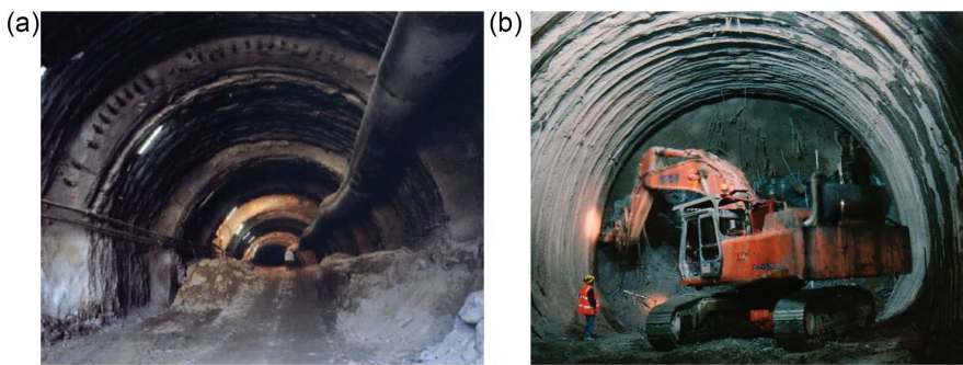
Figure 8.6 Photographs of an excavation with head and bench excavation and use of steel pipe umbrella arch as pre-support in a moraine and a full-face excavation with face reinforcing.
