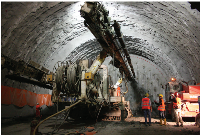
Figure 8.22 Frontal view of the steel pipe umbrella and reinforcements installation. ‘Tunnel of Cavallo’ on high speedway A 14. (Courtesy of Trevi S.p.A.)
