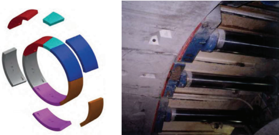
Figure 8.21 View of a tunnel made of segments and detail of the machine jacks acting against the already installed ring.
