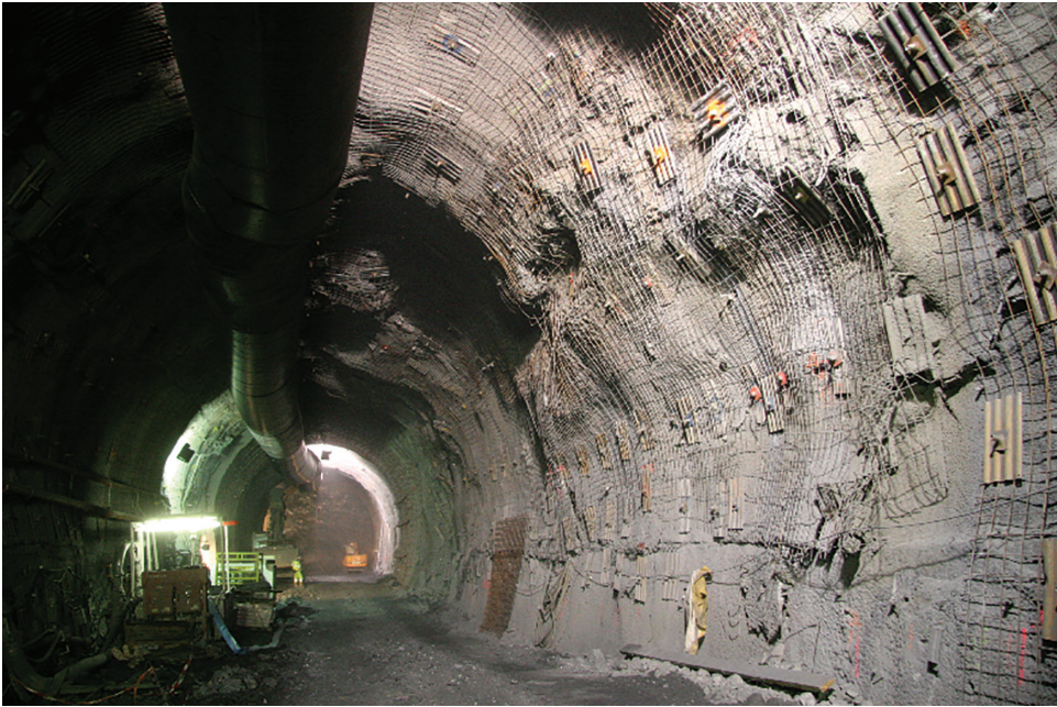
Figure 3.15 Example of squeezing behaviour in the S. Martin La Porte exploratory adit of the Lyon–Turin Railway Base Tunnel.
