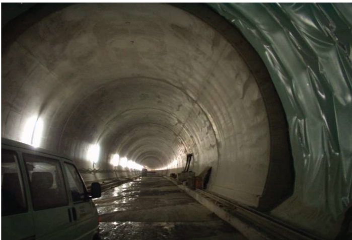
Figure 8.19 Example of the lining cast in place and of the waterproofing layer.
