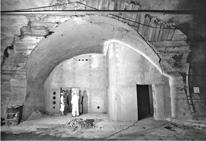
Figure 7.9 The refurbishment of the refuges in the Mont Blanc Tunnel (Photograph courtesy of Morgan Thermal Ceramics)
