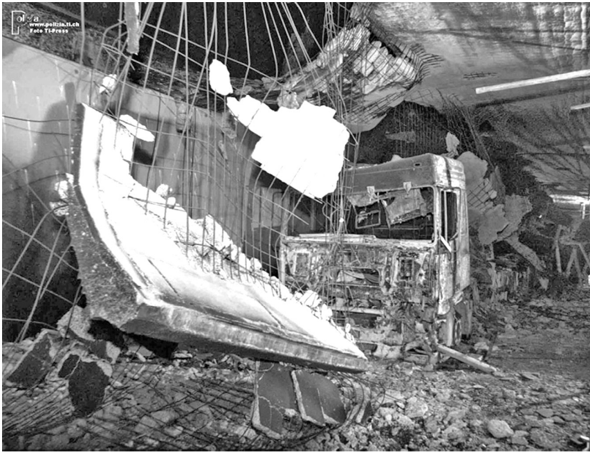
Figure 21.1 Damage to the tunnel and vehicles following a tunnel fire © Ti-Press/Polizia Cantonale
