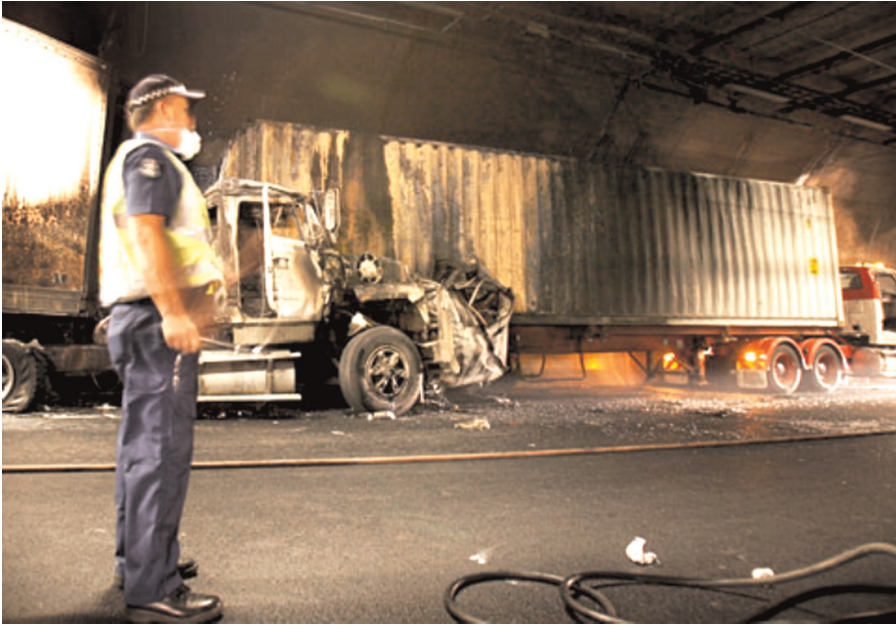
Figure 4.3 Burnley Tunnel after the fire. The road surface, tunnel walls and tunnel services are still intact
