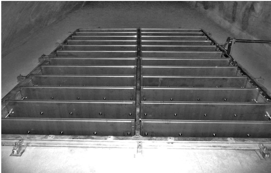
Figure 9.14 View of single point extraction damper in tunnel exhaust air duct (Katschberg Tunnel, Austria) (Reproduced by permission of Peter Sturm of the Technische Universität Graz)
