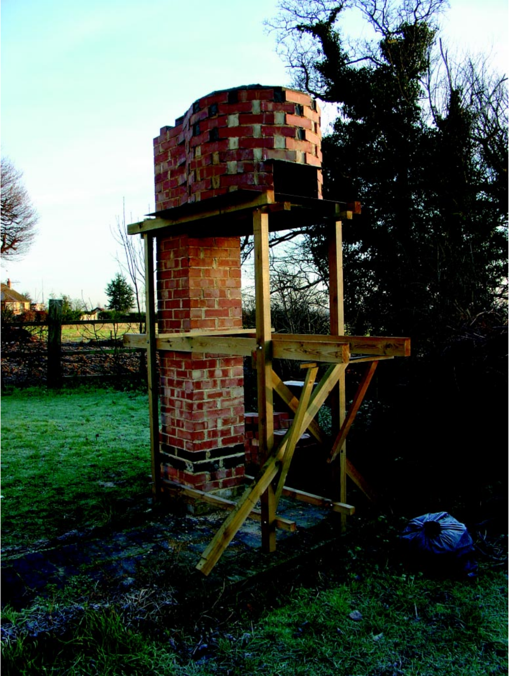
Plate 1 Full-size replica furnace, flue and displacer cylinder. The static structure supporting the cantilever portion of the masonry doubled as scaffolding during construction.
