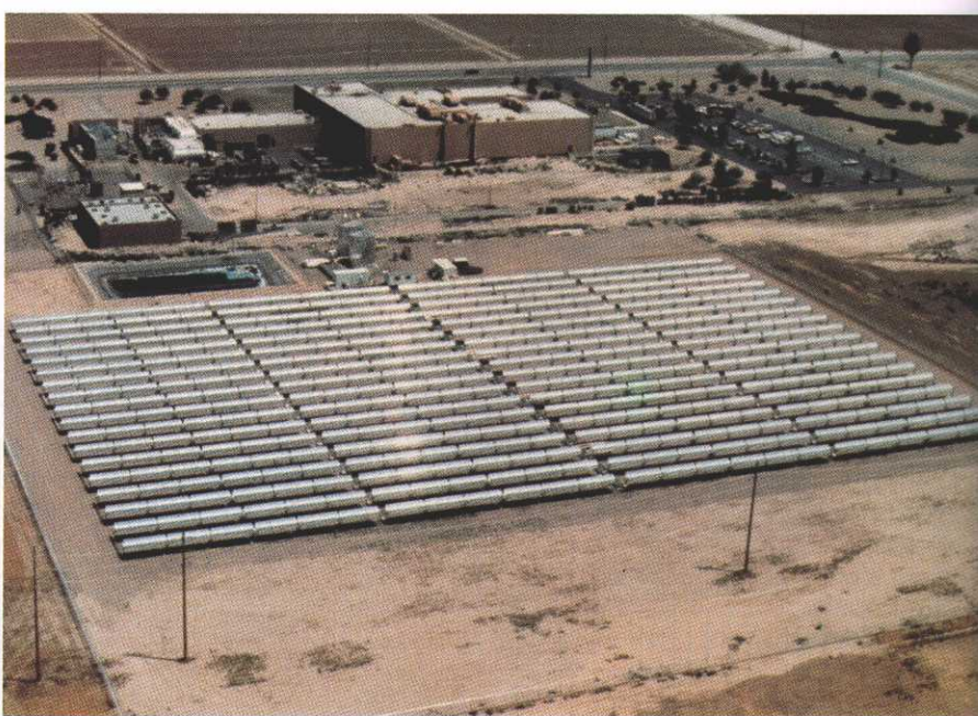
Figure 2-28. System supplying process hot water to the Gould, Inc. foil plant in Chandler, Arizona, USA (Source: SKI/ISNL)
