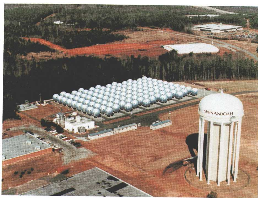
Figure 2-17. Solar Kinetics dish systems for Georgia Power Total Energy System in Shenandoah, GA, 400 kW e and 1065 kW t (Source: NREL)
