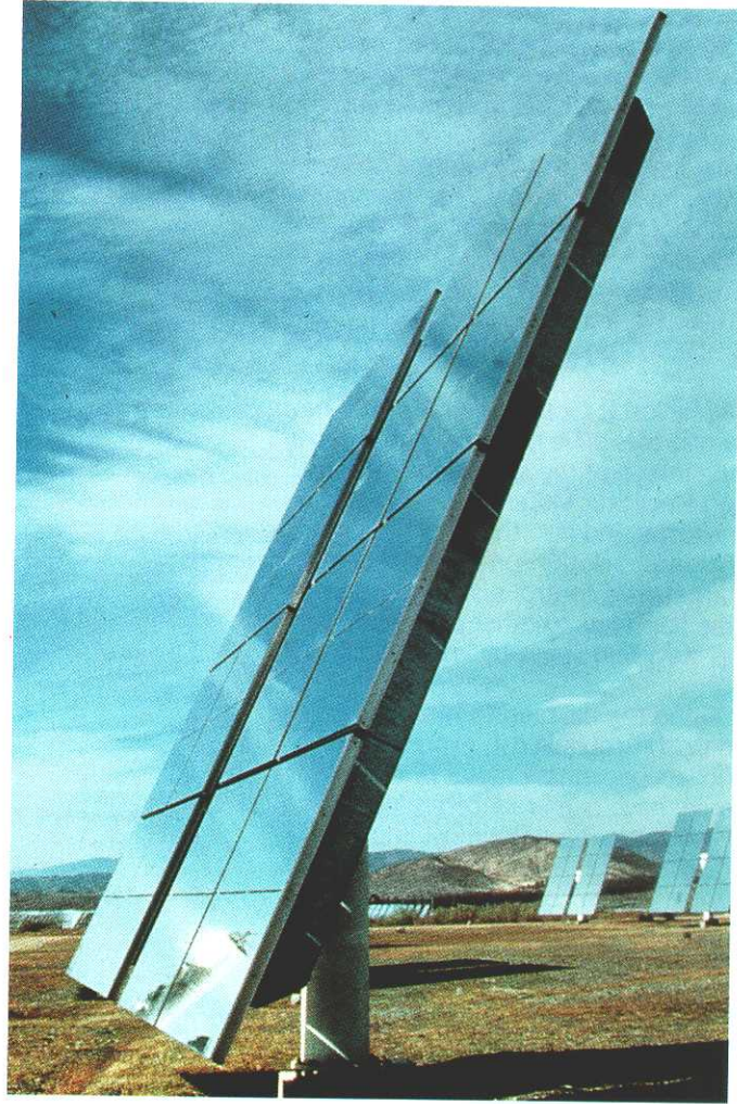
Figure 3-2. The 52-m 2 glass/metal heliostat test series units (MBB, ASINEL) of the GAST Technology Program (Germany/Spain) on the PSA; 65-m 2 GAST units (ASINEL) also on site (Source: DLR)
