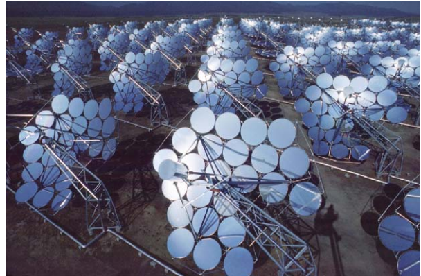
FIGURE 12 Seven hundred dishes producing steam for a central turbine system. Source: LaJet.
