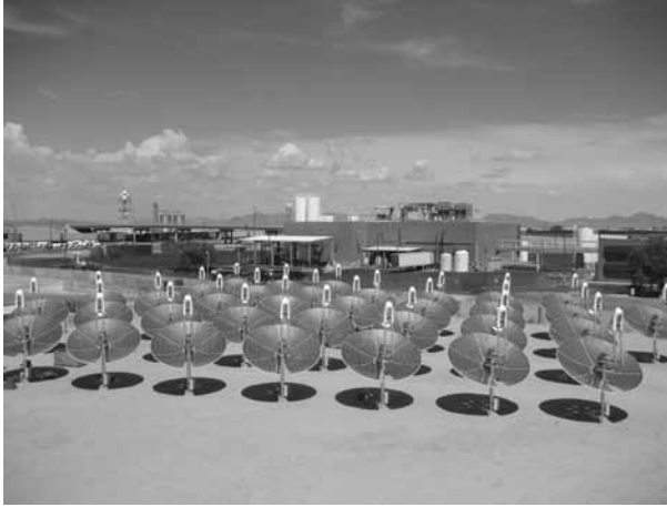
9.12 PowerDish installation in Yuma, Arizona 2010 by Infinia Corp. (Copyright: Infinia Corp.).
