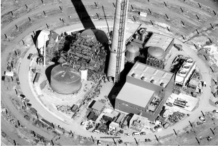
11.4 Two-tank storage system of the 17 MW el Gemasolar central receiver plant. © by Torresol Energy. Reproduced with permission from Torresol Energy, Spain.
