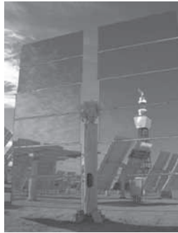
Martin Marietta Solar One and Solar Two (39.9 m 2 )
