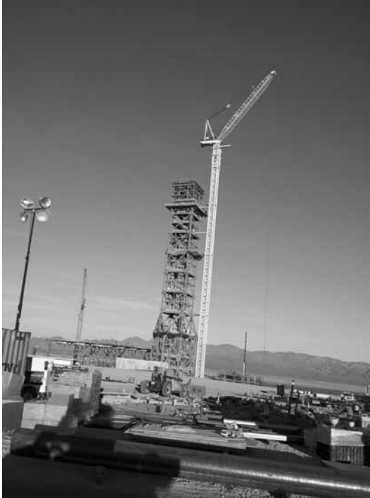
8.9 Phase 1 of 3: BrightSource Ivanpah facility near Las Vegas, January 2012. 121 m steel tower is ready for receiver installation. Over 20% of the 40,000 heliostat pedestals are installed for this 110 MW e plant and heliostat installation proceeds at 100+ per day (Michel Izygon, with permission).
