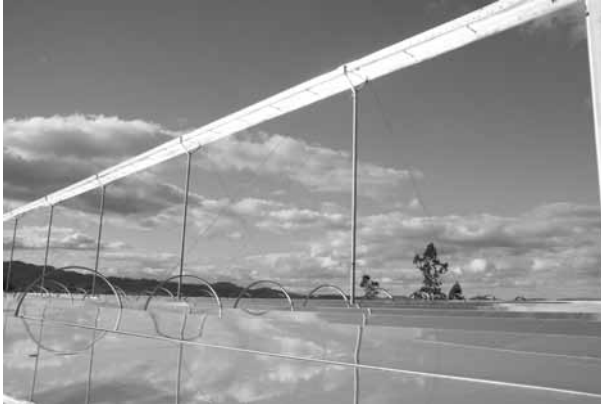
6.15 Stage 2 of the Liddell array in 2006 (copyright Areva Solar, used with permission).
