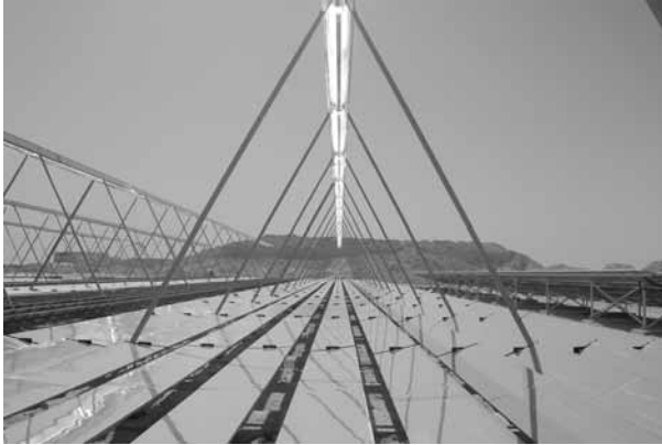
19.3 Linear Fresnel collector for a solar cooling installation in Doha, Qatar (source: Industrial Solar GmbH).
