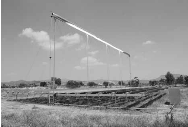
6.24 The 2005 Novatec demonstration module in the south of Spain (courtesy Novatec Solar GmbH).
