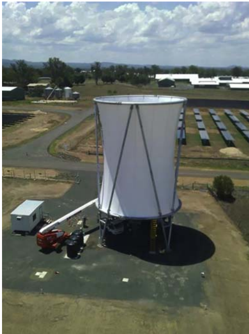
Figure 9.34 Configuration of Gatton cooling tower.
