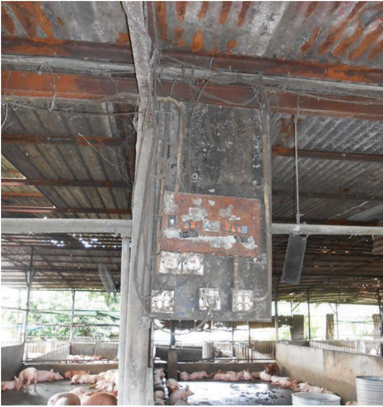
Fig. 1.4ii. Electrical box for wires and fuses in an open area of the pig farm.
