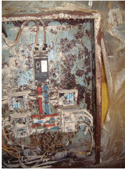
Fig. 1.2ii. Damaged farm-building electrical system.
