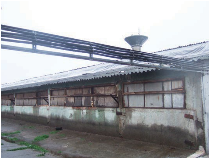
Fig. 7.5i. Older closed and dusty buildings with poor ventilation.
