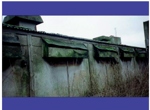
Fig 2.24 – The condition of external vents should be checked. (Courtesy of D. Chennells.)
