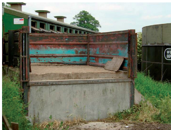
Fig 2.9 – Loading areas should be sited at the perimeter fence. (From Pritchard et al. (2005). with permission.)
