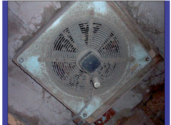
Fig 2.23 – Fans should be kept clean. (Courtesy of D. Chennells.)
