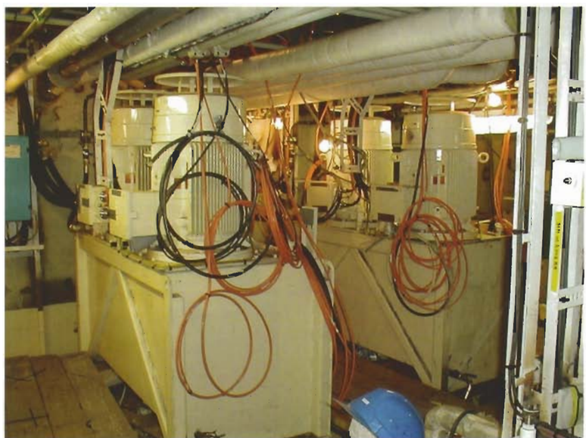
Electric driven pumps
