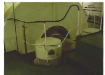
Main engine flywheel with intermediate shaft and main lubricating-oil pumps, electric motors
