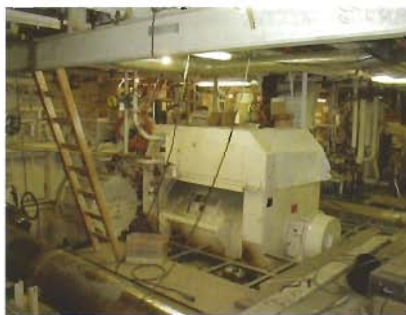
Main-engine driven generator
