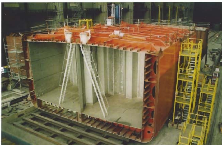
Another view of the same tank
