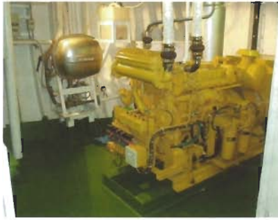
Fresh water generator
