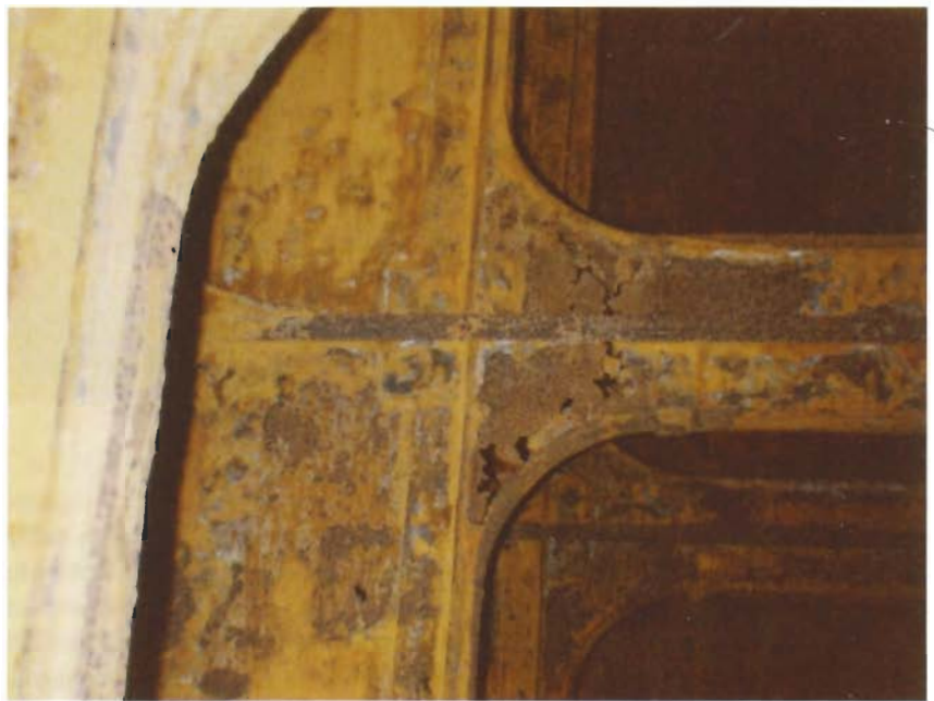
Corrosion in a ballast tank of a tanker
