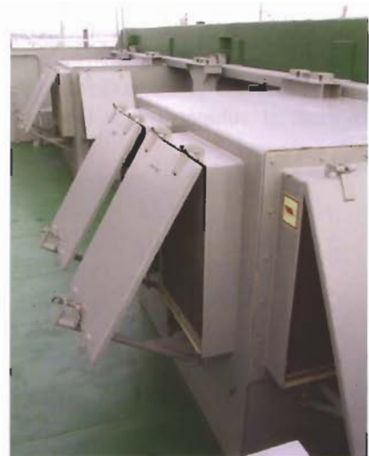
Ventilation grill with cover
