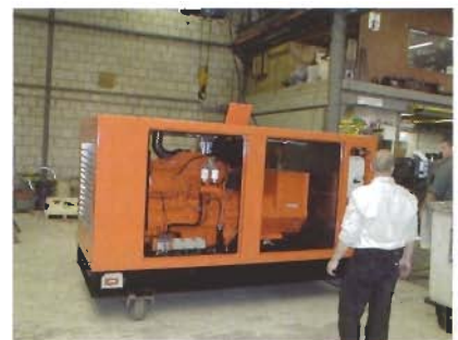
An emergency generator
