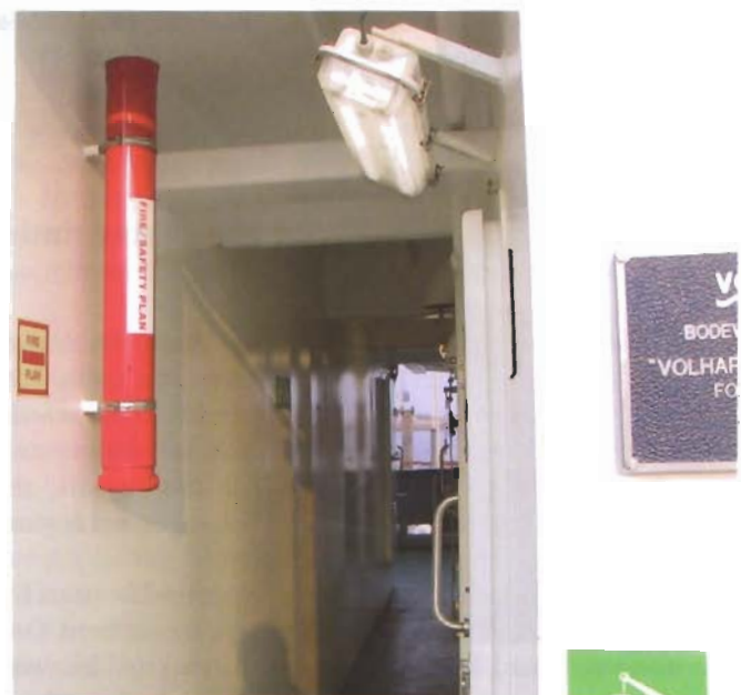
Cylinder containing the safety plan, easily accessible for the fire-fighters
