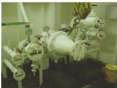
Fuel manifold on a large container-ship
