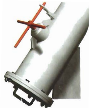
Pipe outside the chain locker, where the end link is connected. The wheel is used to secure a pin through the end link.
