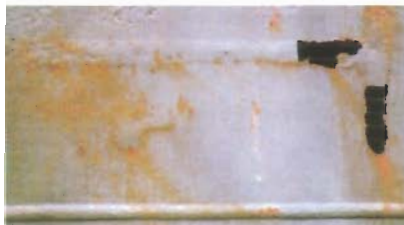
If the mill scale is not properly removed, it will eventually let go
