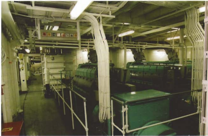
Auxiliary engine room of a ferry
