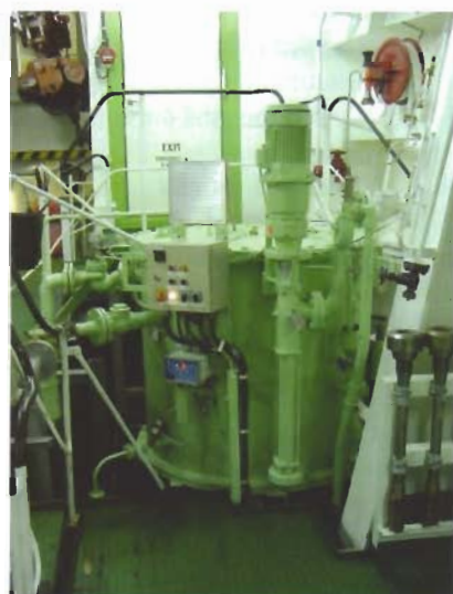
Bilge water separator with 15 ppm oil content meter / alarm
