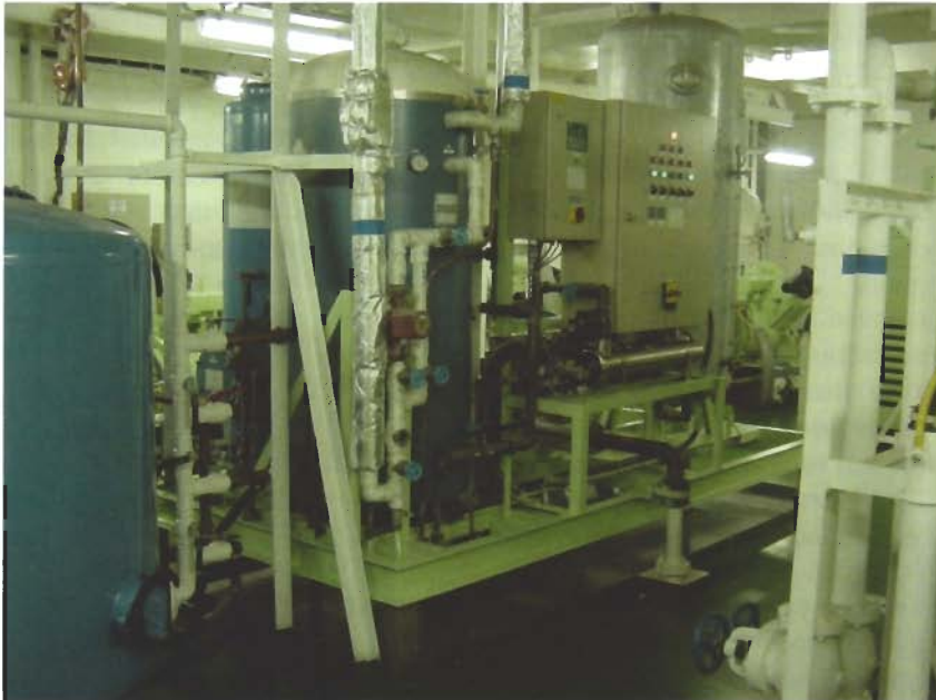
reverse osmosis plant
