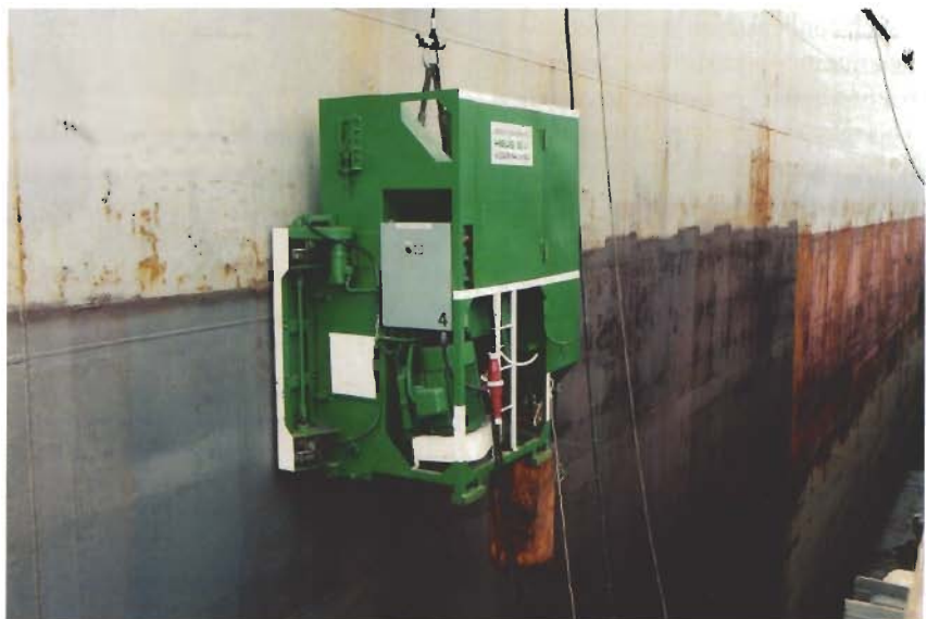
Advanced technique for gritblasting, with special care to prevent excessive inconvenience caused by 'dust'.
