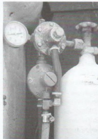
Propane tanks have a shutoff valve which should be closed when the stove is not in use for a period of time.
