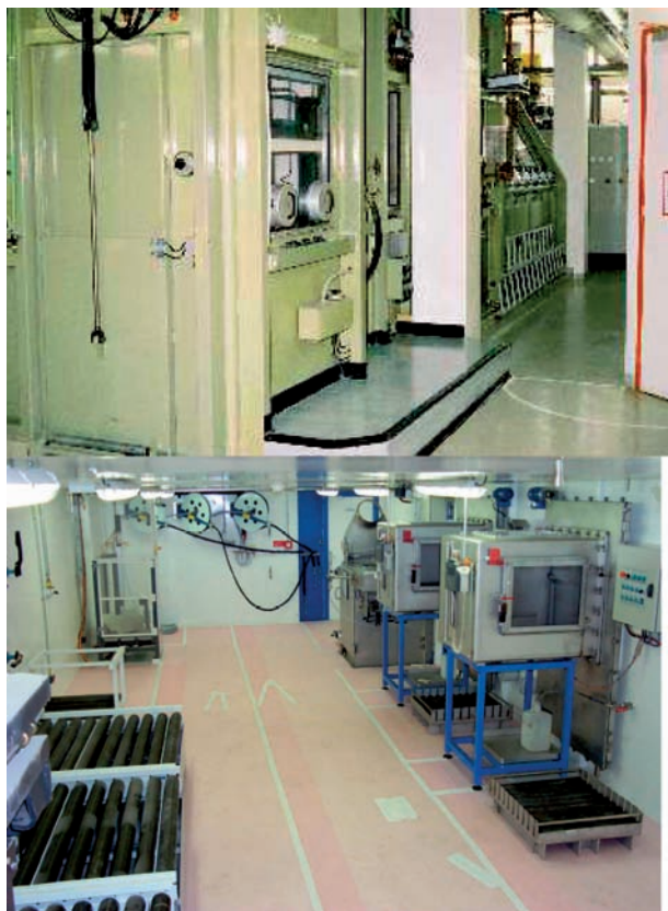
FIG. 13. Examples of waste segregation gloveboxes.
