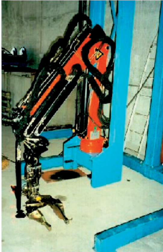
FIG. II-3. Small crane inside a cell.
