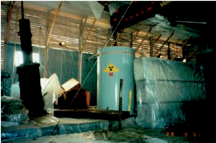
FIG. II-5. Control rod container on top of the SWR ready for transport to the interim store.
