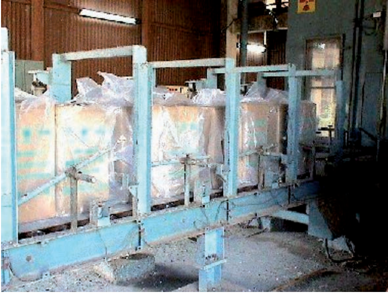
FIG. V-2. HEPA filters lined up on the compactor platform.
