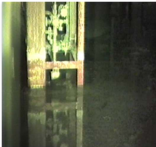
Figure 2.1. Contaminated water in the basement of the reactor building
