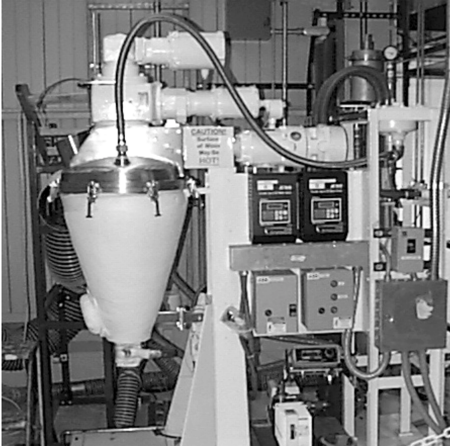
FIGURE 6.6.2 The integrated pilot-scale SPSS process installed at BNL.
