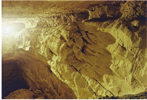
Fig. 6.19 Remains of a broken roof, mine workings row 7 south flank, photograph 2003. Source IfG [33]
