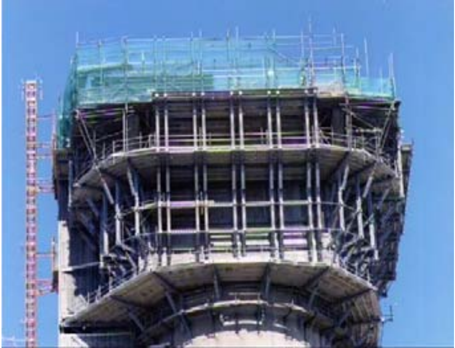
FIG. 11. Stack at Windscale Pile 2, United Kingdom. External access platforms.
