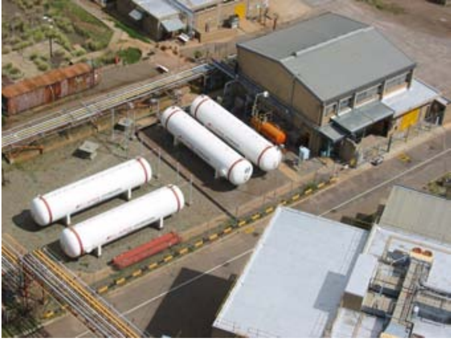
FIG. I.F-7. Operational hydrogen plant.
