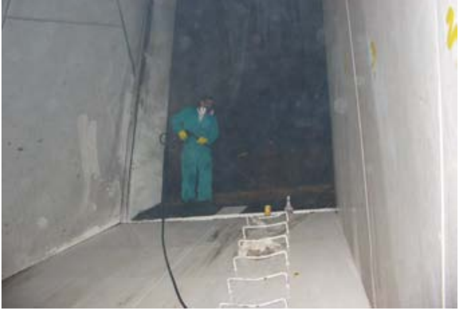
FIG. I.F-2. Epoxy coated plenum.
