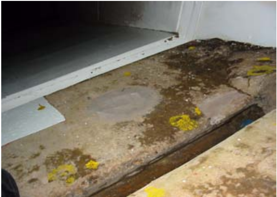
FIG. I.F-3. Water drain point.
