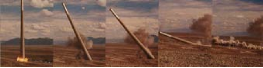
FIG. 4. Concrete stack (225 m high, 17 m dia., weight 9300 t) at Kennecott Copper Smelter, McGill, Nevada, USA.
