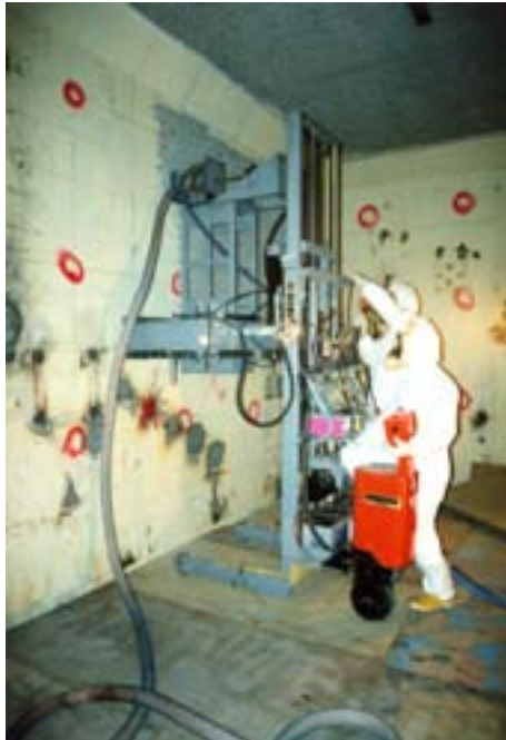
FIG. 8. JPDR decommissioning project. (a) Floor decontamination using a scabbler; (b) wall surface decontamination using a scabbler.
