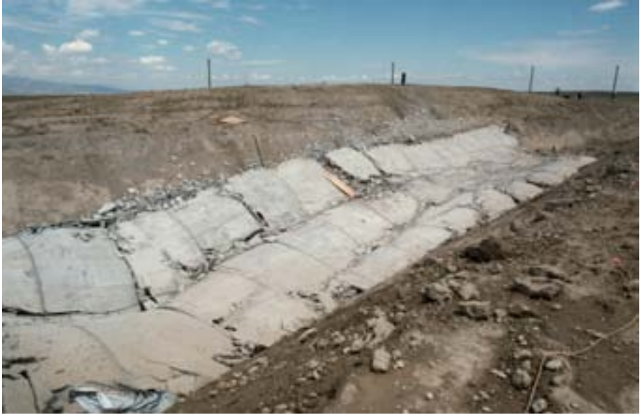
FIG. I.C-4. IET stack collapse after fall into trench.
