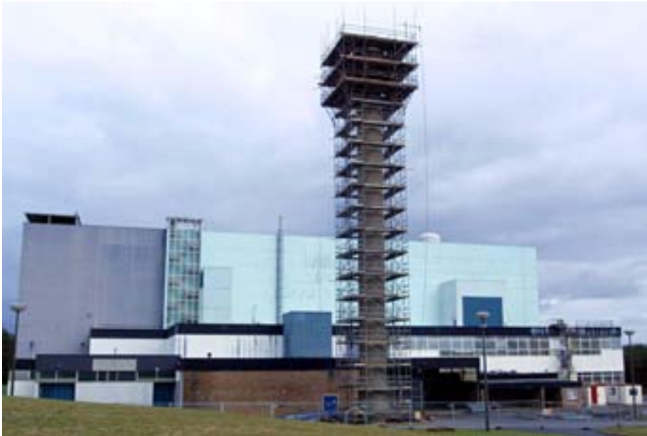
FIG. 10. Scaffolding used during dismantling of the stack of the Steam Generating Heavy Water Reactor, United Kingdom.
