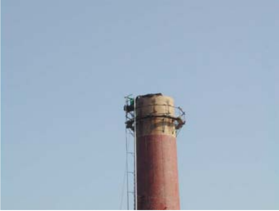
FIG. I.D-6. Stack platforms gone, less than 100 ft (30.5 m) of stack remaining.
