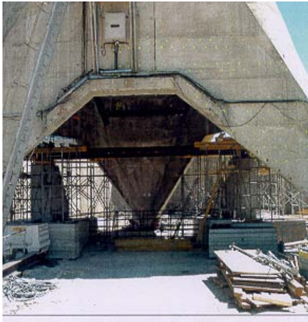
FIG. I.G-4. Consolidation of the foot of the stack with a solid mass of coarse concrete, support masses and hinges.
