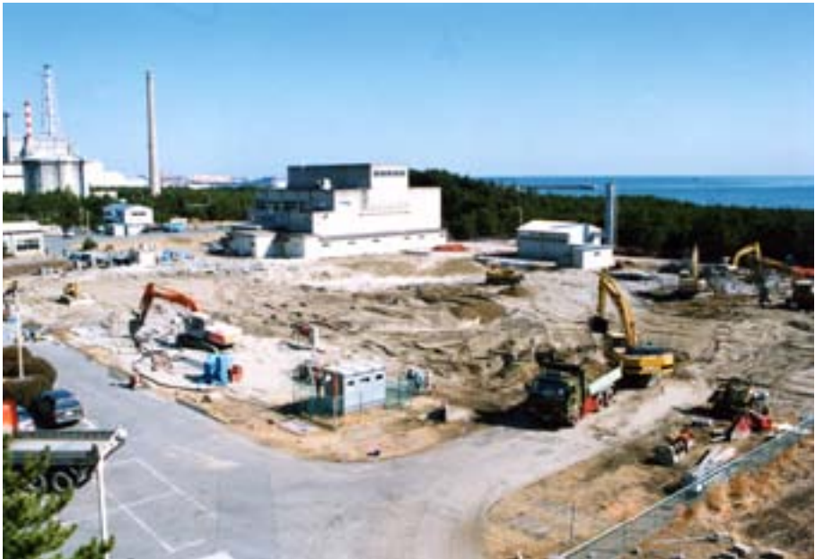
FIG. 2. Japan Power Demonstration Reactor. (a) View before decommissioning; (b) landscaping after building demolition.
