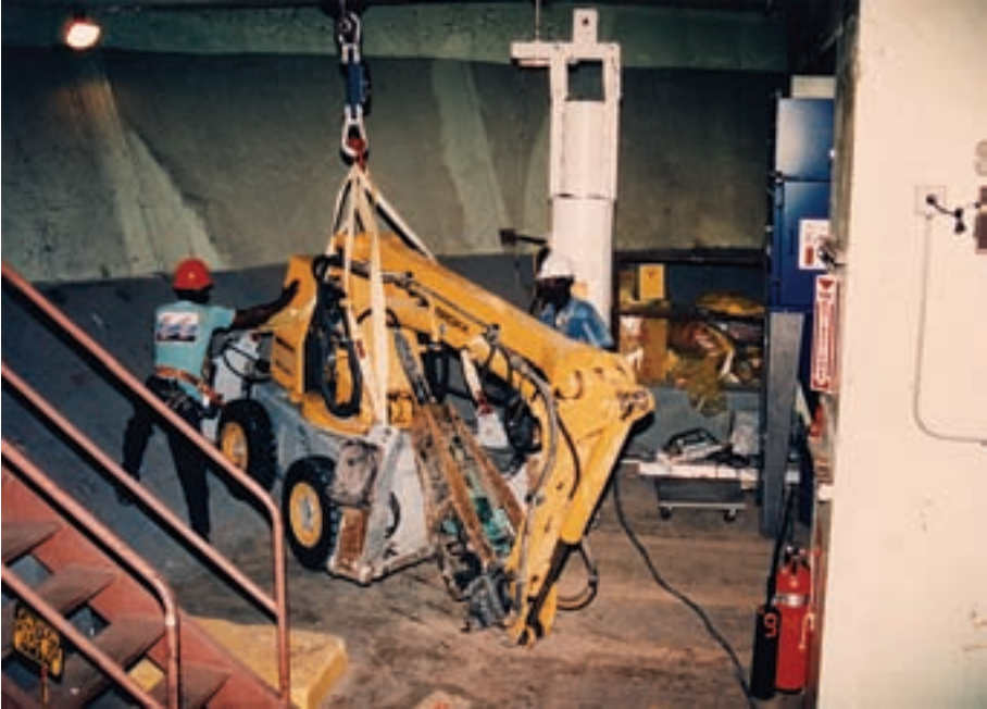
FIG. 21. BROKK excavator being lowered to the lower level at EBWR in preparation for the start of bioshield concrete removal (source: Argonne National Laboratory, USA, contract no. W-31-109 ENG 38).
