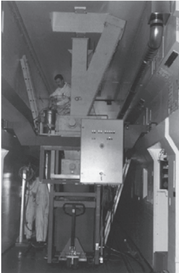
FIG. II-1. Graphite management in Switzerland: hammer crusher.
