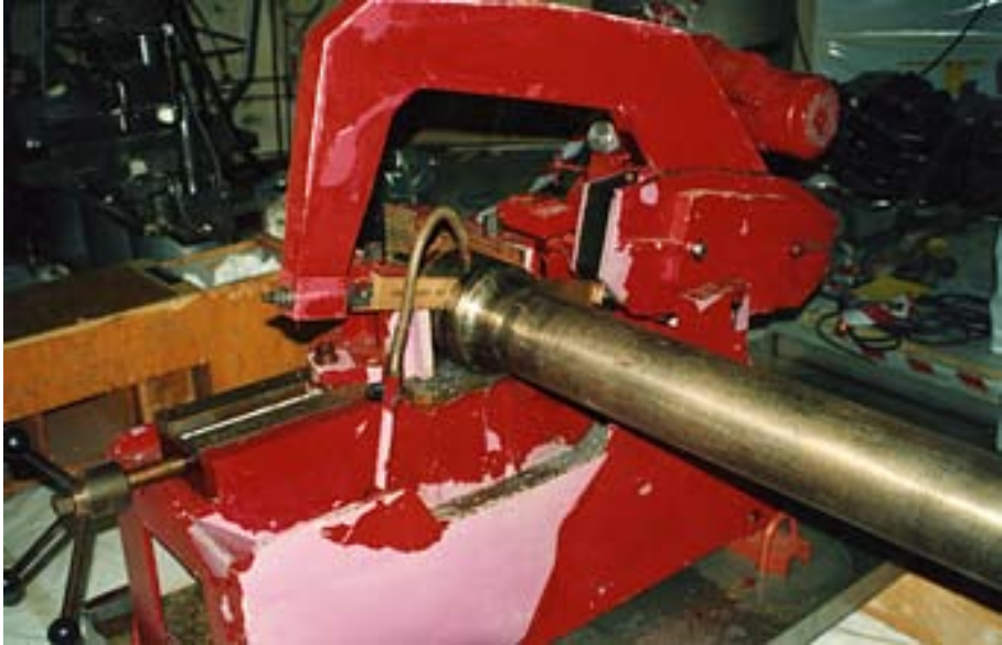
FIG. 20. Reciprocating saw cutting reactor head standpipes at the BR-3 decommissioning project, Belgium.
