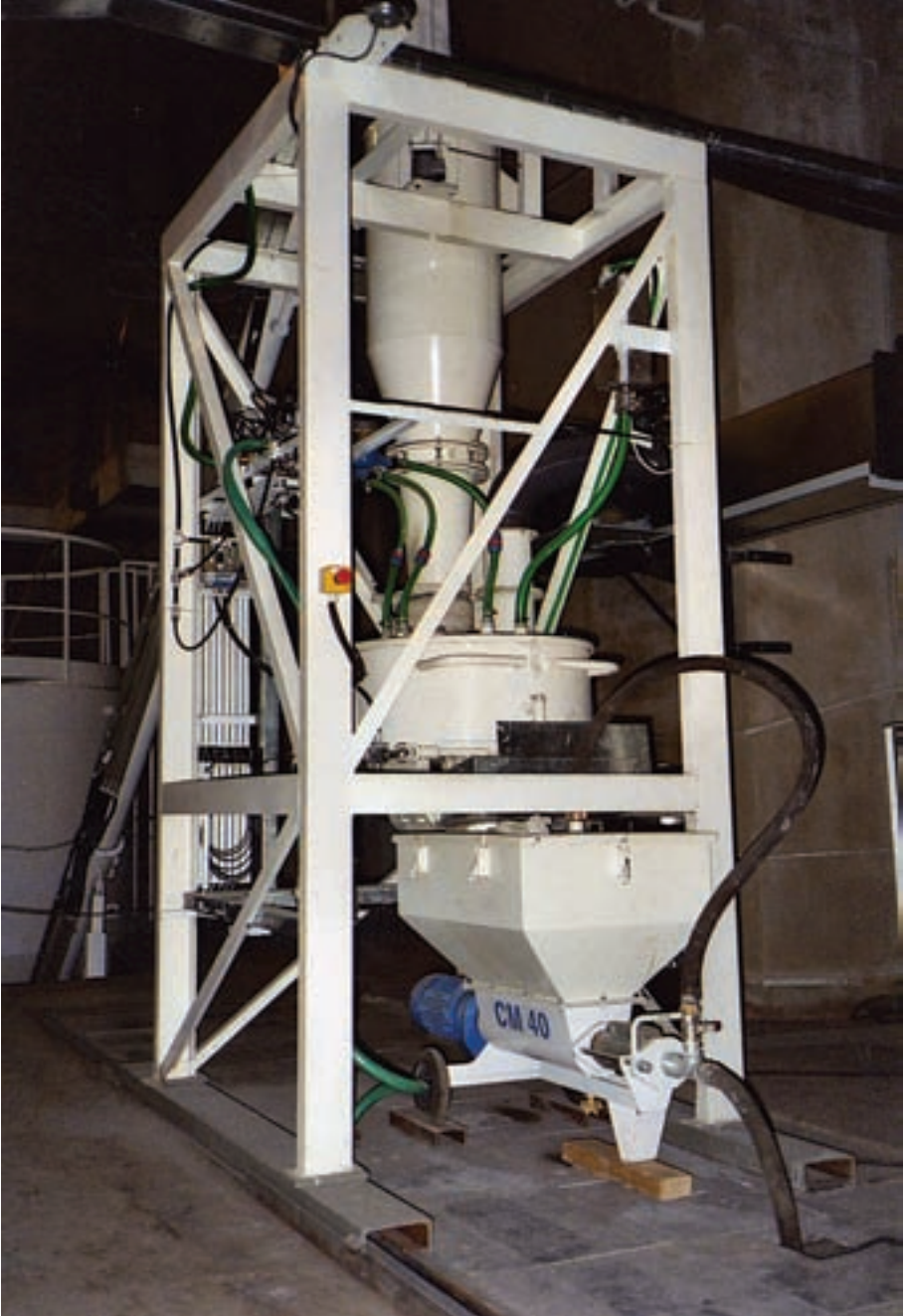
FIG. 12. The IRT reactor, Selaspils, Latvia: waste cementation plant (detail).
