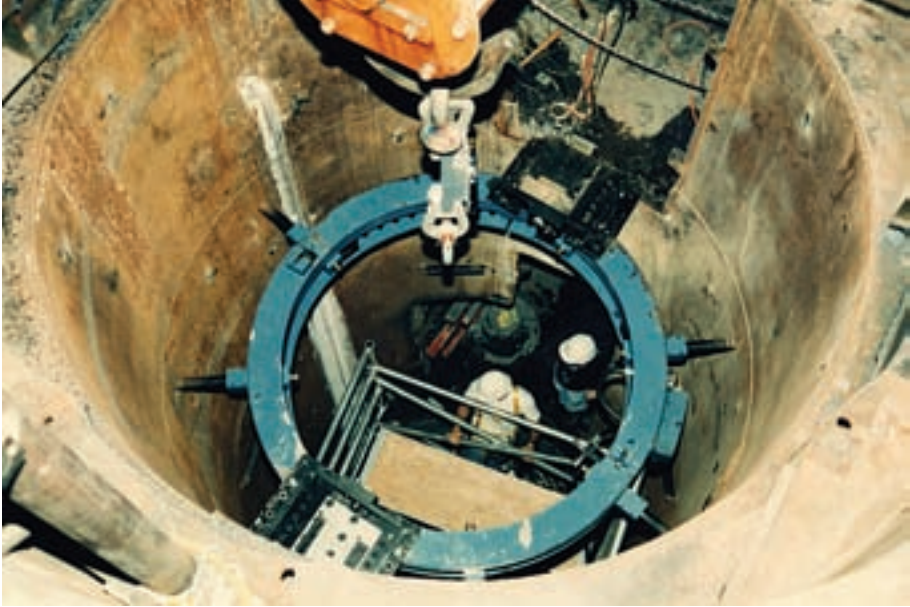
FIG. 10. Split ring cutting machine in place and ready to begin removal of the reactor vessel cavity liner at EBWR, ANL, USA (source: Argonne National Laboratory, USA, contract no. W-31-109 ENG 38).
