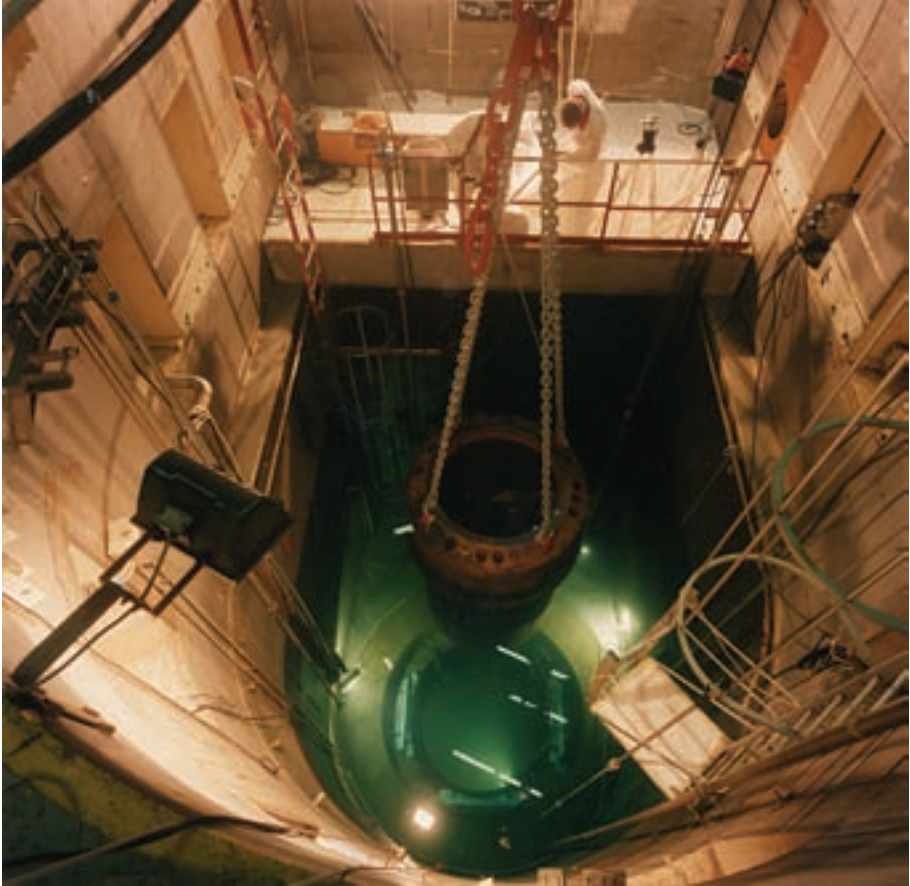
FIG. 8. BR-3 decommissioning project, SCK/CEN, Mol, Belgium: lifting the BR-3 reactor pressure vessel (RPV) (26 t).
