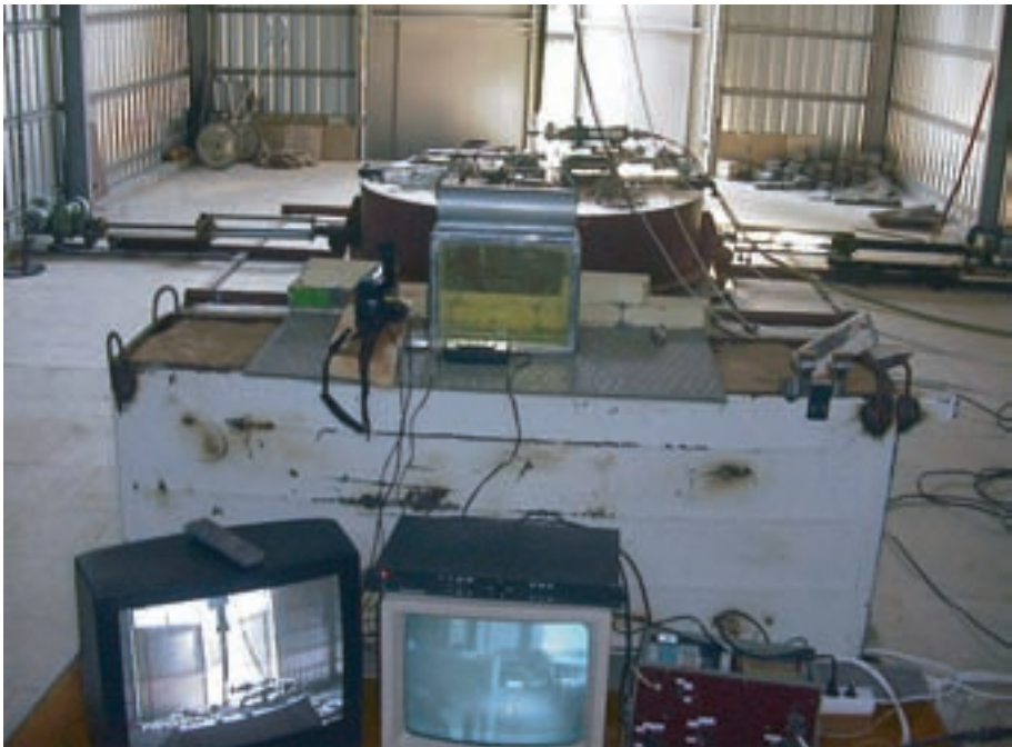
FIG. 30. Remote controlled system for cutting radioactive parts extracted from the first interim waste storage pit, Salaspils reactor, Latvia.
