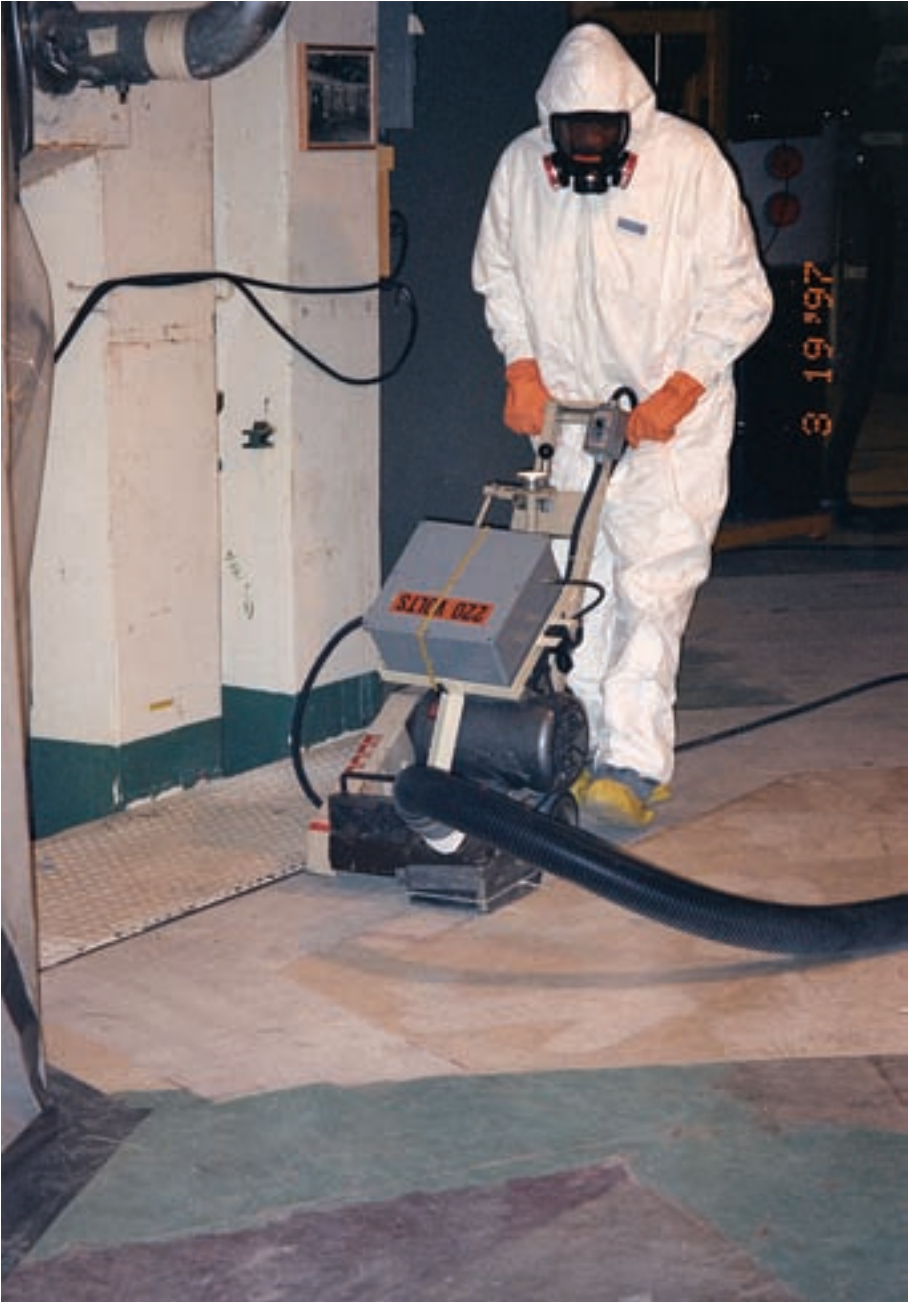
FIG. 23. ROTO PEEN sealer/VACPAC being used for decontamination of concrete surfaces at the CP-5 facility, USA.
