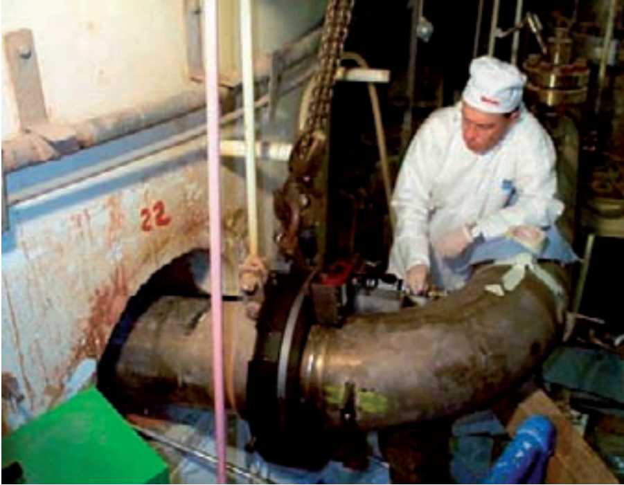
FIG. 7. The ALARA principle put into practice: on-site cutting into large pieces of the BR-3 reactor using a semi-automatic tool.
