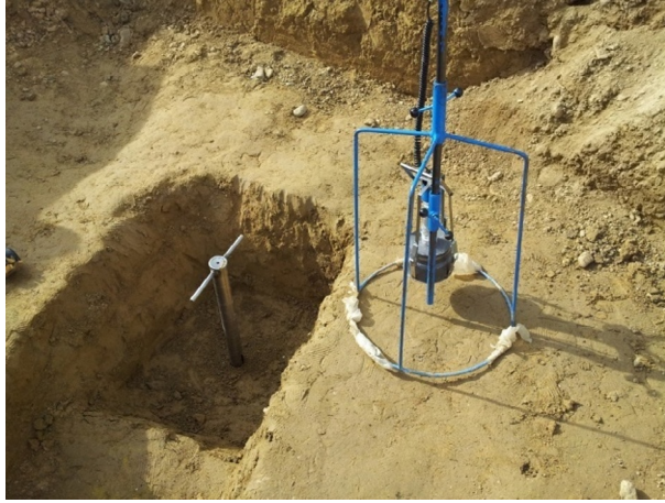
Fig. 10.4 Measurement and sampling of soil for the purposes of the site's final radiological survey.
