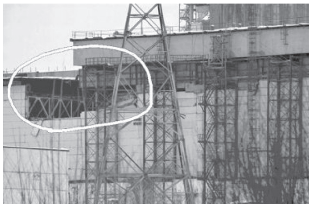
Fig. 9.9 Collapse of structures at the Shelter Object (area of collapse is shown in the white circles ).
