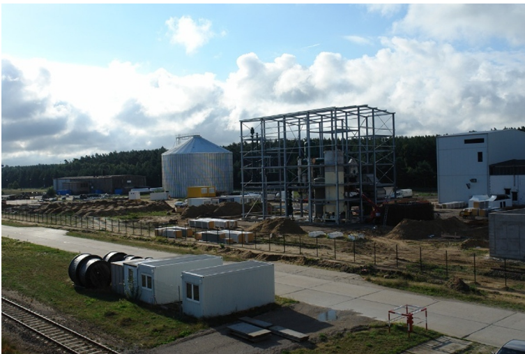
Fig. 3.4 Construction of a biodiesel plant at Greifswald nuclear power plant, Germany. A large decommissioning project has been underway at Greifswald since the early 1990s. To mitigate the social impacts from decommissioning, a massive industrial redevelopment was launched and is still ongoing. This has requested coordination of statutory parties with citizens’ committees, trade unions, and industrial entrepreneurs. (Nuclear decommissioning—planning, execution and international experience, in: M. Laraia, Woodhead Publishing, 2012, ISBN: 978-0-85709-115-4; Fig. 18.10).
