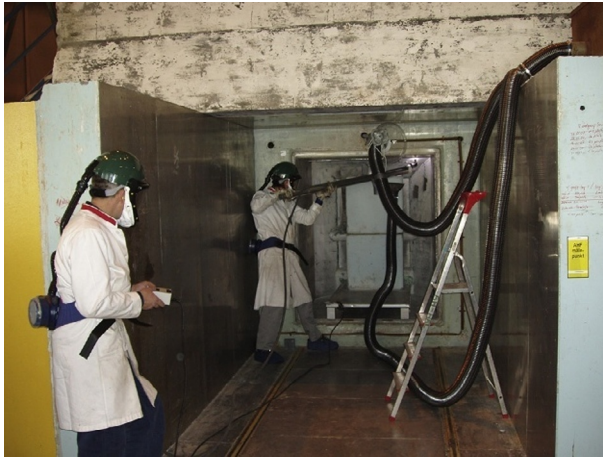
Fig. 11.2 Nose of thermal column being cut loose with a plasma cutter on an extension rod. From N. Strufe, 2009. Decommissioning of DR2. Final report. DD-38 Rev.1 (ENG). Danish Decommissioning, Roskilde. Available as a PDF-file from the Internet address: http://www.dekom.dk/media/24133/dr%20dr2_%20final%20report_eng.pdf .
