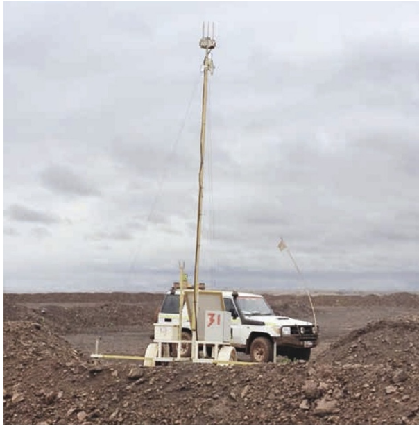
Fig. 8.3 ABB Tropos Solar Powered Wireless Router [45].
