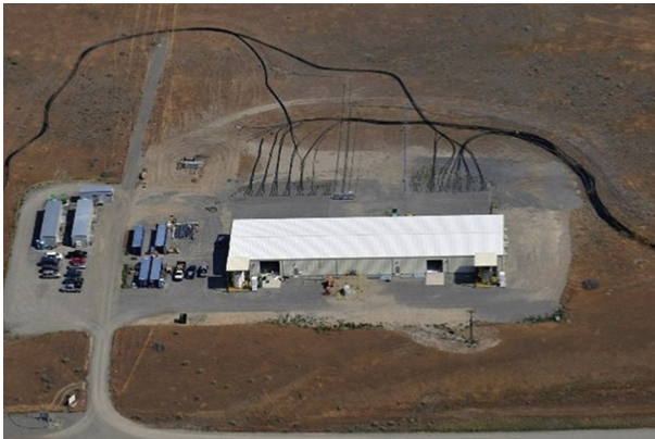
Fig. 13.3 Pump-and-treat remediation within the river corridor. From Mark Triplett, Pacific Northwest National Laboratory.
