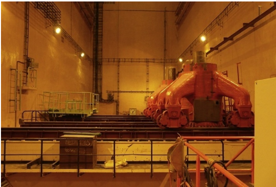
Fig. 9.16 Current state of refueling machines on reactor hall A1 NPP.
