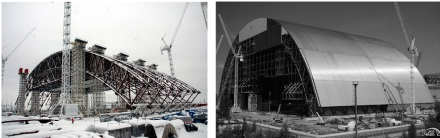
Fig. 9.7 Beginning and near completion of one half of the main arch structure.
