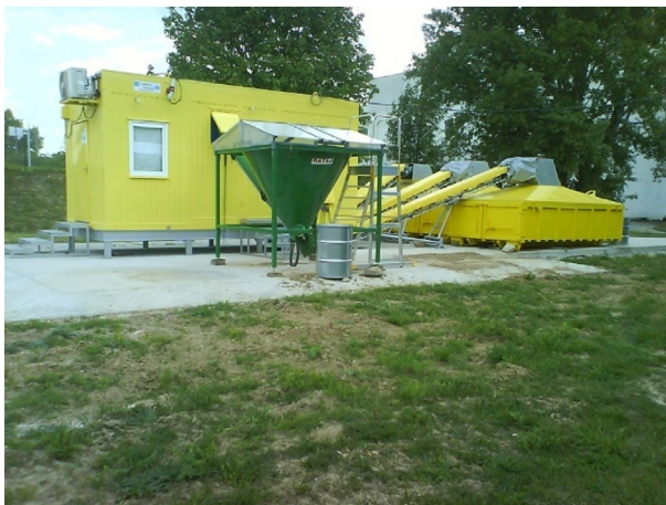
Fig. 10.1 Facility for measurement of contaminated loose materials.
