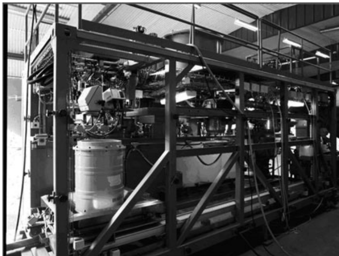
3.18 MOSS transportable waste grouting unit.
