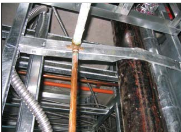
Figure 12-9 Shower Head Rough-in (Poor)
