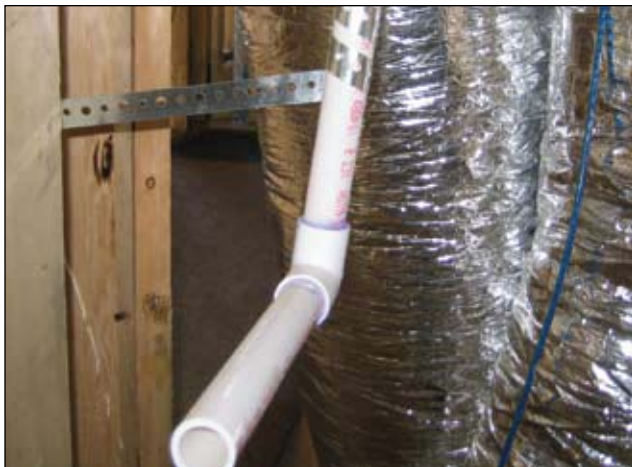
Figure 12-5 Condensate Drain Stub-out (Poor)
