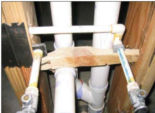
Figure 12-6 Sink Rough-in (Poor)
