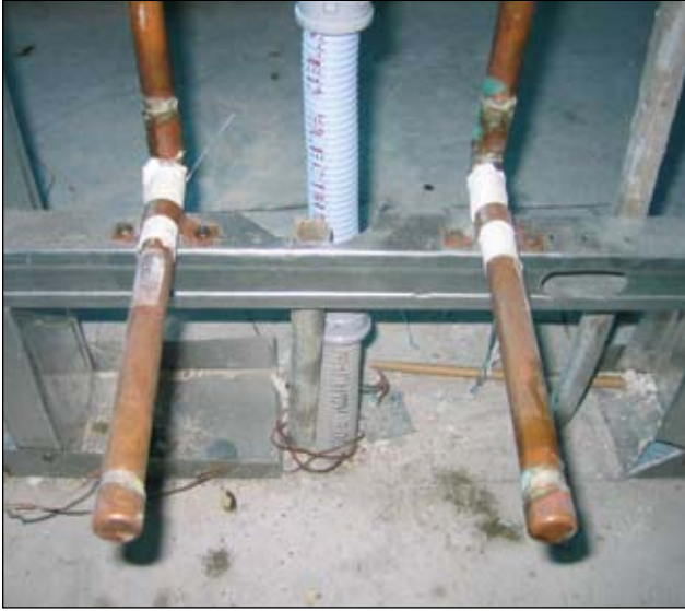
Figure 12-11 Poor Attempt at Dissimilar Metal Isolation
