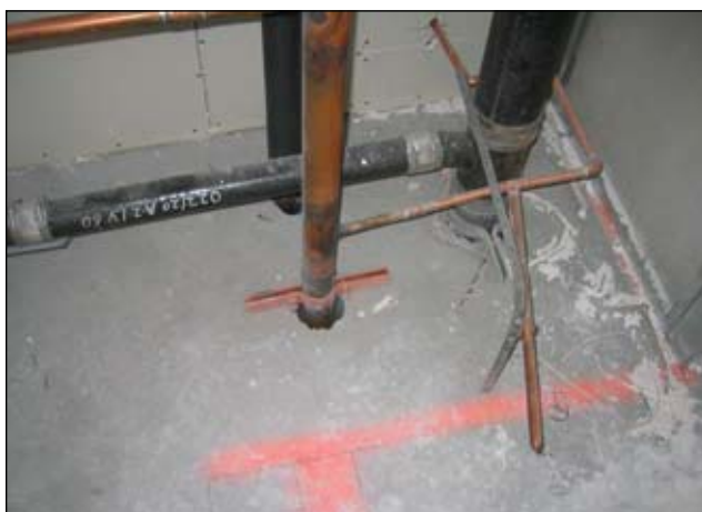
Figure 12-7 Toilet Rough-in (Poor)
