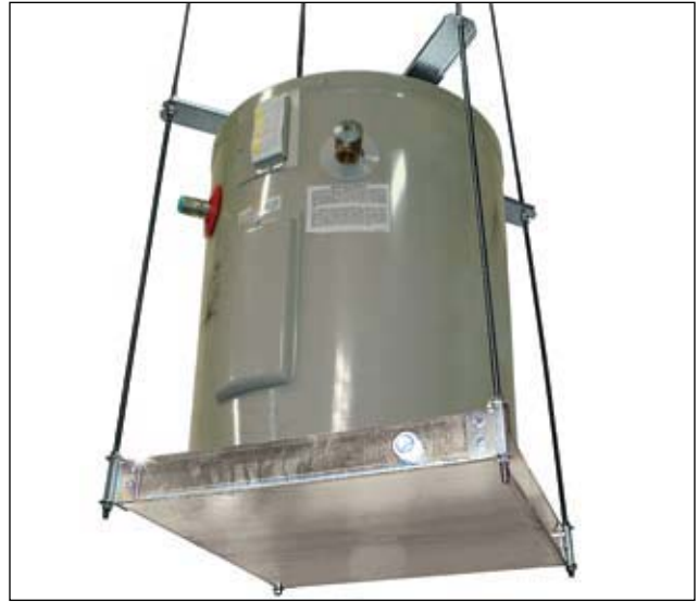
Figure 12-16 Engineered Suspended Equipment Platform
