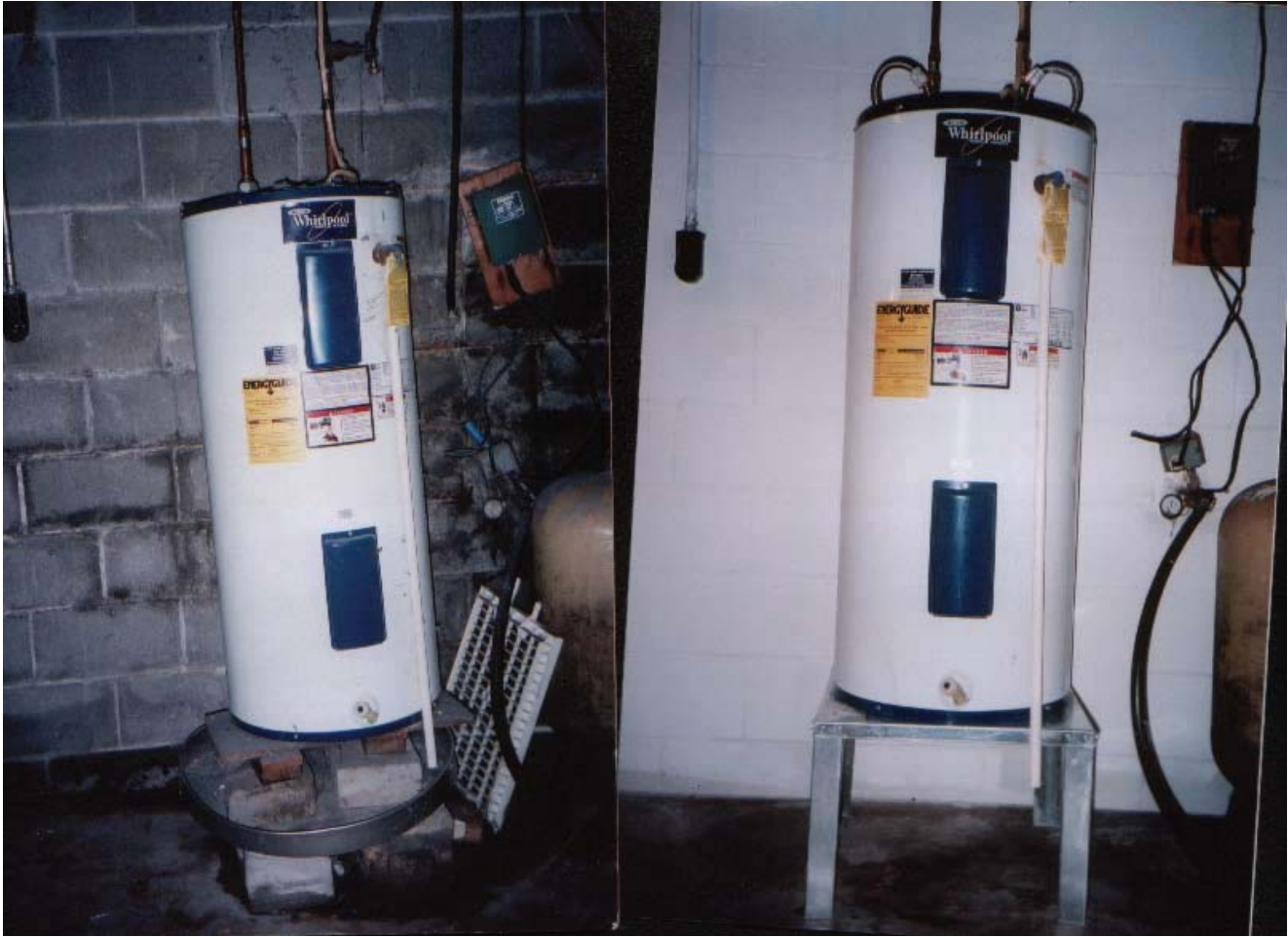
Figure 12-1 A Makeshift Attempt to Support a Water Heater versus an Engineered Solution
