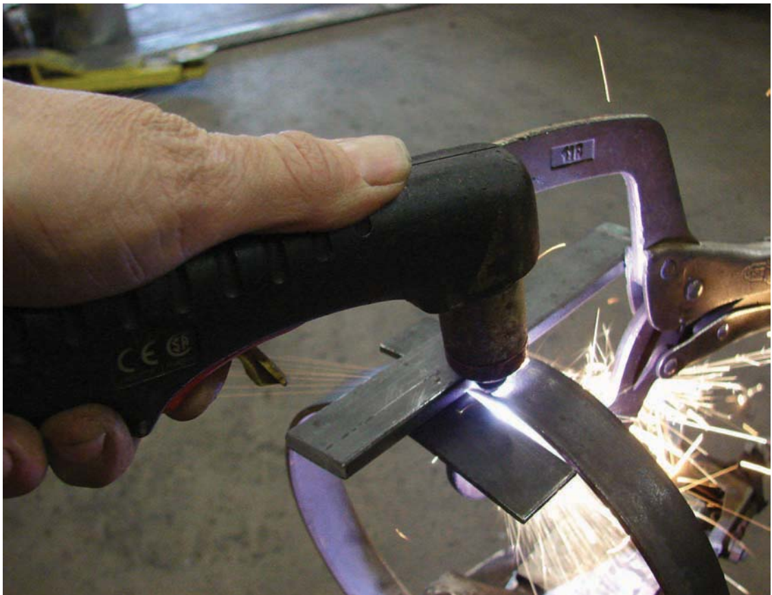
Figure 13-10. Use a plasma cutter to remove the flat ends on the ring.
