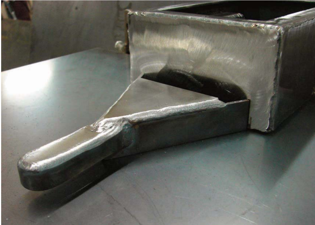
Figure 2-22. Completed hitch aligned and ready to be welded to the wagon body.
