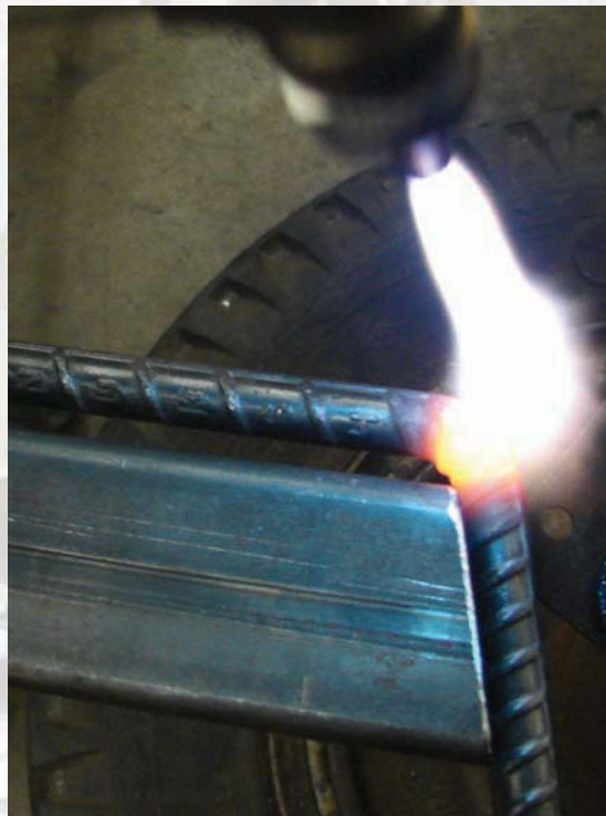
Figure 10-5. Use a template when bending the rebar to help achieve the intended angle.
