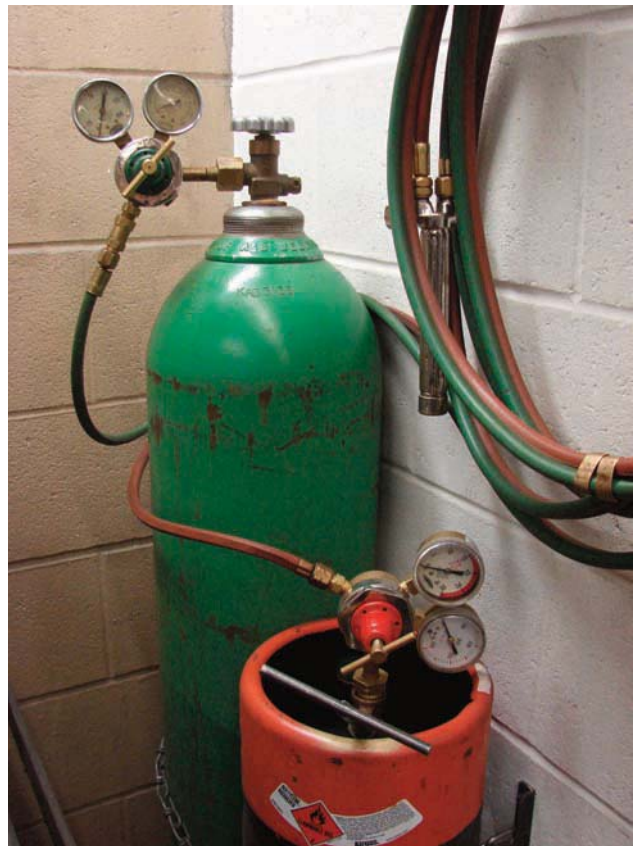
Figure 6-8. An oxyacetylene station includes an oxygen cylinder with attached regulator, an acetylene tank with attached regulator, hoses, and a torch handle. The setup is color coordinated. The green hose is always attached to the oxygen cylinder and all fittings for the setup are right hand threaded. Red hoses attach to the acetylene and the fittings are left hand threaded. These pairings ensure proper hookups without any confusion.
