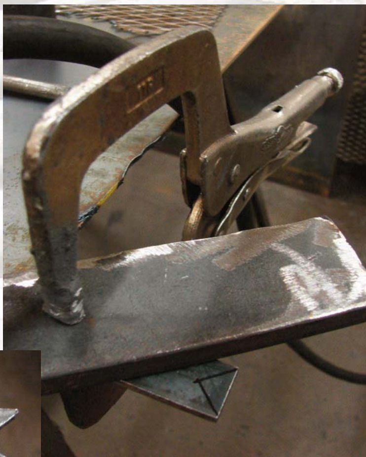
Figure 2-14. a) Use C-Clamp locking pliers and a straight edge to make a straight cut in the hitch tongue top.
