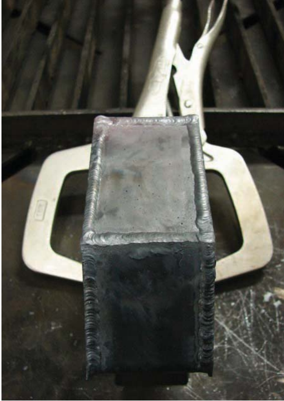
Figure 7-30. Weld the four welds on the bottom of the vase, rotating from side to side with each weld.
