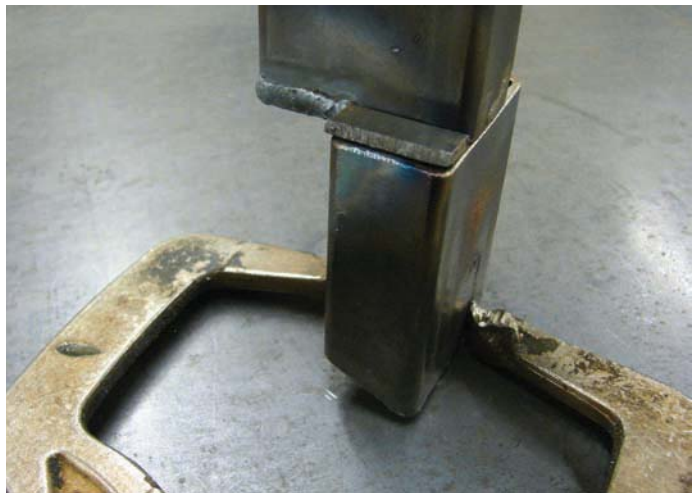
Figure 9-14. C-clamp locking pliers work well to hold the base upright while welding the seat base front side caps in place.
