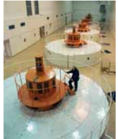
Figure 6.4 Six generators in an Icelandic hydroelectric power station. Each generator produces 45 MW of electrical power.
