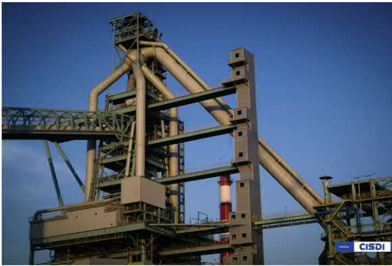
FIGURE 51.3 Blast furnace top equipment including charging conveyor on the left, three of the four top gas uptakes leading to the cross-over main, and downcomer pipe that delivers raw top gas to the gas cleaning plant. Source: Photo courtesy: CISDI International Engineering & Consulting Co., Limited.
