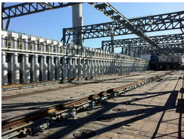
FIGURE 55.7 View of the coke plant roof showing the stand pipes where gases are collected from each oven, the rail mounted charge car used to top charge coal to each oven through four charge holes. Source: Photograph courtesy of thyssenkrupp Industrial Solutions AG.
