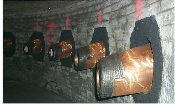
FIGURE 1.5 New tuyeres in a rebuilt blast furnace. They are water-cooled copper with a protective metal coating near the tip. Tuyeres are about 0.15 m inside diameter and penetrate about 0.4 m into the furnace. They are situated about 3 m above the blast furnace taphole and are about 1.2 m apart around the blast furnace circumference. 1200^\circ\text{C} blast air enters the tuyeres at 180–240 m/s and a pressure of 3.5–4.5 bar (gauge). Source: Photograph courtesy of Stelco Holdings Inc.
