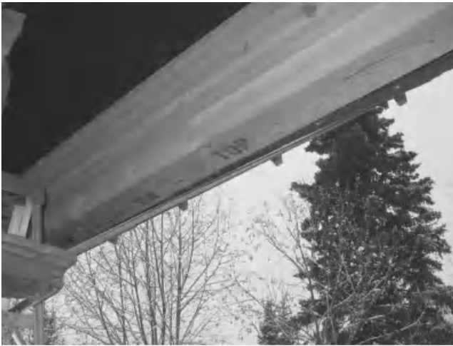
Figure 4.3.2-1 Glulam beam improperly installed upside-down (Photo courtesy of Boise Cascade Corporation, Boise, Idaho.)
