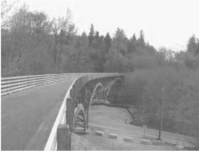
Figure 17.2.6-1 Horizontally curved glulam deck-arch bridge. (Photo courtesy of Western Wood Structures, Inc., Tualatin, Oregon)
