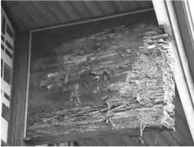
Figure 1.5.1-1 Advanced decay of unprotected glulam beam.
