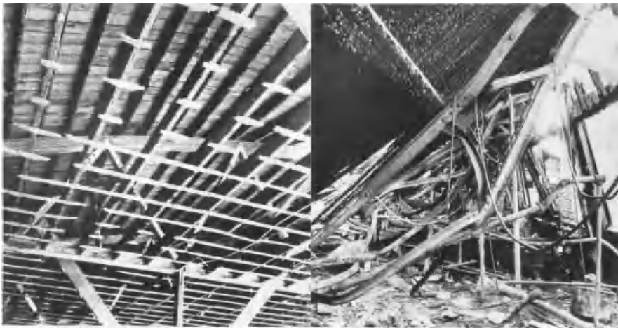
Figure 20.5-4 Glulam trusses (left) supported roof throughout fire, while steel trusses (right) collapsed.
