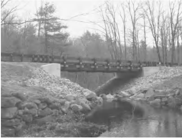
Figure 17.2.2-1 Longitudinal glulam deck vehicular bridge, 40-ft span. (Photo courtesy of Western Wood Structures, Inc., Tualatin, Oregon)
