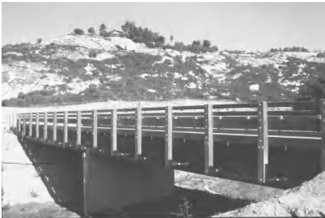
Figure 17.2.4-1 116 ft glulam girder vehicular bridge. (Photo courtesy of Western Wood Structures, Inc., Tualatin, Oregon)
