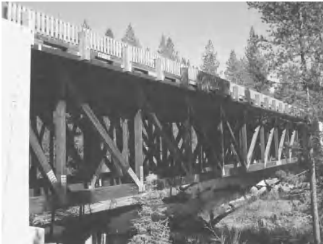
Figure 17.2.5-1 Glulam deck-truss vehicular bridge. 148 ft span. (Photo courtesy of Western Wood Structures, Inc., Tualatin, Oregon)
