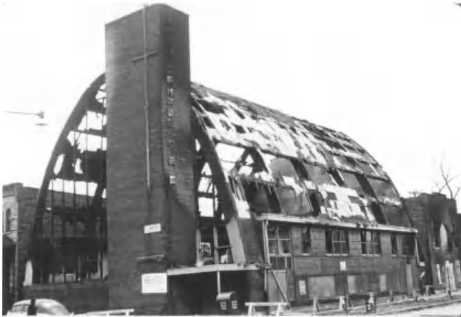
Figure 20.3.2-1 Glulam framework remains standing after devastating fire at Zion Baptist Temple.
