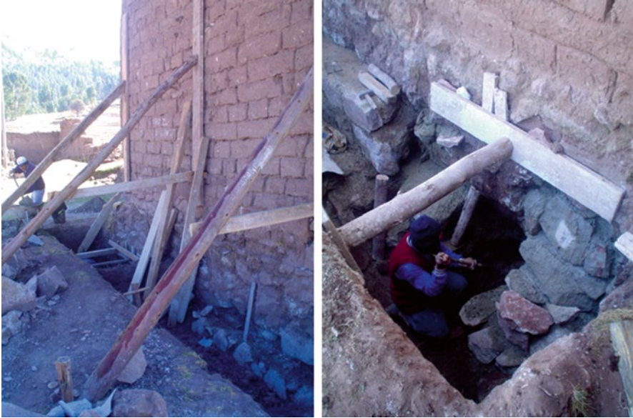
Fig. 5.49 Foundation repair work: underpinning of the foundation of an earth block wall [85]
