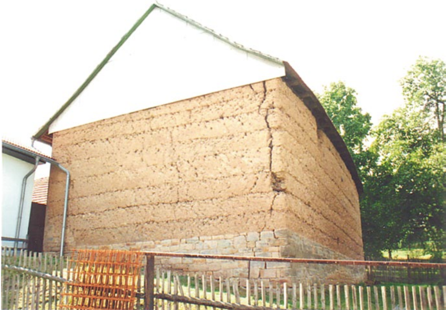
Fig. 5.45 Structural damage caused by planning mistakes: cracks in a cob wall caused by uneven settling of the building ground [30]
