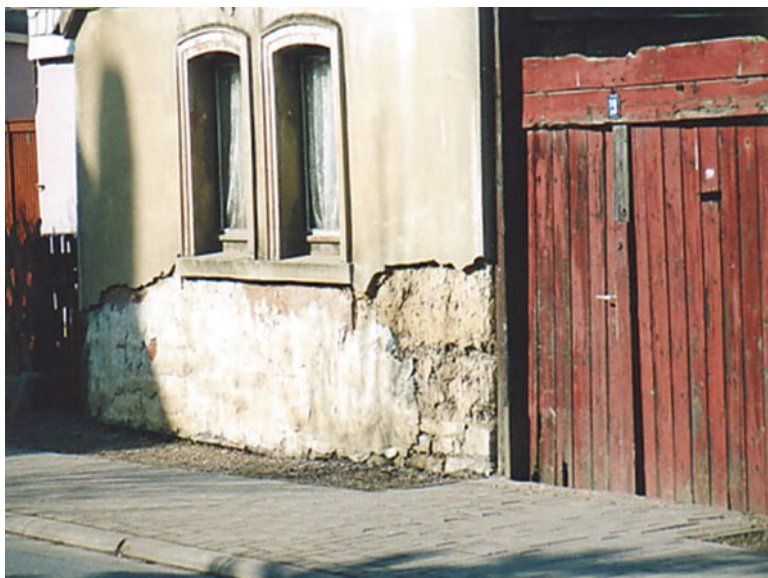
Fig. 5.15 Structural damage in the stem wall area caused by raising of the street level [30]
