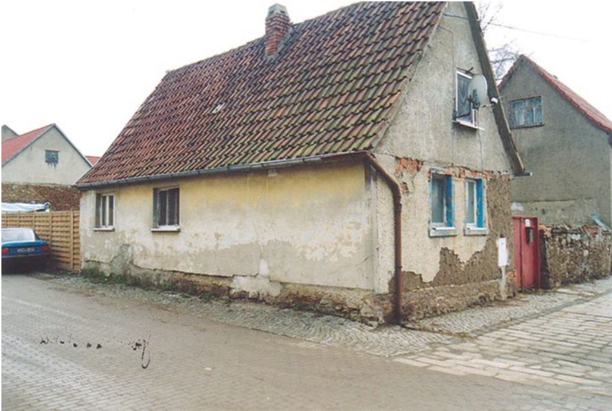
Fig. 5.17 Structural damage in the stem wall area: crystallized salts visible as a gray to white film within the capillary fringe [30]
