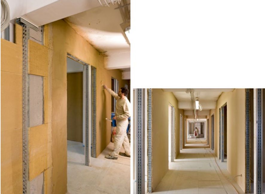
Fig. 5.63 Sustainable renovation using clay plaster boards, UN Framework Convention on Climate Change, Bonn, 2011 [81]
