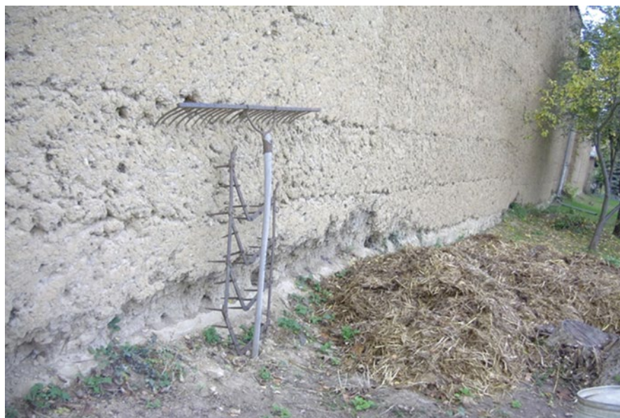
Fig. 5.16 Structural damage in the stem wall area: salt attack, intensified by a manure pile
