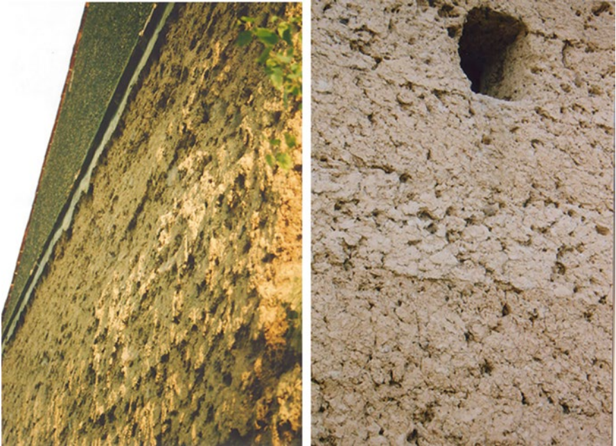
Fig. 5.21 Cob wall surfaces: “normal” erosion due to weathering [30]
