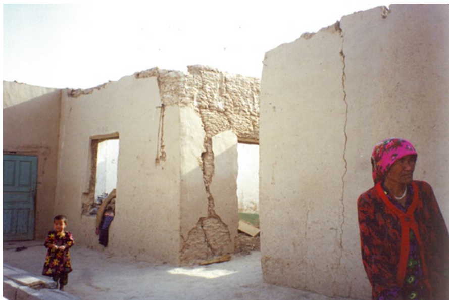
Fig. 5.37 Damage patterns after earthquake impact: destroyed residential building made of cob (pachсах) (Kamashi, Uzbekistan, 2000 [45])
