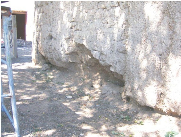
Fig. 5.13 Weakening of the cross section of a load-bearing earth wall caused by salt attack in the foundation and stem wall
