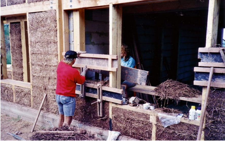
Fig. 3.19 Shaping during the installation of light straw clay: formwork panels as temporary formwork
