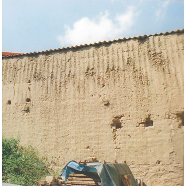
Fig. 5.22 Cob wall surfaces: erosion channels formed by concentrated flows of draining rainwater [33]
