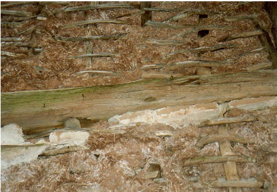
Fig. 5.18 Wall surface of a half-timber structure: exposed stake work caused by erosion of the earth building material [30]
