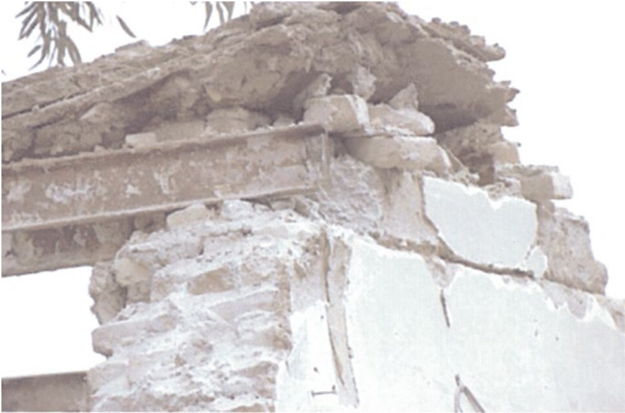
Fig. 5.42 Damage patterns after earthquake impact: steel ceiling joist laid on earth block wall coping without load distribution, Bam, Iran, 2003 [46]
