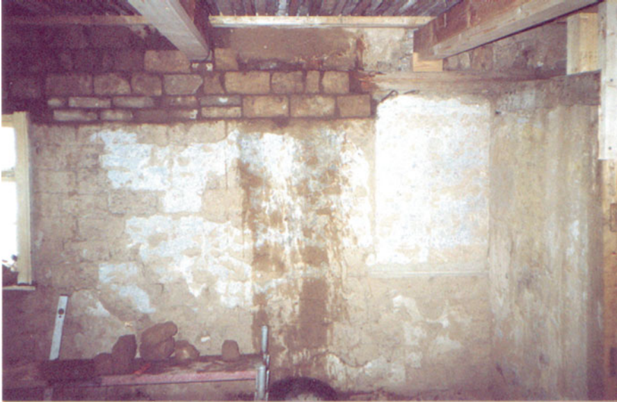
Fig. 6.1 “True recycling”: repair work on an existing earth block masonry wall using salvaged earth blocks [14]
