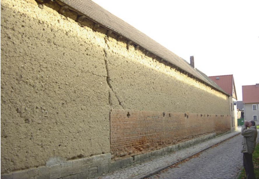
Fig. 5.43 Structural damage caused by improper execution of work: vertical crack in cob wall caused by a difference in wall height
