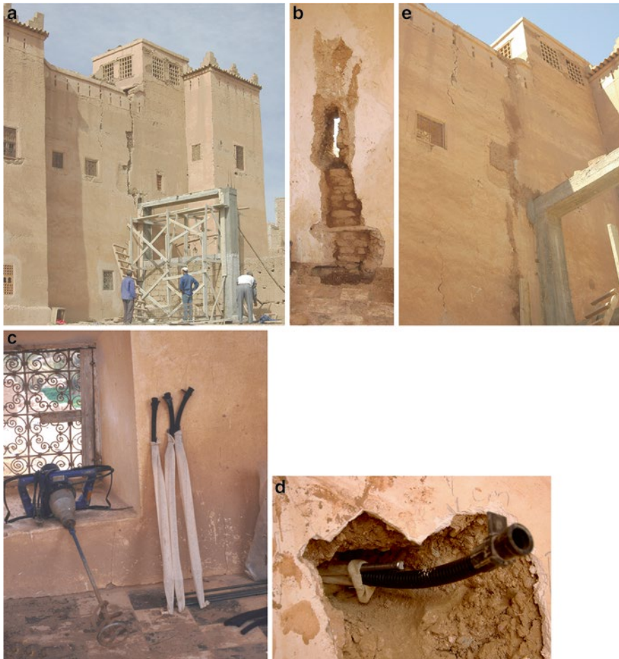
Fig. 5.57 Repair of earth block walls, crack repair: pinning [76]. (a) Reinforced steel frame installed as emergency shoring before crack repair, (b) filling of cleaned crack with earth blocks, (c) steel pins and plastic hose inserted in gauze tube, (d) steel pin inserted into drill hole, and (e) view of wall after the crack repair
