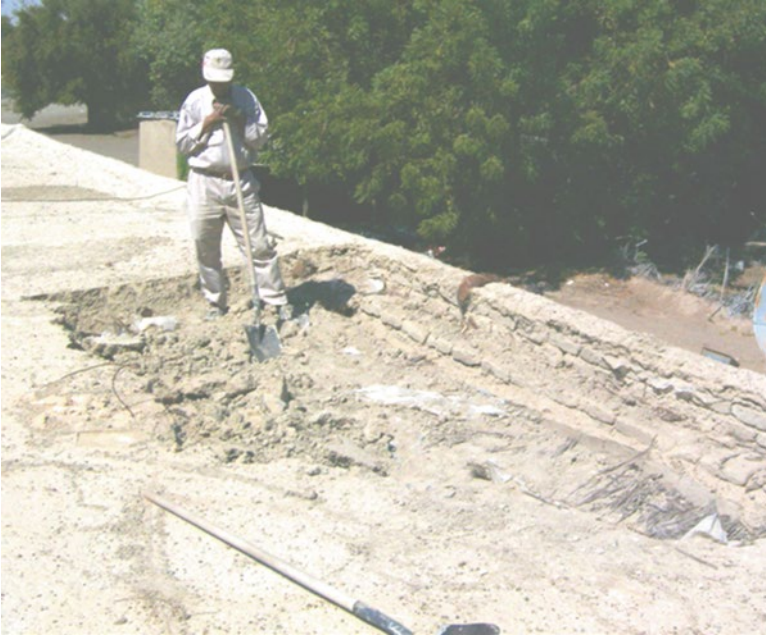
Fig. 5.60 Traditional flat roofs made of earth building materials: repair of the roof seal (plastic membrane)
