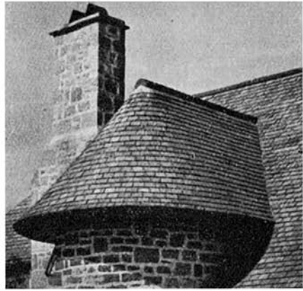
Fig. 9.—12-IN. BY 6-IN. OLD DELABOLE SLATES ON A CIRCULAR TURRET ROOF; MITRED VALLEY
