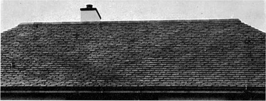
Fig. 2.—OLD DELABOLE SLATING—RANDOM-WIDTH SLATES OF A STANDARD LENGTH LAID TO A REGULAR GAUGE
