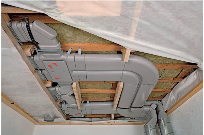
Rigid and semi-rigid duct used to achieve air distribution.
