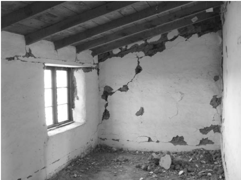
19.4 Damage in 2010 to an unreinforced replica historic building constructed in 1977 of unstabilised rammed earth near to Darfield, New Zealand.
