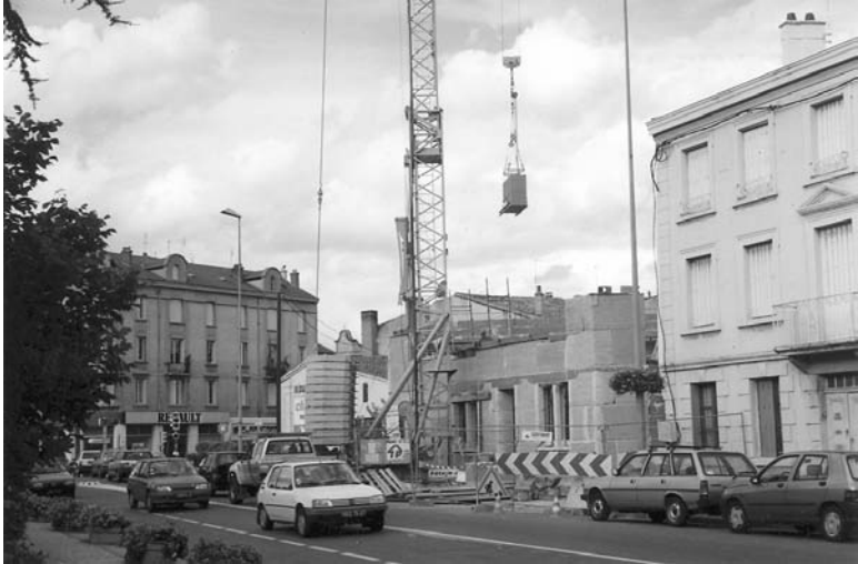
23.18 Pre-fabricated earth walls being craned into position during construction at Montbrison, Loire (© Nicolas Meunier, 1995).
