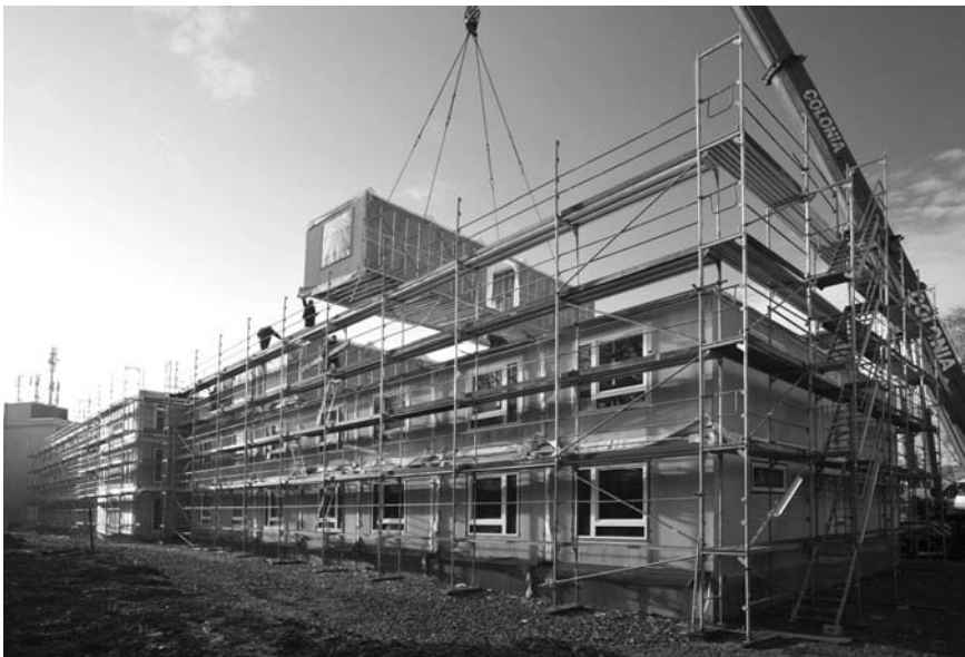
5.30 The modules under construction. Photo courtesy of Kleusberg GmbH & Co KG, Wissen, Germany.
