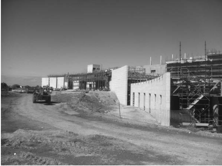
1.1 RACV Project, Torquay, Australia. Insulated SRE cladding a steel portal frame to 11.2 m height using telescopic handler access (© Earth Structures Pty Ltd, 2011).
