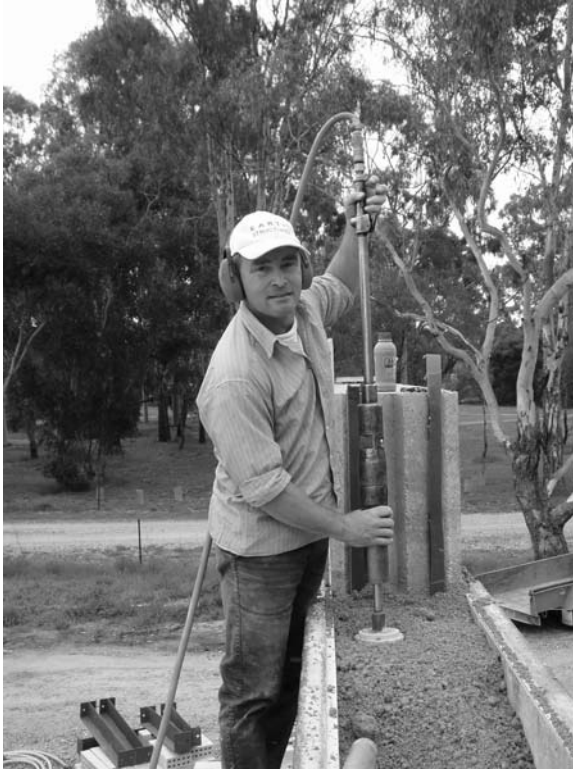
22.7 A pneumatic rammer. Note the access for the operator to the formwork and material. The actual ramming is the least physically demanding aspect of an SRE builder's day.
