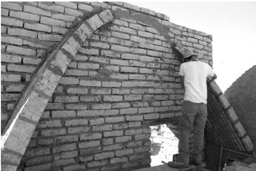
17.18 Nubian vault under construction in Texas by masons trained by the Adobe Alliance (photo: Adobe Alliance).
