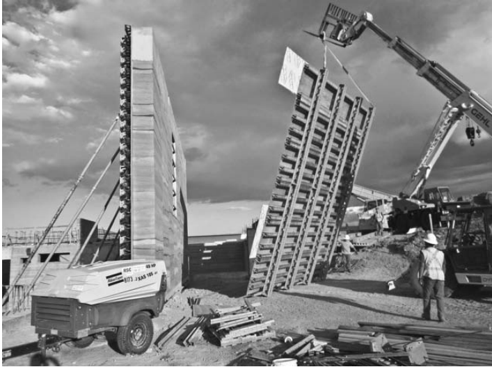
1.5 Formwork stripping at Southeast Wyoming Welcome Center, Wyoming: in order to meet tight timelines, larger panel sizes are useful (© SIREWALL Inc., 2011).
