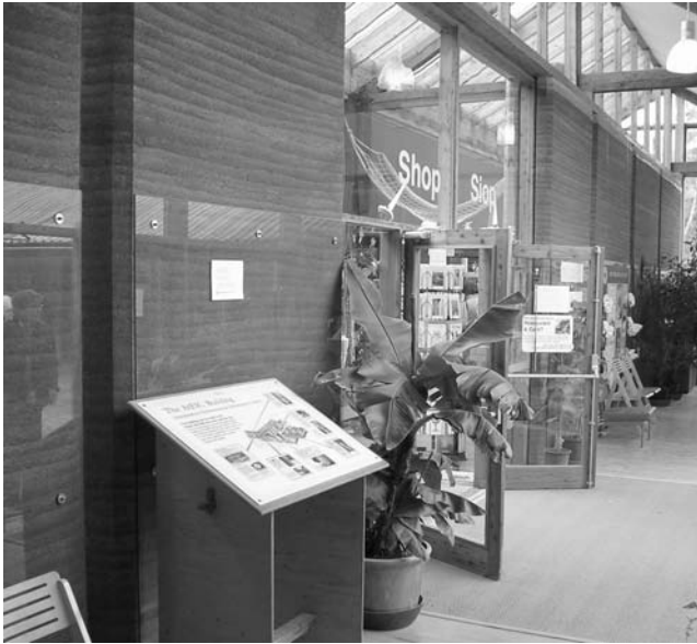
23.2 Unstabilised rammed earth internal wall at the Autonomous Environmental Information Centre (AtEIC), Centre for Alternative Technology (CAT), Wales (© M R Hall, 2004).
