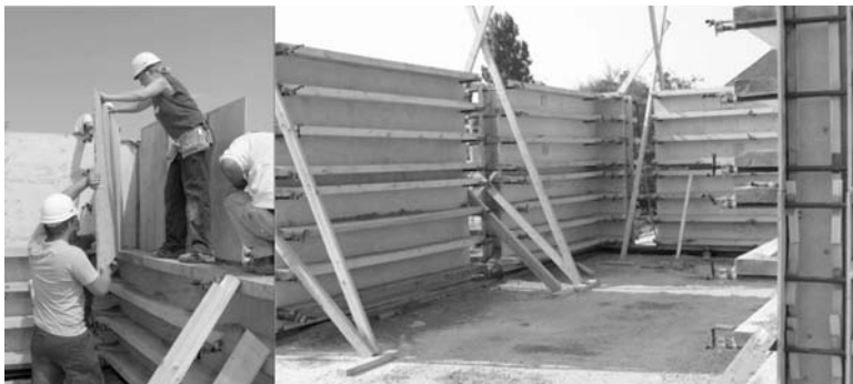
23.5 California-style timber formwork system in use during the construction of a stabilised rammed earth pavilion, Chesterfield, UK (© M R Hall, 2003).
