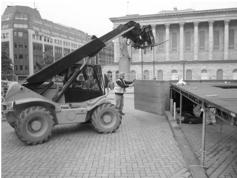
23.27 Pre-cast SRE wall sections with internal steel reinforcement being delivered and offloaded from a flatbed truck in Birmingham city centre (© Earth Structures Europe Ltd, 2008).
