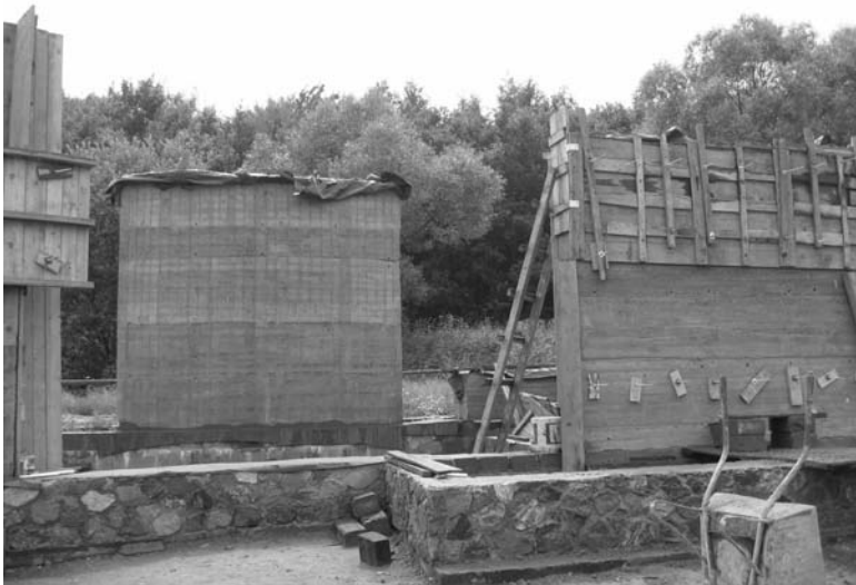
23.31 Panelled timber rammed earth formwork used at the Pašek experimental research house (© Teresa Kelm, 2008).
