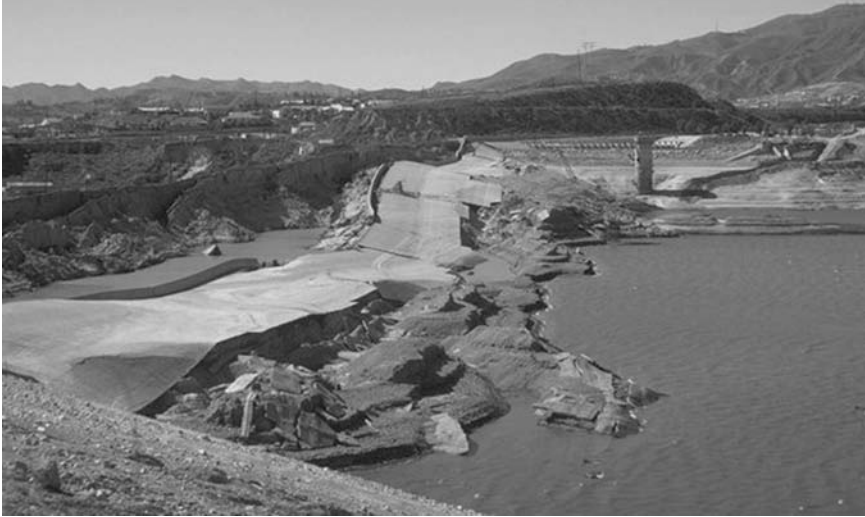
20.14 Liquefaction damaged dam during earthquake.
