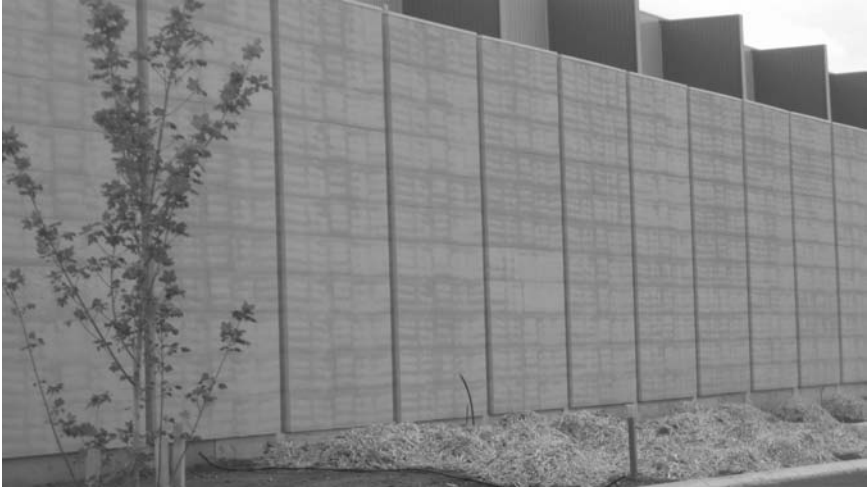
22.12 A series of monolith SRE panels showing horizontal form lines and plugged bolt holes. Note the folded steel capping along the wall heads. Pitruzello olive processing plant, Sunbury, Victoria.
