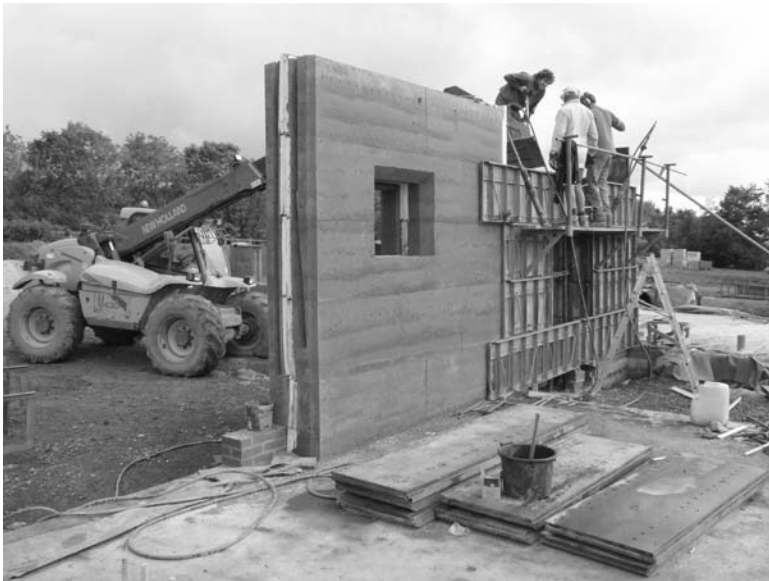
23.7 Stabilised rammed earth wall with extruded polystyrene cavity insulation and small opening with chamfered edge detail and the Stabilform™ formwork system, at Straightways Farm, Devon, UK (© Earth Structures Europe Ltd, 2007).
