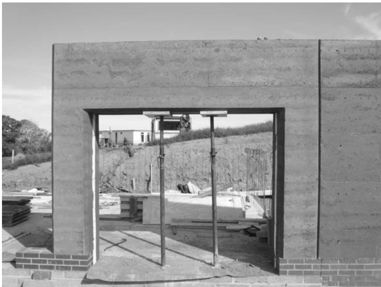
23.11 SRE wall with cage reinforced integrated lintel temporarily supported by telescopic props during curing, at Straightways Farm, Devon, UK (© Earth Structures Europe Ltd, 2007).
