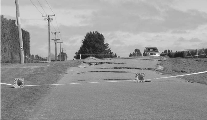
19.8 Earthquake fault trace displacements of about 1.5 m vertically and 4 m horizontally. Road previously straight and level, New Zealand 2010 (photo: M. Pender).
