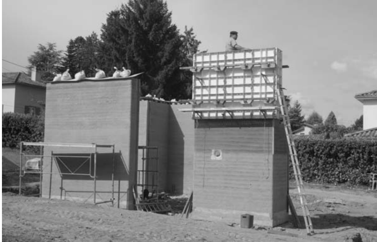
23.20 Use of vertical sliding formwork system during construction of the rammed earth walls at Chasselay (© Nicolas Meunier, 2011).
