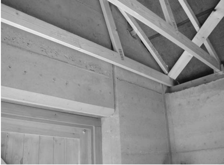
23.12 Steel lintel attached to the adjacent SRE walls using resin-bonded steel bolts on the stables building at The Manor, Ashley, UK (© M R Hall, 2002).
