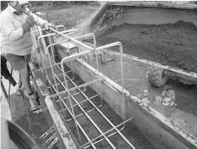
23.10 Stainless steel reinforcement cage used in conjunction with Stabilform™ formwork to produce an integrated SRE lintel, at Straightways Farm, Devon, UK (© Earth Structures Europe Ltd, 2007).
