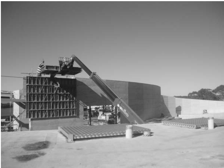
22.15 A telescopic handler delivers material to a 4.8-m-high wall. Telescopic handlers have been successfully used to deliver material to walls as high as 13 m.
