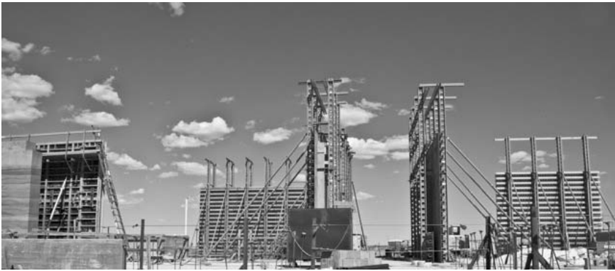
1.6 Multiple gang forms at Southeast Wyoming Welcome Center, Wyoming: in order to meet tight schedule timelines, it is useful to have multiple walls underway at different stages of the process, thereby keeping the forming team, the ramming team and the mixing teams busy at all times (© SIREWALL Inc., 2011).
