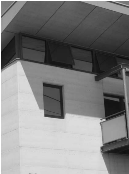
22.10 A typical SRE 'block-out' opening. Note the adjacent opening has a control joint alongside it.
