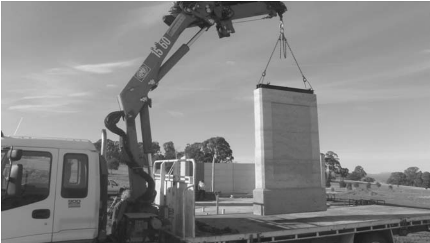
22.20 Transporting an elevated SRE panel. Note the concrete footing in this case is an integral part of the monolith. Mansfield, Victoria.
