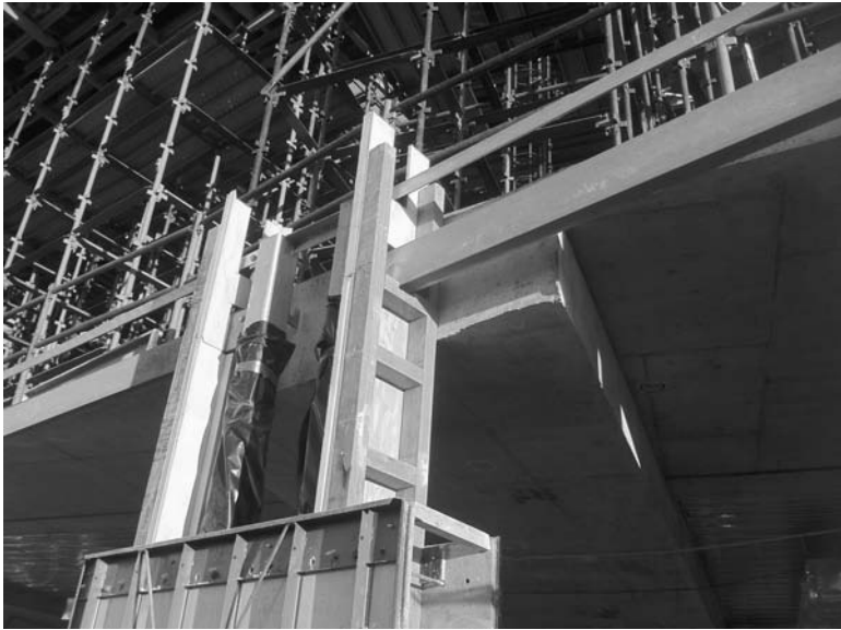
A1.1 Steel portal frame within cloister walls at the RACV project, Torquay.
