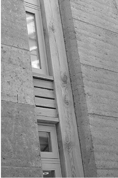
23.13 Glazed timber window frame attached and sealed to an unstabilised rammed earth wall at the Rivergreen Centre, Aykley Heads, UK (© Rivergreen Developments Plc – Developer/Contractor, photograph by Allan Mushen, 2006).
