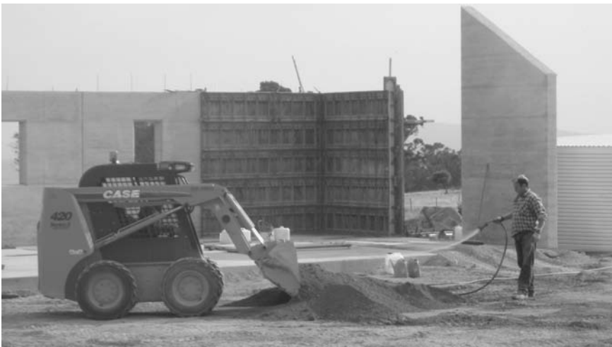
22.6 Blending and wetting the SRE material using a skidsteer loader. An average mix will take between 6 to 8 minutes to complete, including the blending of the Plasticure waterproofing admixture.
