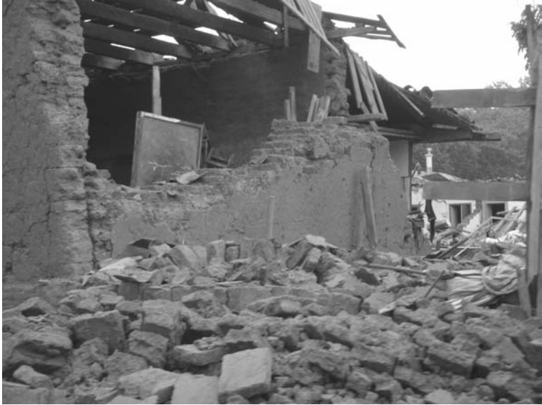
19.3 Out-of-plane wall failure of a house in Parral, Chile with no ceiling diaphragm, poor connection to the cross wall and lack of connection at the near corner. (photo: Exequiei Araos)
