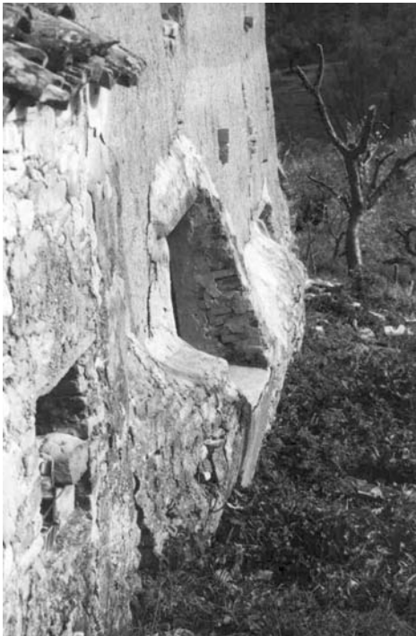
16.6 This is an example of an earth building that has been consolidated using concrete. The base of the building has rejected the concrete, and it in turn has rotated away from the earth wall. This is caused by severe erosion due to trapped moisture below the concrete itself.
