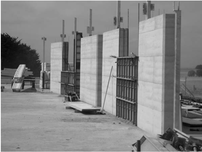
22.8 Placement of SRE formwork. Note the two consecutive 'set-ups' under construction by the one team. A team will typically build one or two complete panels per day.
