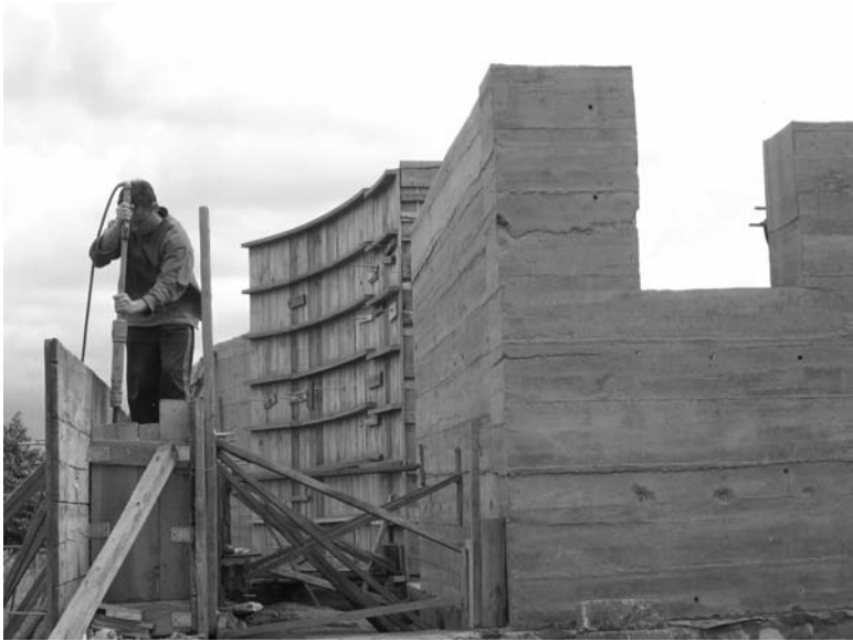
23.32 Pneumatic compaction of rammed earth walls, including a large curved section, at the Paştek experimental research house (© Teresa Kelm, 2008).
