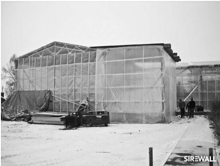
1.8 Sublette County Library, Wyoming: the heating and hoarding tent in the snow with air temperatures well below -30^{\circ}\text{C} (© SIREWALL Inc., 2011).
