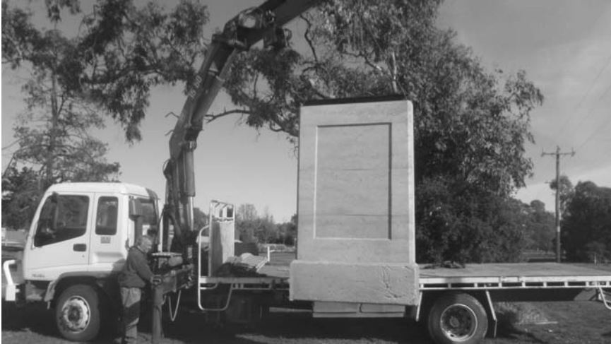
22.26 Lowering an elevated SRE panel into an excavated trench. The concrete footing sits 50 mm above the surrounding ground. Mansfield Shire sign wall, Mansfield, Victoria.
