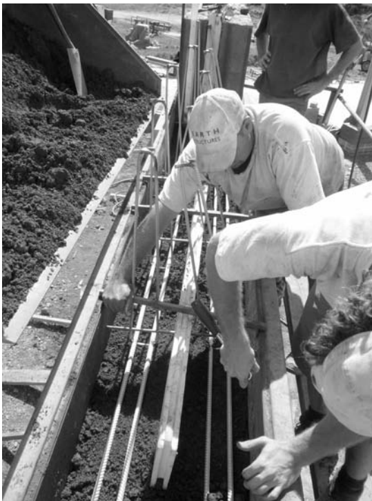
3.3 Interlocking extruded polystyrene insulation positioned in conjunction with stainless steel reinforcement in a structural SRE cavity wall (© Earth Structures Europe Ltd, 2007).
