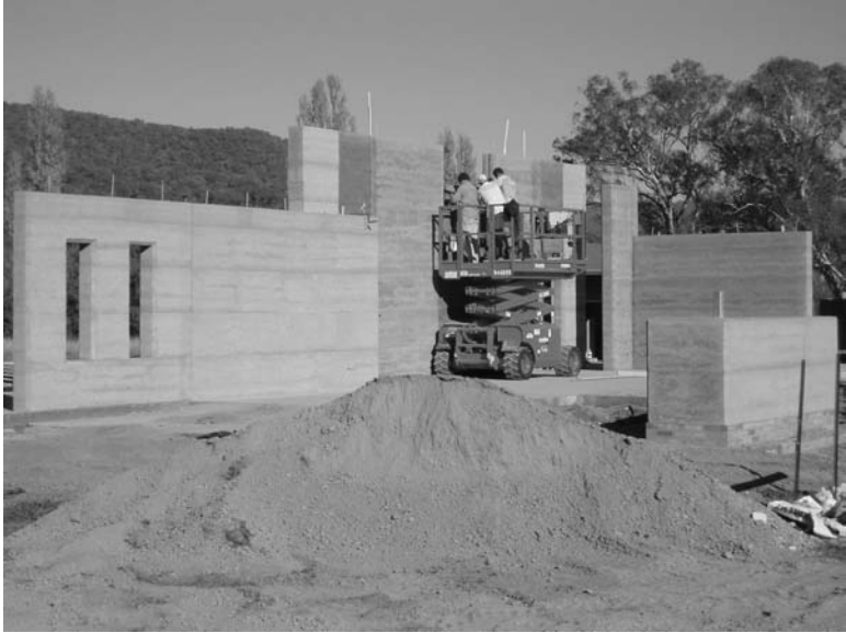
22.14 A scissor lift is used to elevate formwork and blended material to walls over 3.6 m height.
