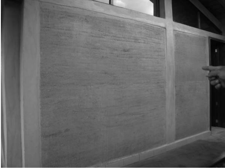
14.2 Panel to panel rammed earth construction using the California form. Finished rammed earth wall with concrete posts and bond beam.
