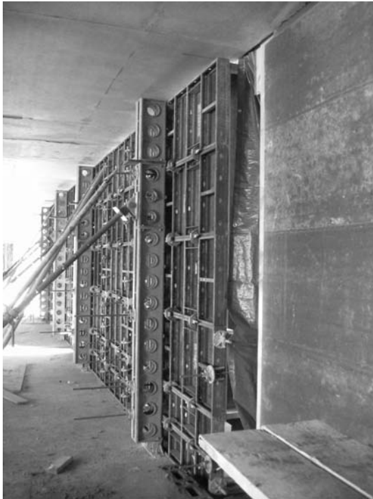
23.4 Lightweight formwork in use during construction of the 6-m unstabilised internal rammed earth wall at the Rivergreen centre, Aykley Heads, near Durham, UK (© Paul Jaquin, 2005).
