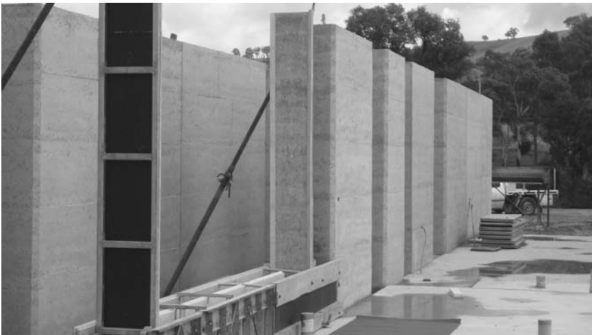
22.16 An insulated wall set up and ready for ramming. Note the material used for this project was a blend of recycled concrete and local aggregate resulting in a very low embodied energy. Berkeley residence, Thornton Victoria.
