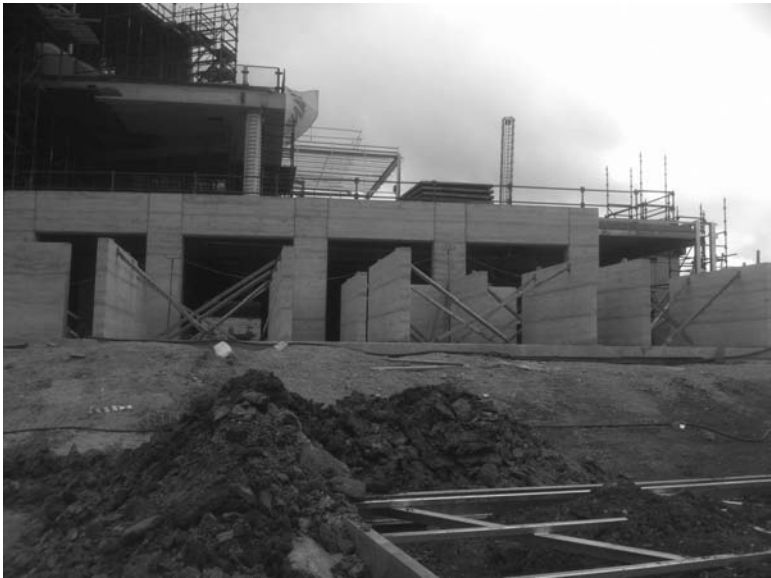
1.2 RACV Project, Torquay, Australia. Precast SRE panels ready for hoisting to Level Three. Cloister walls in background (© Earth Structures Pty Ltd, 2011).
