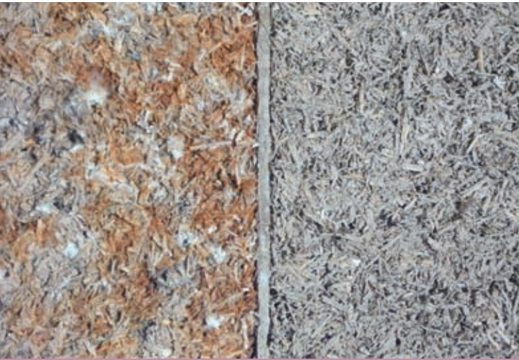
Hempcrete made with newly developed binder next to a neighbouring wall cast at the same time using a proper hempcrete binder.
