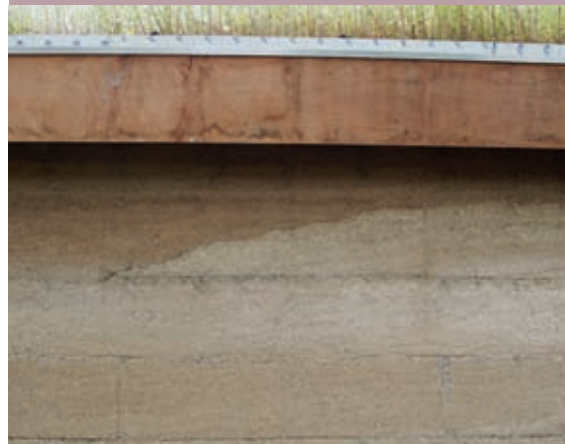
Hempcrete wall showing lines left by shuttering lifts, and a gently sloping day joint.
