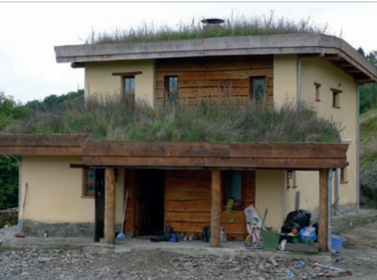
A truly 'zero-carbon' building, built from cob (mixed from clay dug on-site), hempcrete and timber. The embodied energy associated with this family home is much lower than that for a conventional building.
