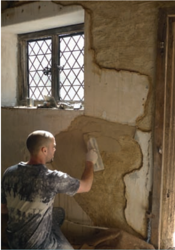
With skill and patience, lime plasters can be repaired selectively in historic work by patching in new plaster to the old, retaining the areas that were still sound.
