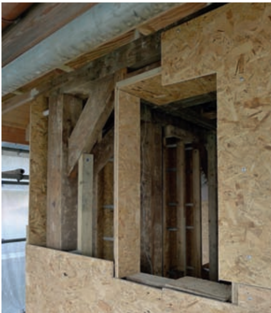
The shuttering boards used to form the window reveals are fixed to the framework for the window.
