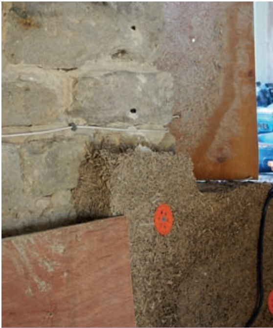
Hempcrete cast as solid-wall insulation internally fits neatly into the uneven surface of the stone wall.
