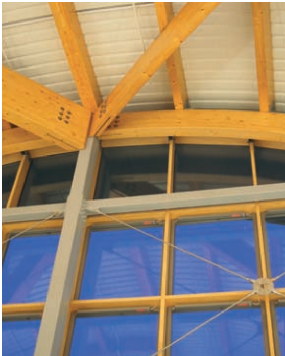
Steel and glulam interact in the frame of a large superstore built using Lime Technology's Hembuild® panels.
