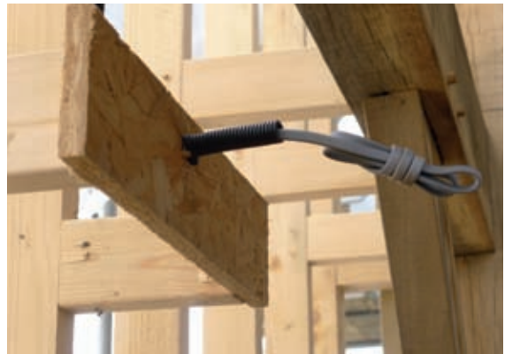
Wiring for wall lights is run through timber supports, which also provide a solid background for the light fitting to fix into.
