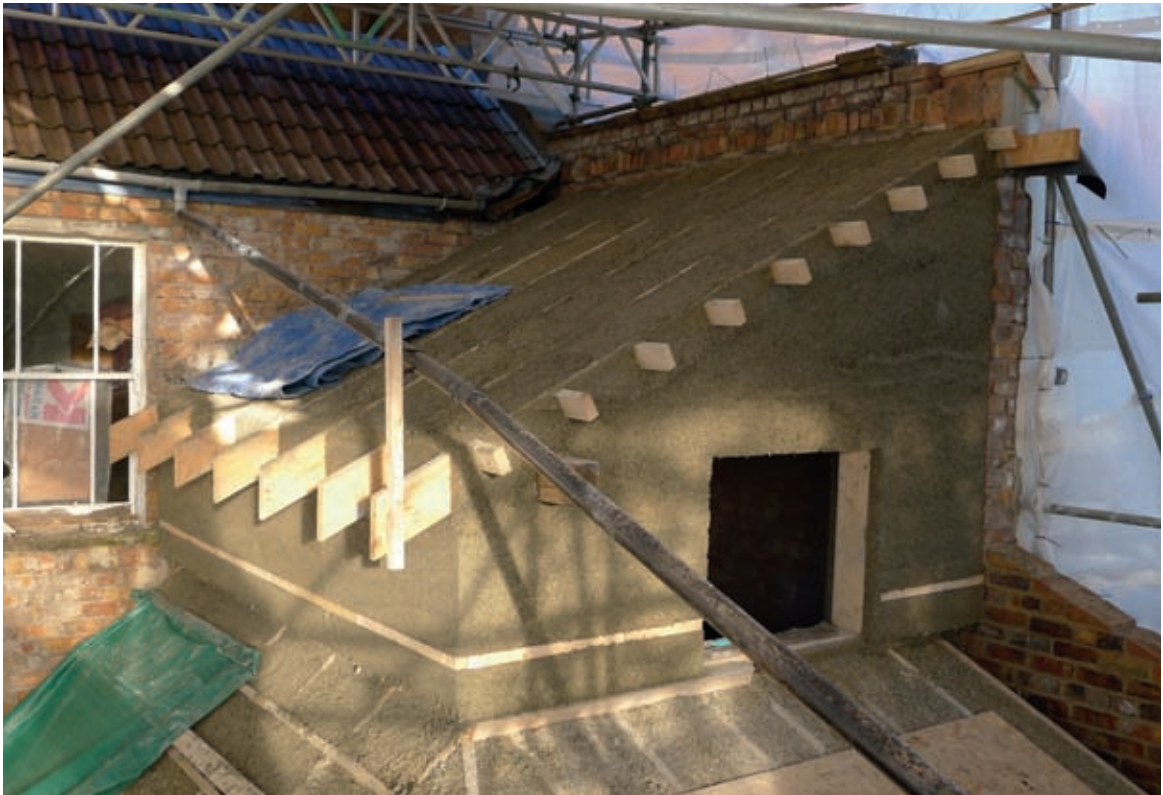
A cascade of hempcrete roofs. Note the visible difference in density between the roofing hempcrete and the walling hempcrete.
