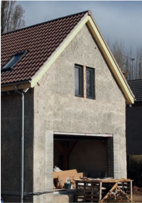
300mm walls of cast-in-situ hempcrete easily achieve the thermal performance required for a new building.
