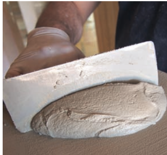
'Knocking up' a manageable amount of plaster on the hawk (by pushing it back and forth with a trowel until it forms a single consistent lump).
