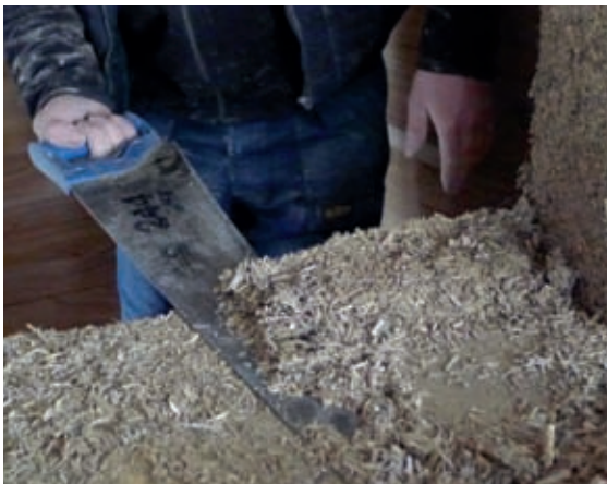
Hempcrete is over-filled at windows and then cut back with a saw so there is solid hempcrete immediately under the window.
