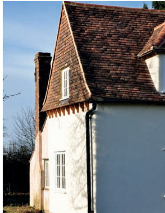
Hung-tile cladding provides extra protection to this exposed hempcrete gable. This replicates the original gable detail in this listed timber-frame cottage.
