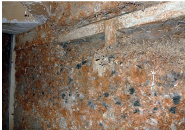
Hempcrete wall made with a newly developed (and insufficiently tested) binder, two months after casting.
