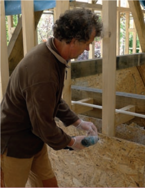
Fixing shuttering to an exposed frame is much easier than with a central frame.
