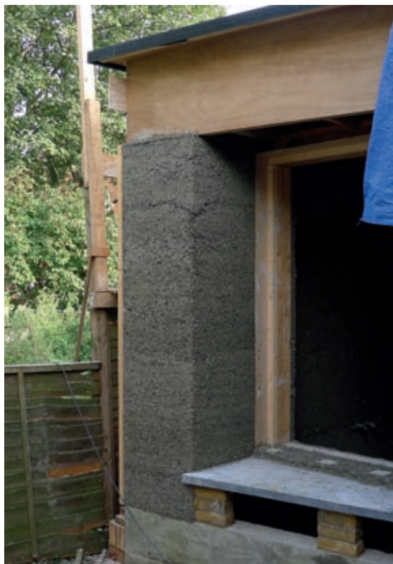
A monolithic wall made from timber and hempcrete replaces many different materials that are required in a conventional modern wall build-up, e.g. bricks, blocks, cavity insulation, membranes and wall ties.
