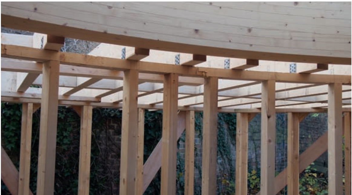
Untreated softwood and glulam beam making up the frame for a hempcrete wall.
