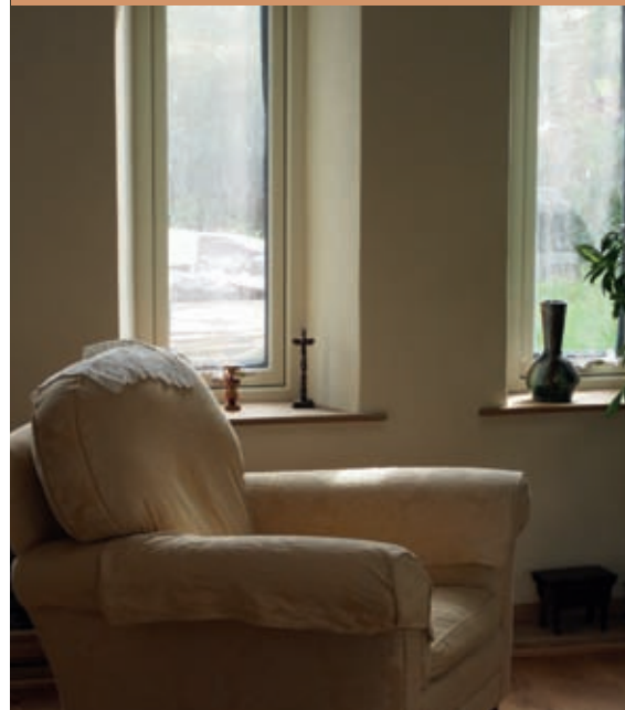
Angled window reveals are attractive within a deep hempcrete wall and maximize the amount of light.
