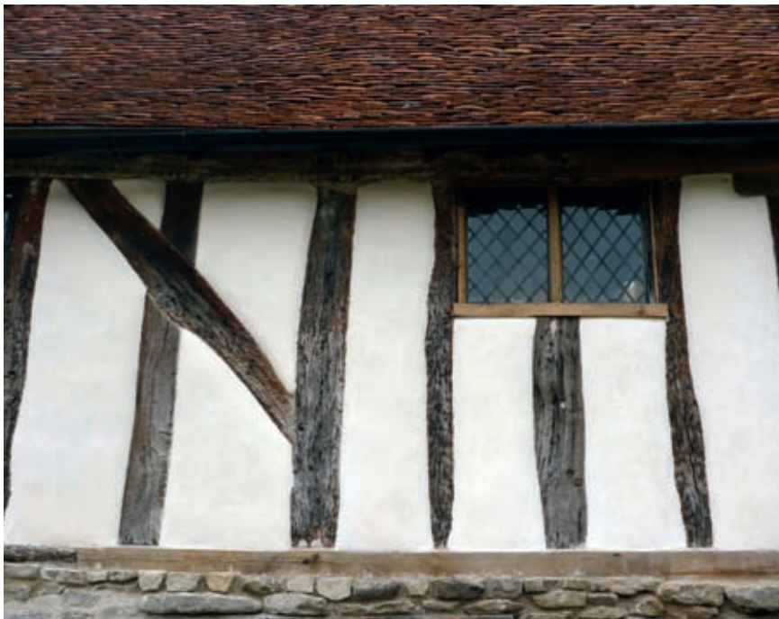
Shuttering and casting around ancient timber frames, such as in this Tudor barn, can be a slow business.
