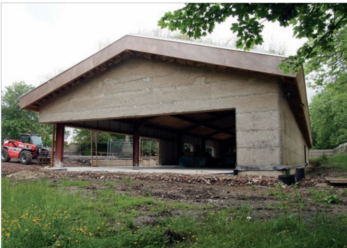
This new-build community centre, cast during an exceptionally wet summer using a slow-setting binder, was rendered a year after the hempcrete was cast.
