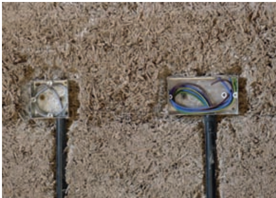
If necessary, electrical cables and other fittings can be chased into the hempcrete after it has set.
