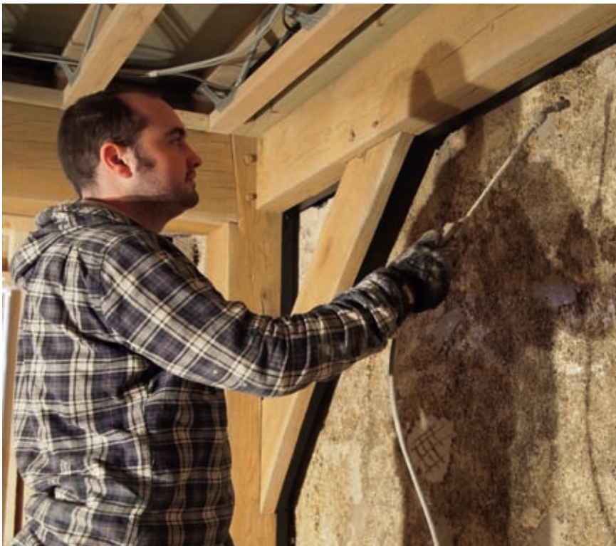
Wetting down hempcrete to ensure the correct level of suction (see box overleaf) before applying a basecoat plaster.
