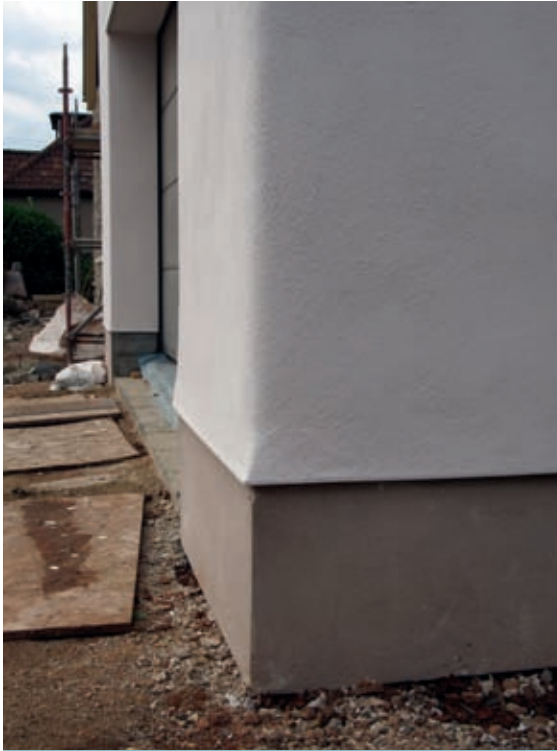
A drip detail incorporated into the bottom of the render stops water from running down the plinth.
