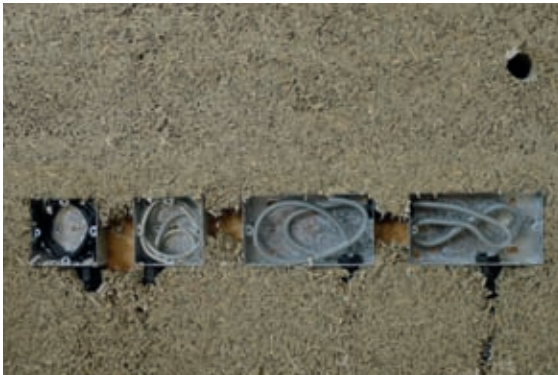
Back boxes are fixed to timber supports so that they sit flush with the face of the wall.
