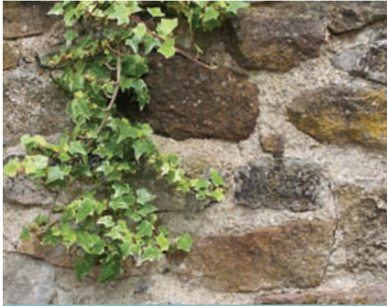
A moderately hydraulic lime mortar is used for pointing in this wall, since the stone is very hard. For softer masonry, an air lime mortar would be appropriate.
