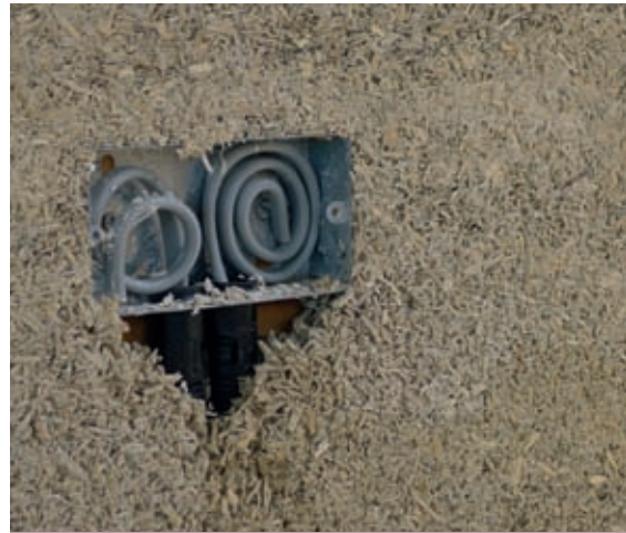
Any unfilled voids in the wall such as this, under the back boxes, can be filled in afterwards.
