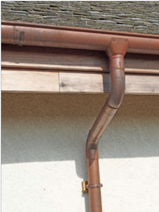
Copper rainwater goods on a hempcrete house: a robust and attractive solution.
