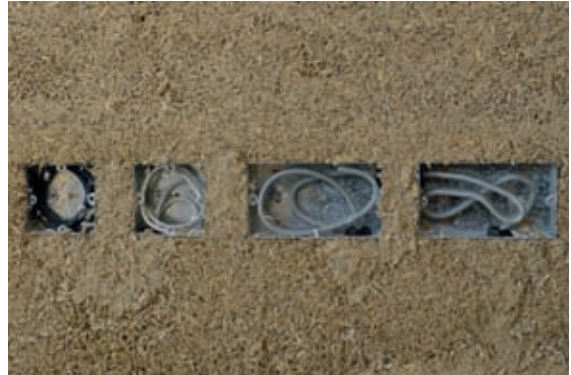
Any holes around fittings can be filled by hand after the wall has been cast.
