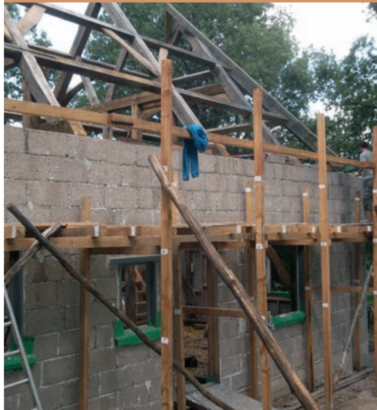
Hempcrete blocks in a new-build house under construction. (Note: the timber structure in the foreground is wooden scaffolding, not part of the frame!)
