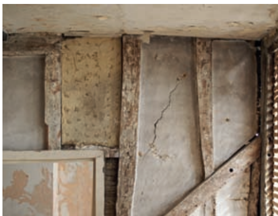
Hempcrete is the perfect material for repairing and increasing the thermal performance of ancient timber-frame buildings, due to its hygroscopic properties.
