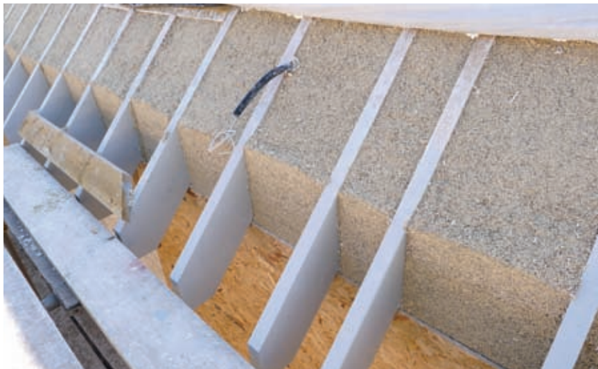
Hempcrete at the eaves of a building: the waterproof roof membrane is in place but can be rolled back to allow the hempcrete to be placed.
