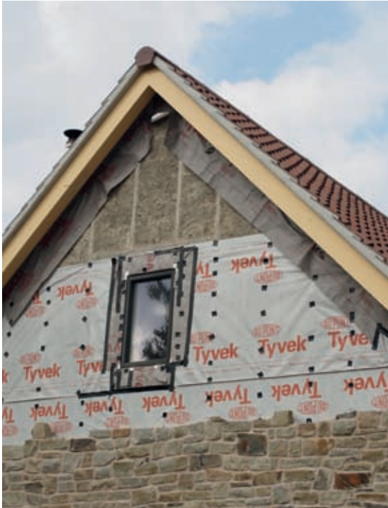
Masonry cladding on a hempcrete building. Note the external frame enabling the cladding to be tied in to the wall, and the vapour-permeable membrane.
