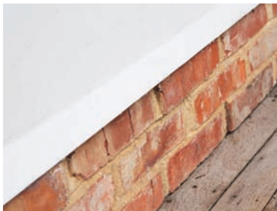
Plinths can be more sustainable than a concrete upstand with cement render, as shown by this plinth made from reclaimed brick and lime render.
