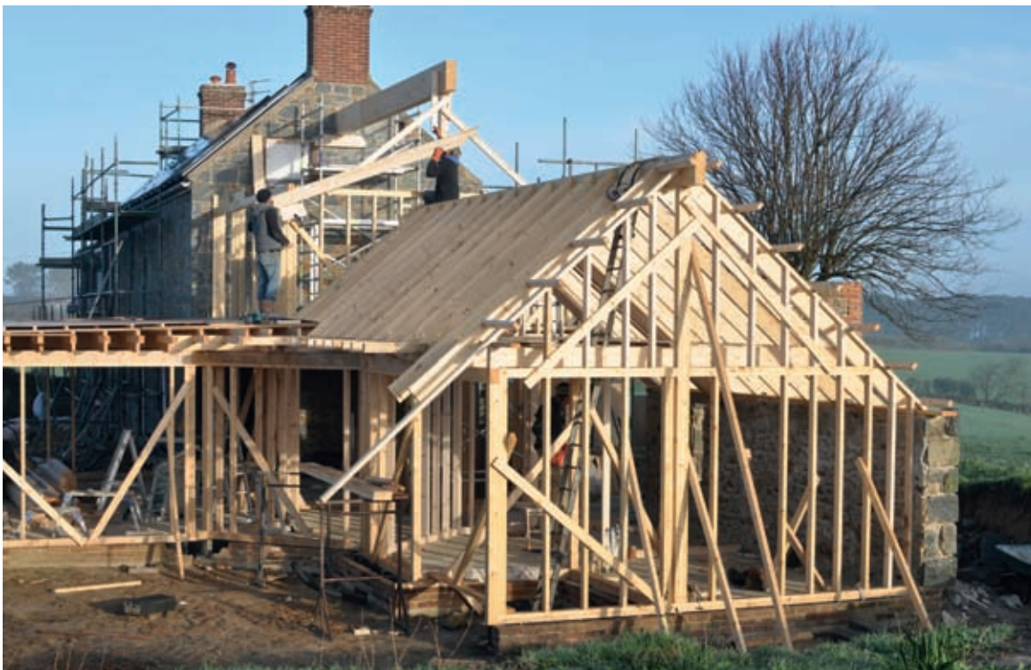
The structural frame for a new-build hempcrete extension. Note the glulam ridge beam and temporary bracing put in place to support the frame while it is being built.
