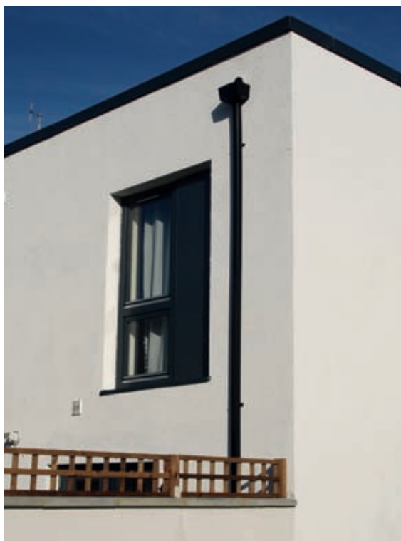
A large eaves overhang is not always necessary on hempcrete buildings: at Callowlands in Watford, a hidden gutter and a specialist hydrophobic lime-based render allow the overhang to be eliminated.
