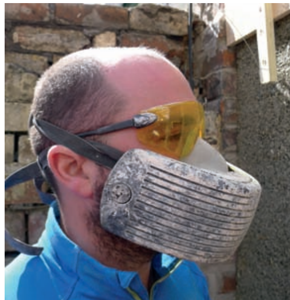
Goggles and a high-quality P2 dust mask are essential when mixing hempcrete.
