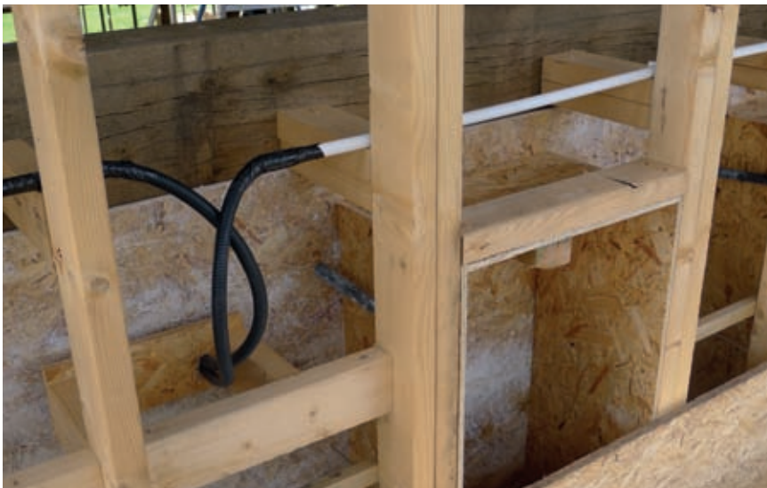
Conduit and cables are run in the wall before the hempcrete is cast.
