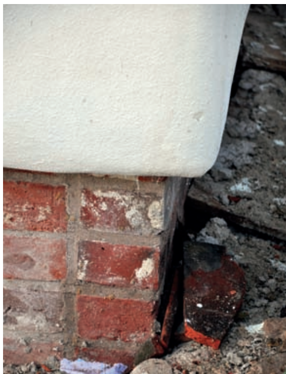
A brick plinth for a hempcrete wall in a listed building. The bottom of the render curves in towards the wall, disguising an unusual hidden drip detail, included to meet conservation aesthetics requirements.
