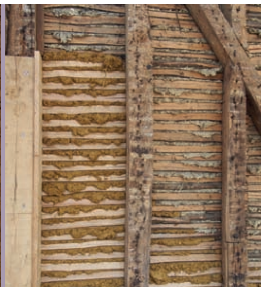
The same repair from the back, before hempcrete is cast around the frame from outside.
