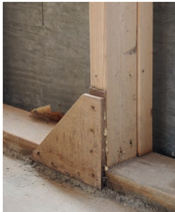
A plywood gusset used to replace a metal angle bracket as a frame fixing.
