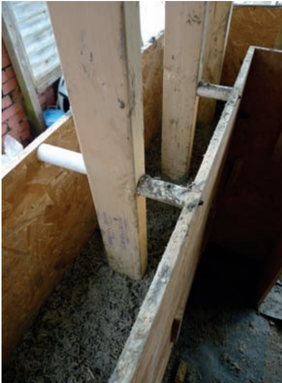
A softwood frame buried centrally in the wall is the standard design.
