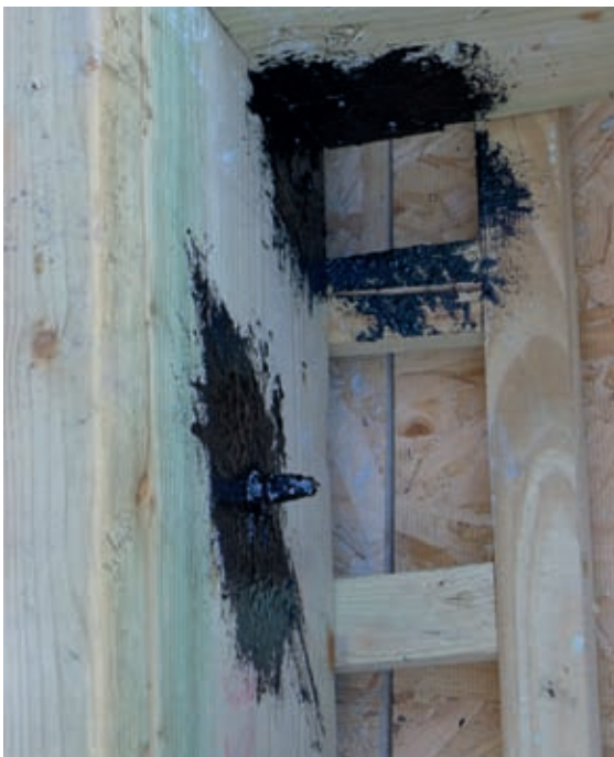
Steel fixings in contact with hempcrete should be painted with a protective coating.
