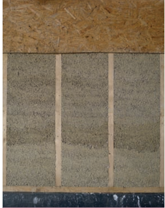
Shuttering partially removed from a section of wall with an exposed frame.
