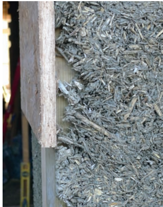
Casting hempcrete at less than 50mm coverage over timbers causes weak spots.
