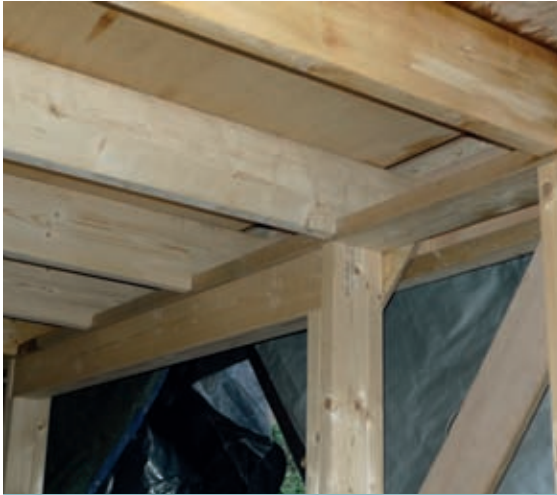
Rafters bearing on the wall plate and fixed down from above with long screws, to avoid fixings coming into contact with the hempcrete.
