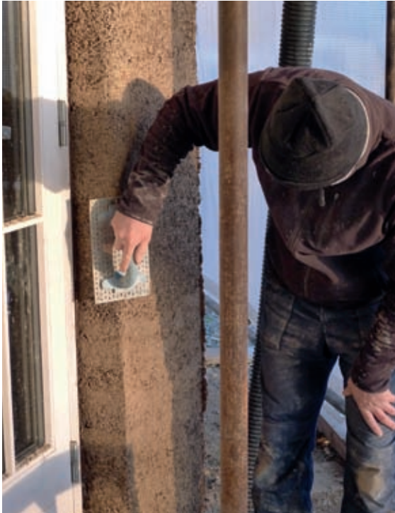
Before it sets hard, hempcrete can easily be shaped using a nail float. Here the sharp corners are rounded off to give softer lines to the building.
