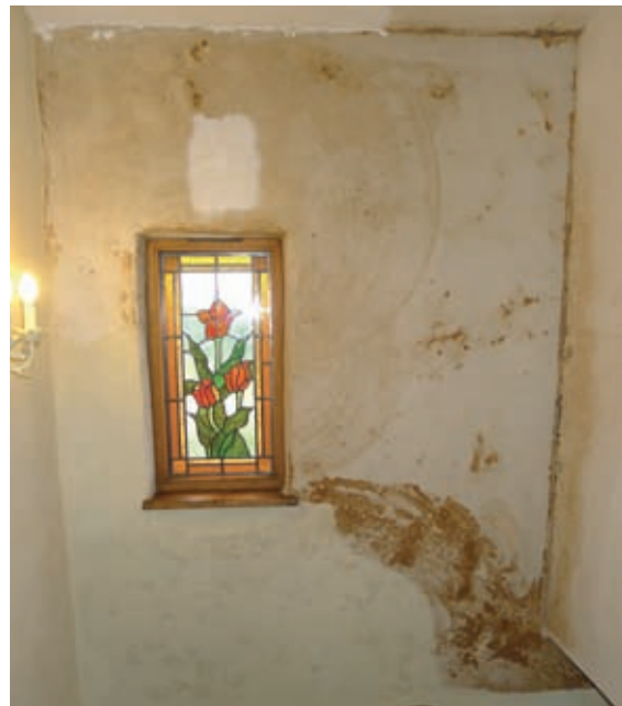
An extreme case of staining on plaster as a result of finishes being applied too early.
