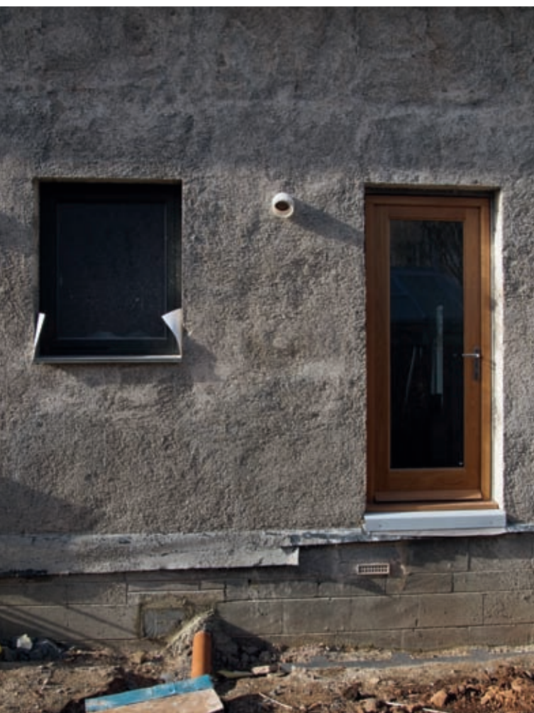
A good-sized plinth keeps the hempcrete wall in this new-build house well above ground level.
