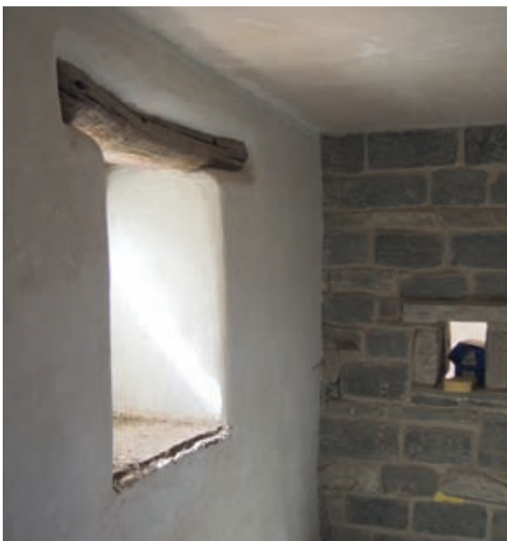
Hempcrete solid-wall insulation at a thickness of 70-100mm, with lime plaster applied.
