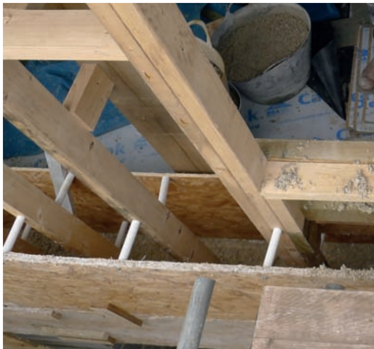
Design the frame so that shuttering spacers are the same length on both sides.
