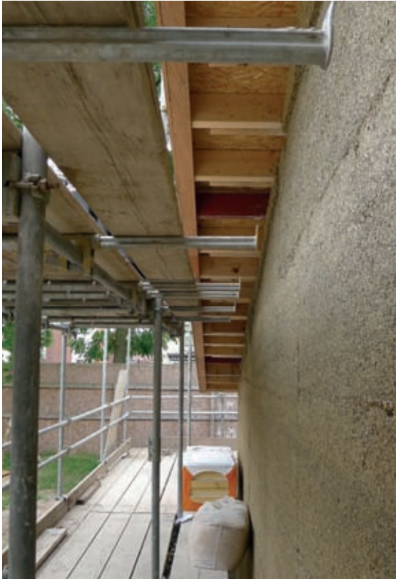
Ensure that horizontal scaffolding poles are not too close to the wall to prevent shuttering being moved.
