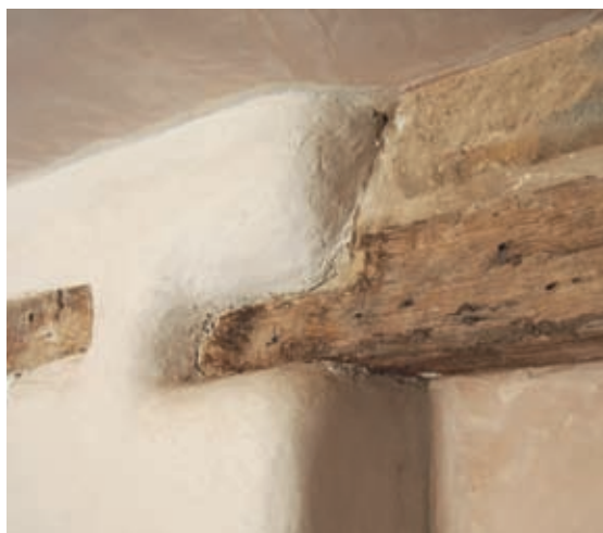
A ‘rough’ lime plaster applied by a novice can still be an attractive finish.
