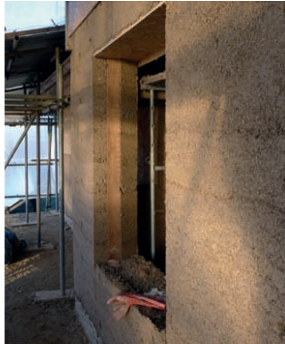
The framework for a window is left flush with the surface inside the reveal to provide a fix for the window frame.
