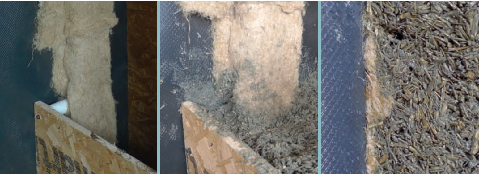
Using hemp-fibre insulation to create airtightness at a junction between hempcrete and an existing wall.
