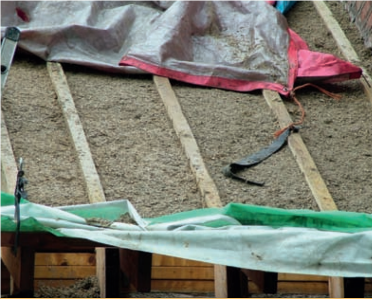
Keeping the work dry can be a challenge when casting roof insulation. Image: Margot Voase
