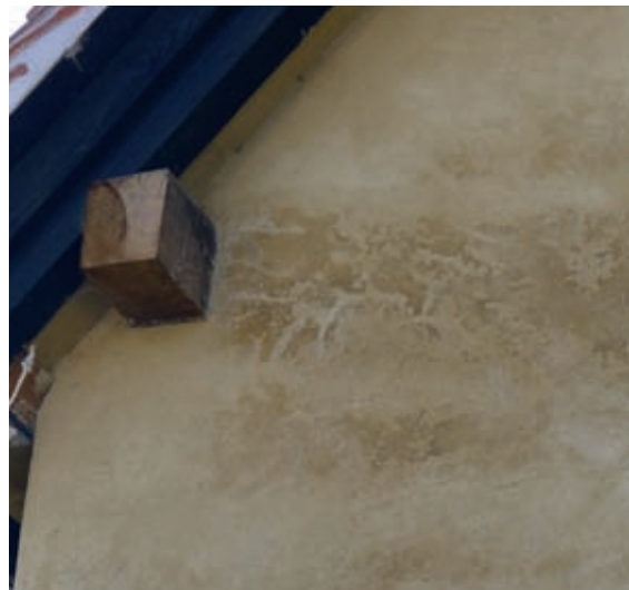
Render applied too early: dark patches show where liquid water is drying through the render.
