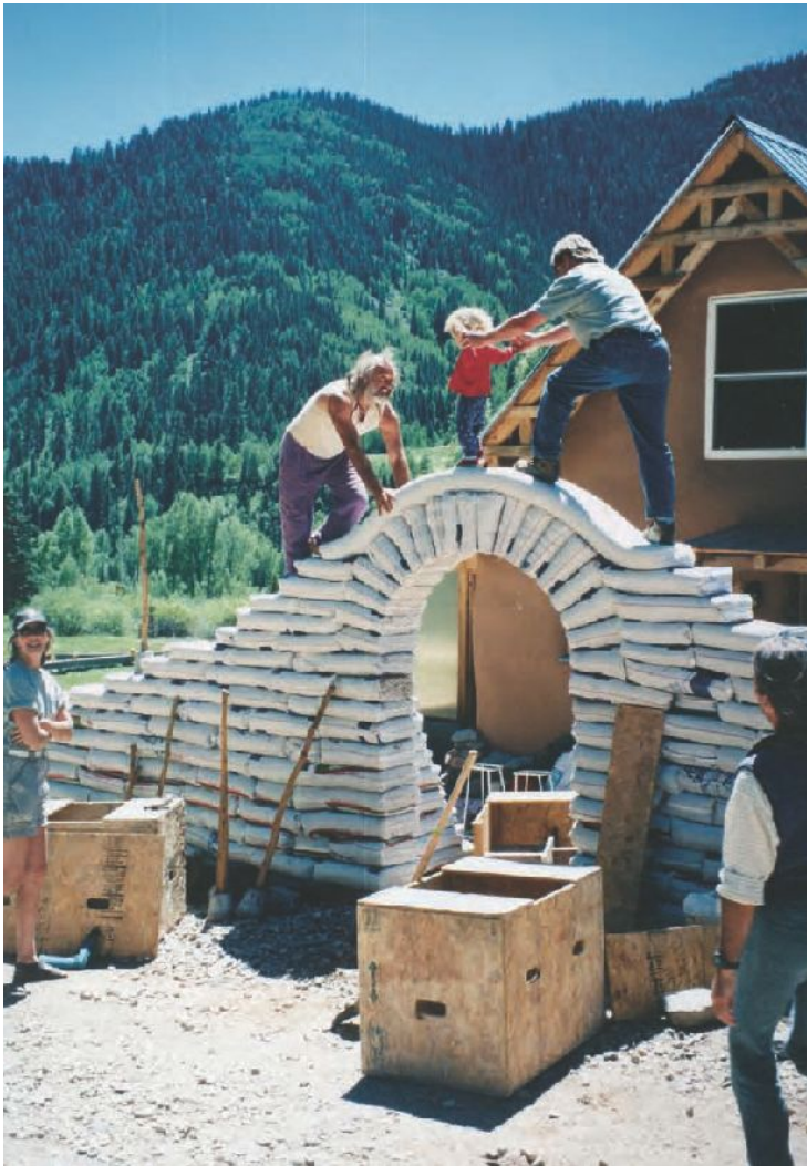
This freshly laid Earthbag wall was constructed in a weekend at the 1999 Colorado Natural Building Workshop held in Rico, Colorado (Fig.1, left).
