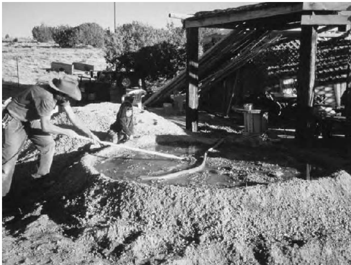
2.9: In some cases where water is a precious resource or needs to be hauled to the building site, the earth can be flooded and held in check by tending little dams, allowing it to percolate overnight.
