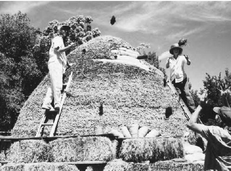
13.2: For a water-resistant earthen-base plaster, we increase the percentage of clay to sandy soil, pack it full of long straw, knead it into hefty loaves, and smack them onto the dome.
