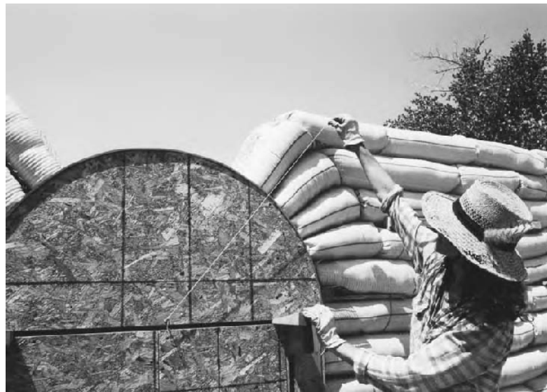
10.8: The attached stringline assists as a visual aid in determining the appropriate angle to shape the fan bags.
