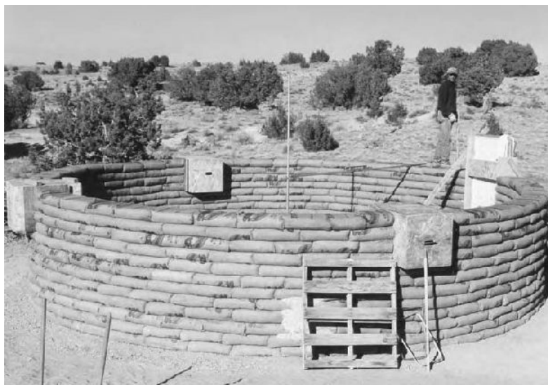
2.14: Burlap bags have a nice organic look that can be appreciated during construction.
