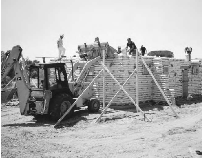
3.35: A five- to seven-person team built the 9'6" tall walls for this 750 sq. ft. Bureau of Land Management Ranger Station in eight days.
