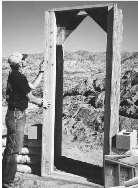
2.25: An open, mine-shaft style form allows easy access to the inside of a building without climbing over the wall during construction.
