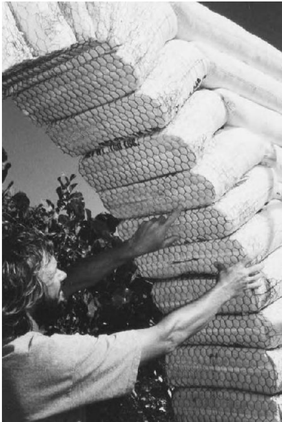
2.34: Cradles provide the underside of arches with an extra grippy surface for the later application of plaster.
