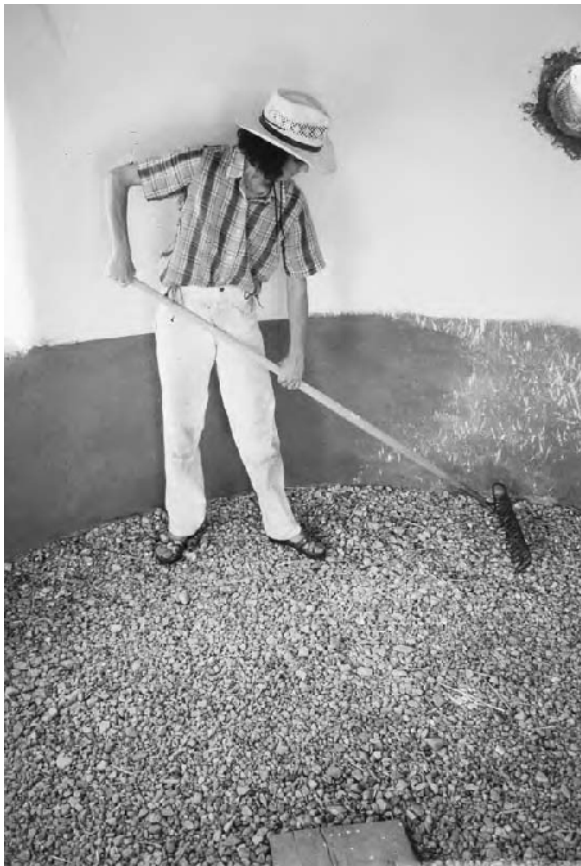
16.3: Rake this gravel out level and the lowest layer of your earthen floor is done.
