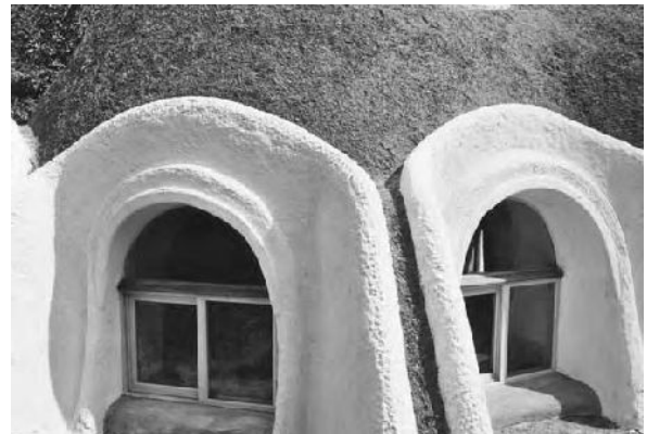
13.3: The vertical faces of our Honey House are protected with lime plaster, and the exterior windowsills are made of lime-stabilized earth. Both applications have held up very well for five years.
