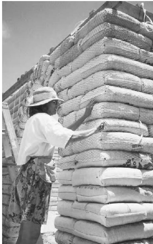
14.20: Carol Escott cinches up chicken wire with a combination of tie wires and nails. Photo Credit: Sustainable Systems Support.
