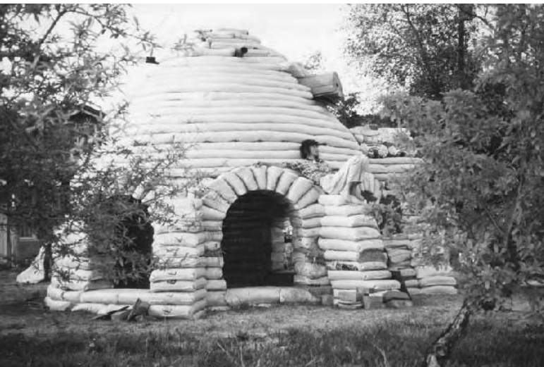
12.33: The completed bag work of the Honey House after removal of the forms.
