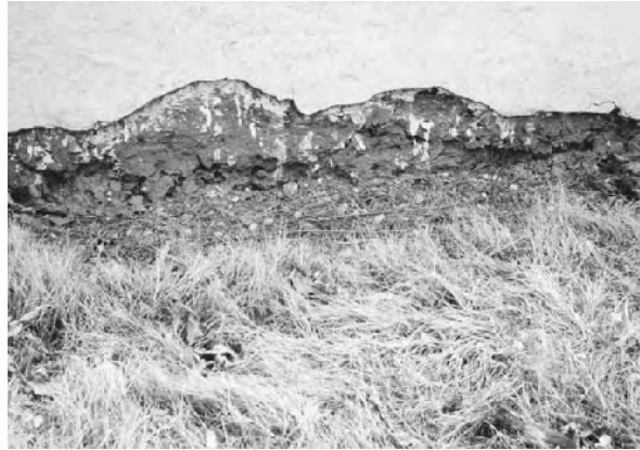
4.11 (above): Plastering down to ground level risks wicking moisture into the walls, causing spalling and other moisture-related damage.
