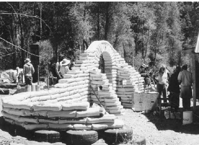
4.13: Tire foundation/ stem wall used to support an earthbag wall at Colorado Natural Building Workshop in Rico, Colorado.
