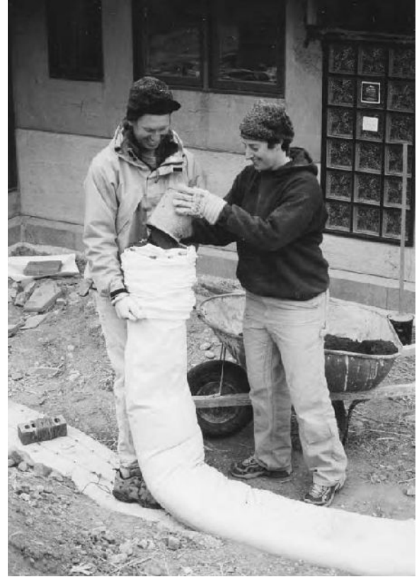
3.24: A tube chute acts as a sleeve to scrunch a length of tube onto, as well as a funnel that the dirt is fed into.
