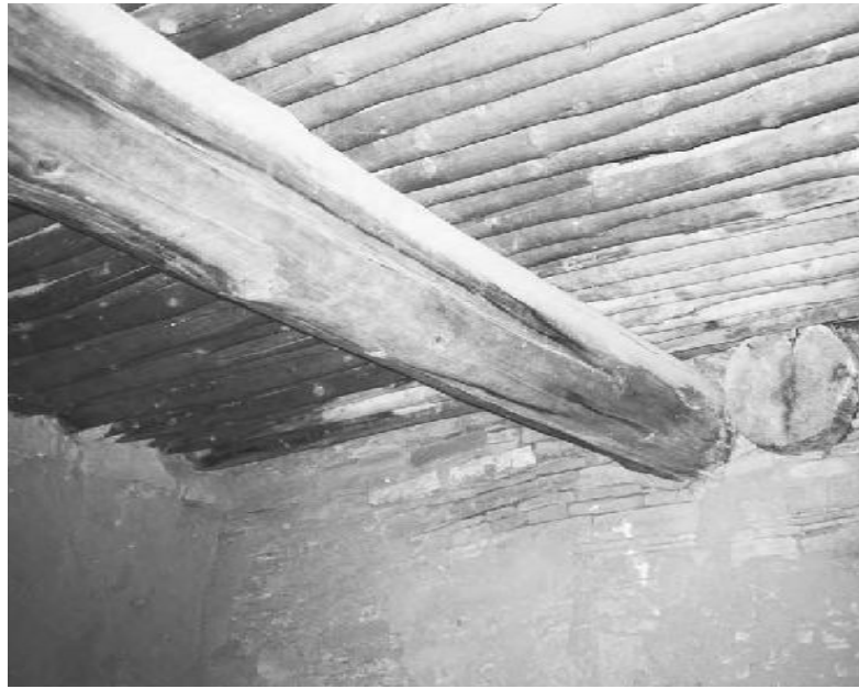
9.9: This Anasazi structure in Chaco Canyon, New Mexico, shows the original vigas and latillas sitting on stone and mud walls, still intact after 1,000 years. Will a modern tract house ever get to make this claim?
