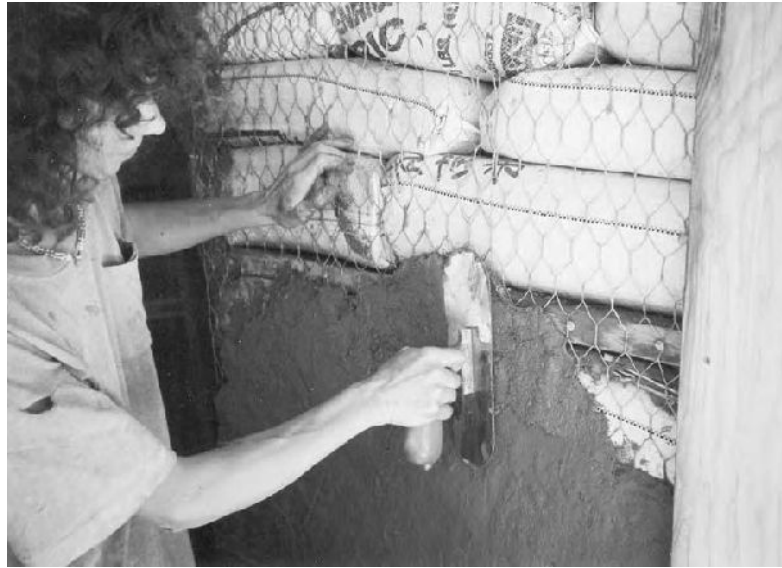
15.5: Fiber-free plaster goes on quickly, and deeply fills all the voids between the rows of bags until the plaster comes flush with the wire.
