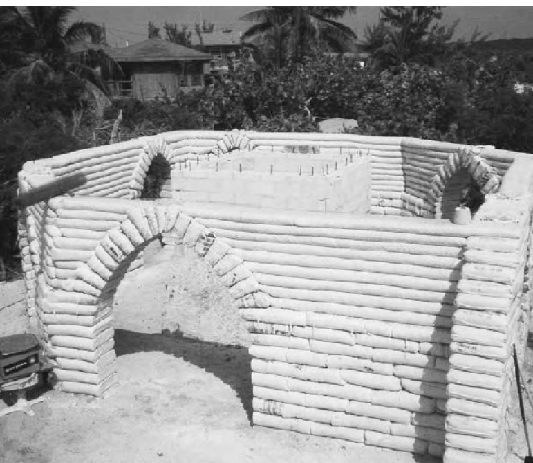
2.13: The 100-lb. and way-too-big bags can also be used to surround the window and doorways in conjunction with the narrower 50-lb. bags/tubes for the walls.
