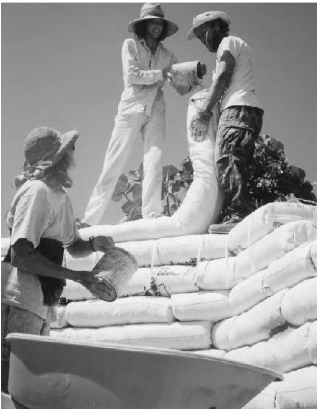
3.29: The person holding the chute is the "walking bag stand," while the "tube loader" fills the chute and the third person delivers dirt and feeds cans to the loader.
