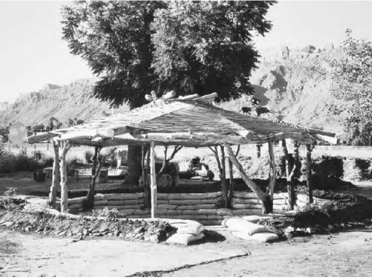
9.25: Inspired by the reciprocal roof, Jason Glick designed this fanciful gazebo lined with a sunken earthbag seating area for the Youth Garden Project in Moab, Utah.
