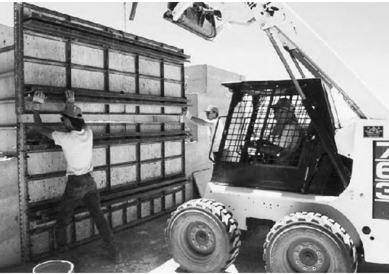
1.5: The entire form box can be set in place using the Bobcat. Steel whalers keep forms true and plumb and resist ramming pressure.
