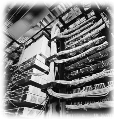
FIGURE 18.4 Lucent SYSTIMAX GigaSPEED Installation, rear angle view of patch-panel rack. (Copyright © 1999, Lucent Technologies, used by permission.)
