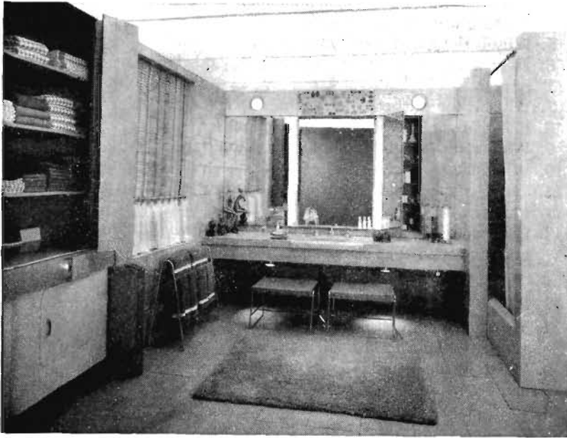
Fig. 37.14. This bathroom has a completely lighted ceiling. Fluorescent tubes are concealed by a translucent ceiling. The mirror is surrounded with fluorescent tubes concealed by frosted glass panels. (Courtesy General Electric Company)
