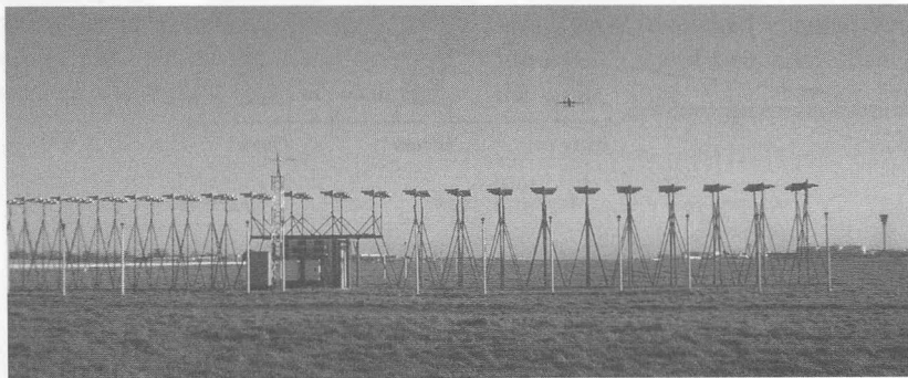
(c) Localizer antenna (viewed down the runway)
