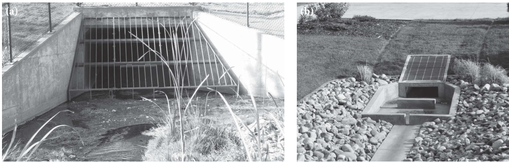
Figure 15.1 Examples of rack and grate. (a) Rack in front of box culvert and (b) inclined grate on inflow conduit.
