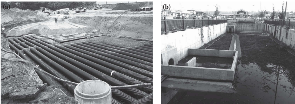
Figure 13.23 Underground detention basin. (a) Sump intake and (b) pipes for storage volume.
