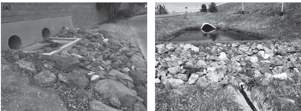
Figure 11.5 Erosion protection at culvert exit. (a) Riprap protection and (b) plunging pool.
