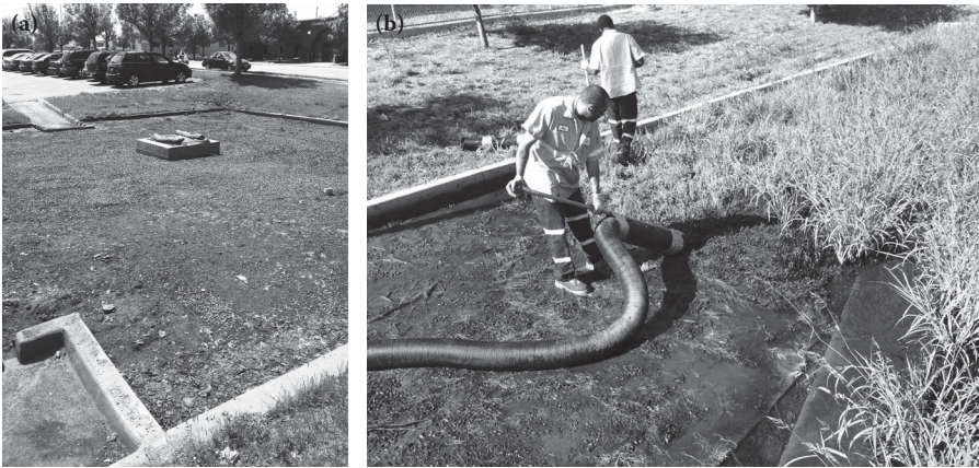
Figure 17.19 Repair of clogged porous bed. (a) Plugged porous bed ( f < 1 in./h) and (b) vacuum clean to remove cake layer.
