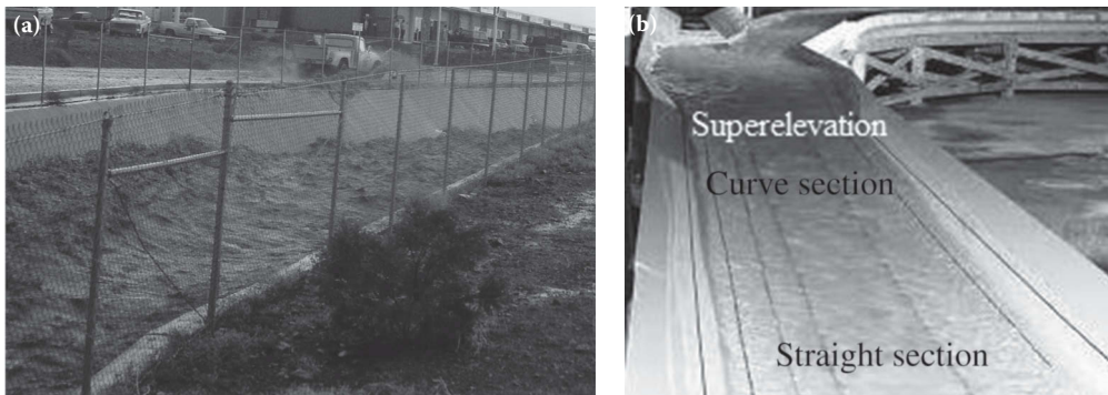
Figure 8.6 Superelevation in concrete curve channel. (a) Superelevation at bank and (b) superelevation in laboratory.
