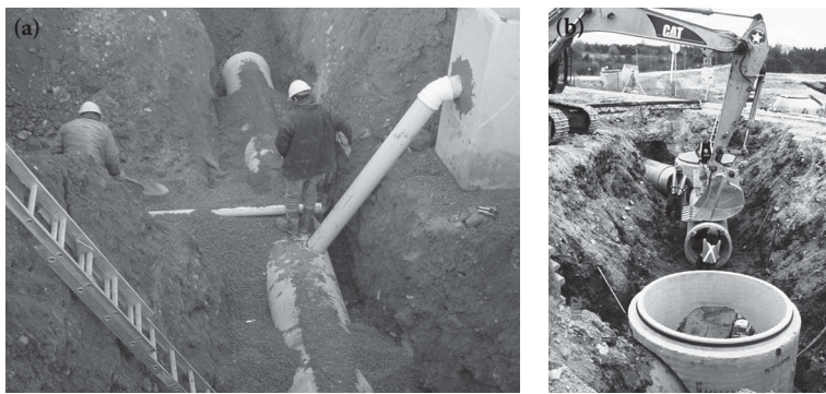
Figure 12.4 Laterals in sewer system. (a) Inlet connected to sewer line and (b) manhole on sewer line.
