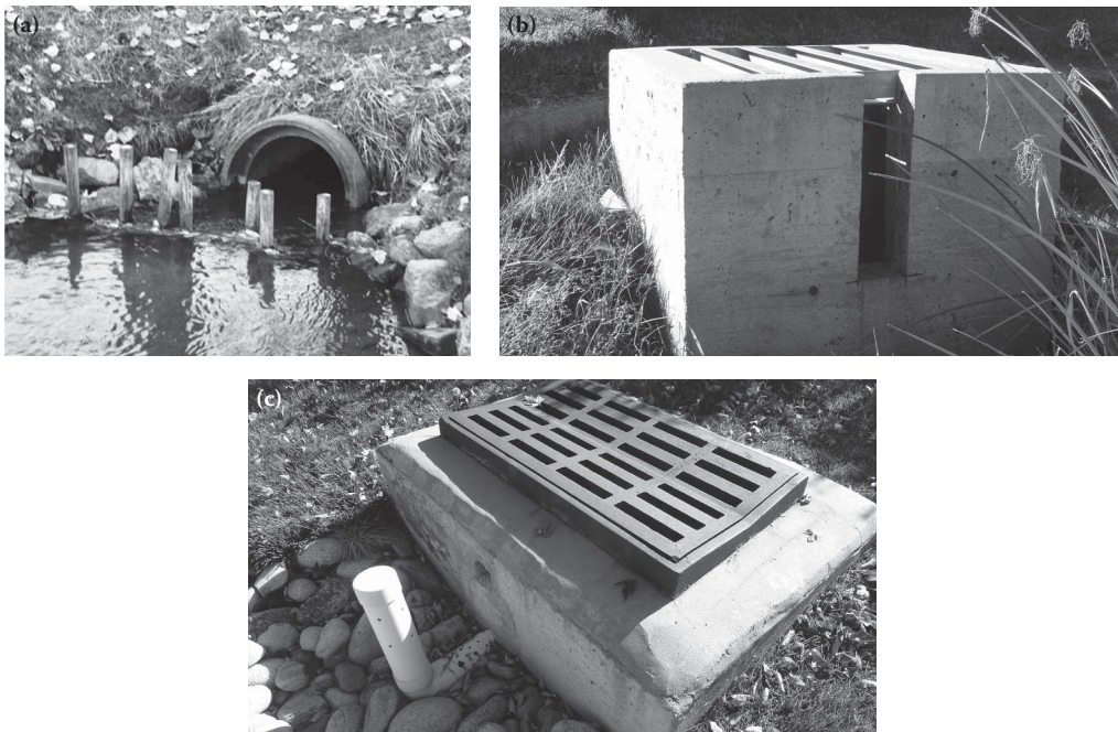
Figure 13.26 Outlet box to control flow releases. (a) Orifice only, (b) orifice and weir, and (c) orifice, weir, and riser.
