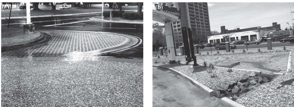
Figure 17.5 Receiving porous areas. (a) Structured porous pavement and (b) sandy infiltration bed.
