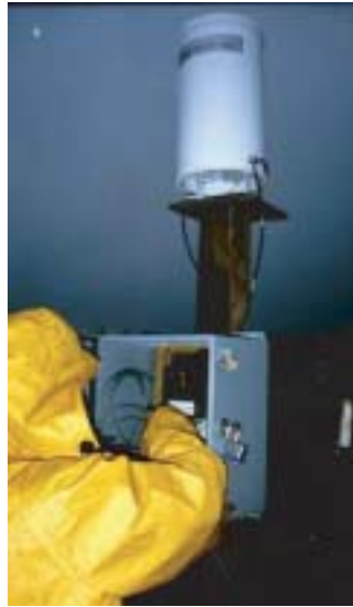
Figure 6.20 Tipping bucket rain gauge with data logger.
