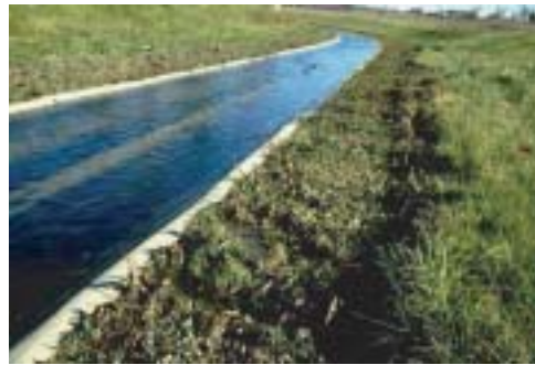
Figure 3.9 Lined channel in Milwaukee, WI.
