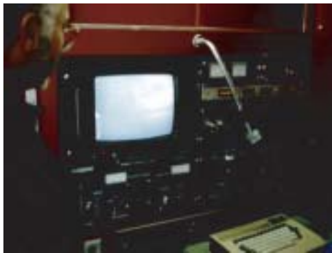
Figure 6.116 Remotely operated TV camera surveys of storm sewers in Boston to locate inappropriate discharges.
