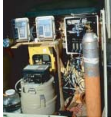
Figure 5.17 ISCO sampler used in instrument shelter with flow monitoring and telemetry equipment in Madison, WI.
