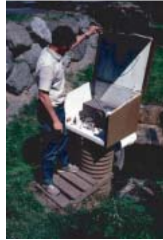
Figure 4.20 Level recorder at Bellevue flow monitoring station.
