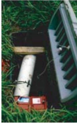
Figure 6.17 Acoustic flowmeter at USGS test site.
