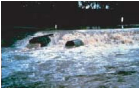
Figure 4.5 High flows in Coyote Creek overflowing road culvert.
