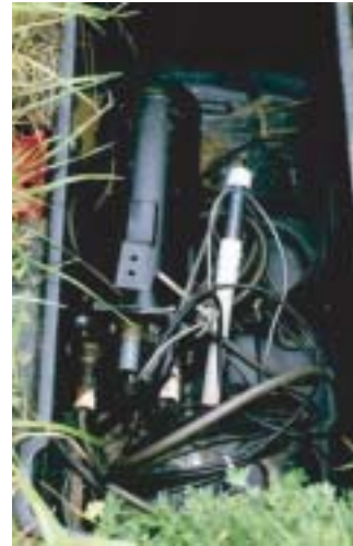
Figure 6.16 ADS acoustic flowmeter at USGS test site.
