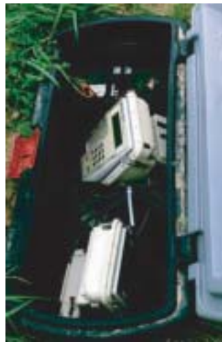
Figure 6.15 Sigma bubbler flowmeter at USGS test site.
