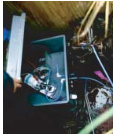
Figure 6.18 Automatic dye injection installation at USGS flowmeter test site.
