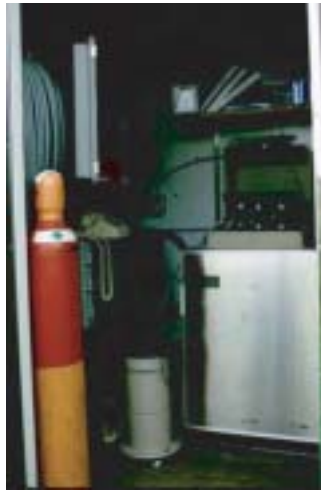
Figure 5.20 Refrigerated automatic sampler in Madison, WI, instrument shelter.
