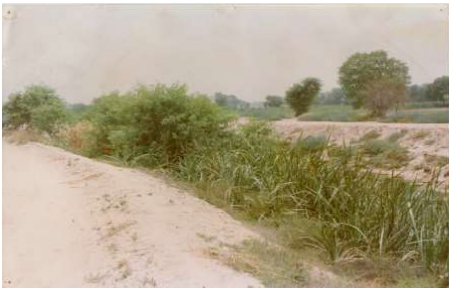
Fig.7.6c Unmaintained Open Drain at FDP, Faisalabad, Pakistan
