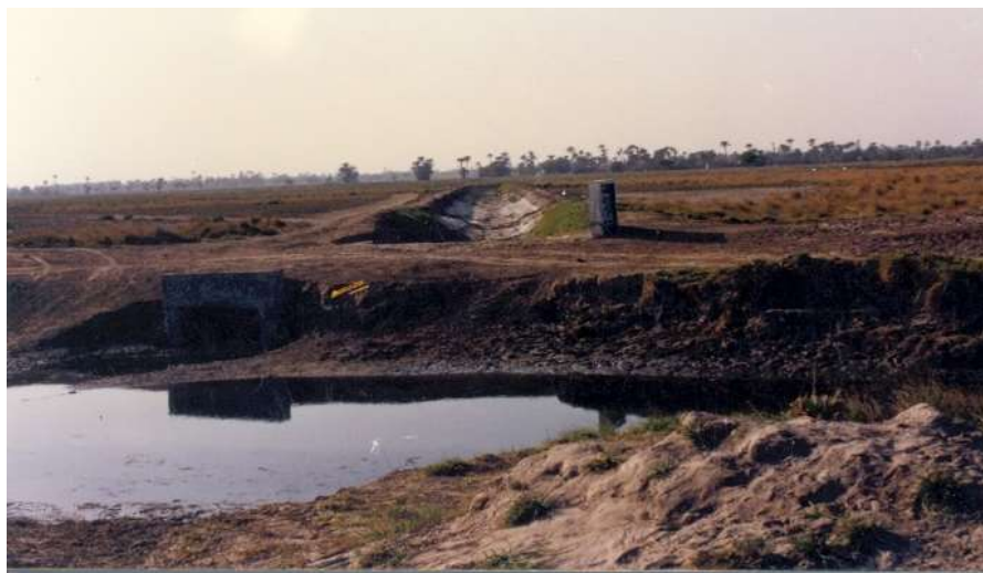
Fig. 7.7 Bank Erosion at Kot Adhu Surface Drain, Khan Garh, Distt. Muzaffer Garh, Pakistan
