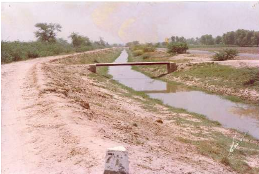
Fig. 7.3 A Well Maintained Surface Drain at FDP Faisalabad, Pakistan
