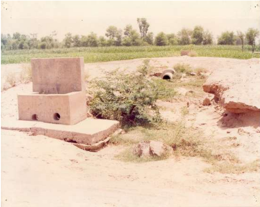
Fig.7.6b Bank Erosion in Surface Drain at FDP Faisalabad, Pakistan
