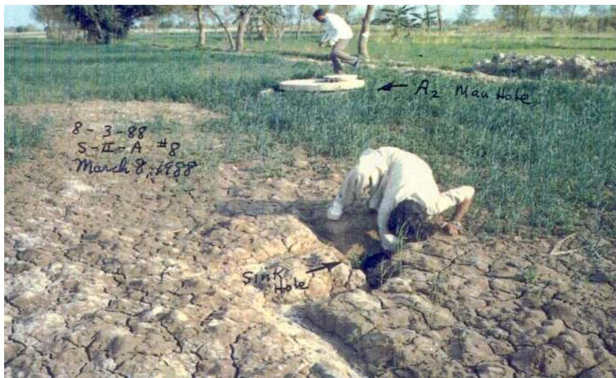
Fig.7.10 Sink Hole in Back Filled Material at FDP, Faisalabad
