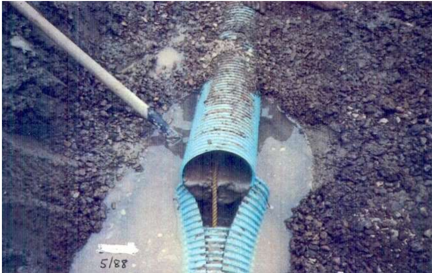
Fig. 7.11 Sediments Deposition in PVC Pipe Through sinkhole (FDP, Faisalabad)
