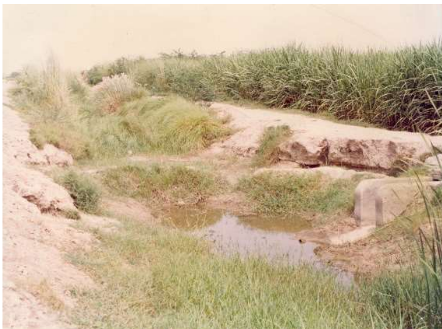
Fig.7.6a Bank erosion and vegetative growth in open drain at FDP Faisalabad
