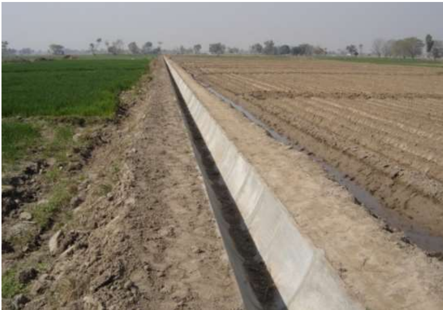
Fig.1.17 A Precast Slab Lined WC
