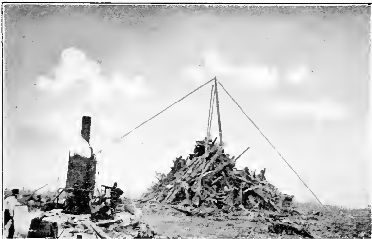
FIG. 27. SHOWING PILING STUMP FRAGMENTS BY MEANS OF A GIN POLE. A HEAVY TEAM CAN BE USED IN PLACE OF THE DONKEY ENGINE FOR LIGHT WORK
