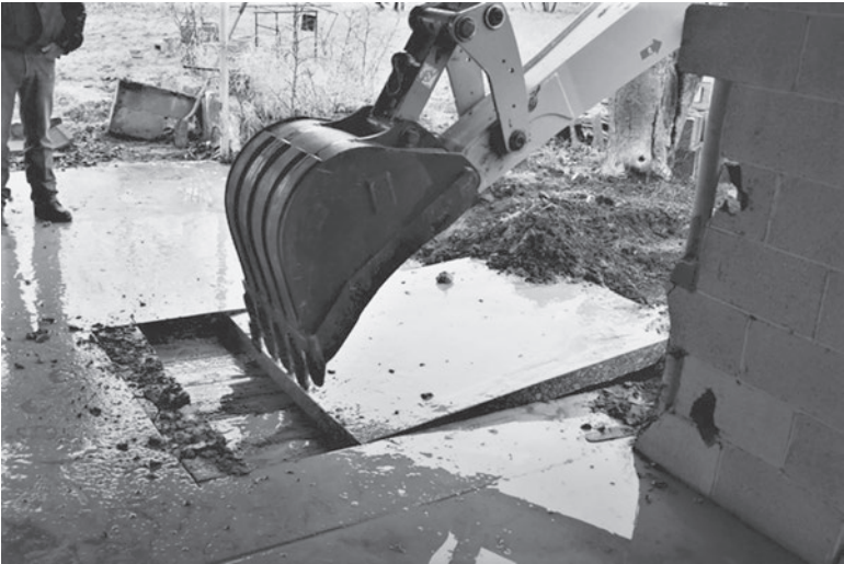
Figure 31.2 After cutting and removing a narrow strip, the backhoe can slide a large slab of concrete away from the area.
