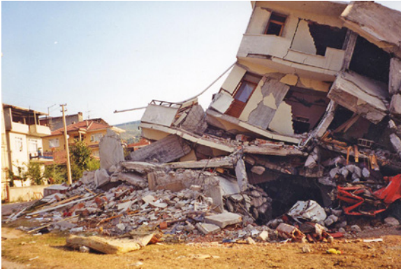
Figure 10.35 The damage in the earthquake area was huge.
