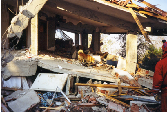
Figure 11.27 Barricaded basement. (Kaynasli, Turkey, 1999)
