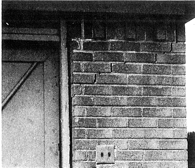
C. Separation of brick veneer from door jamb
