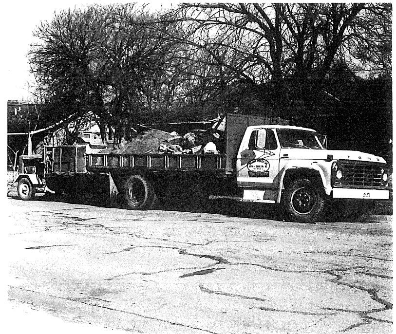
Figure 6-4. Mud-jacking equipment. The pump mixes the soil-cement with water and forces the grout through the large hose to the injection location (pre-drilled 2 inch holes).
